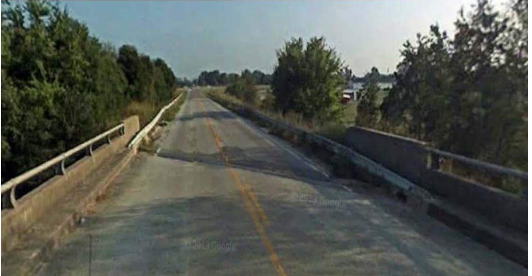
Photograph of US-31W (looking north) crossing over I-65 at approximately Sta. 295+00 (MP 78.6)
