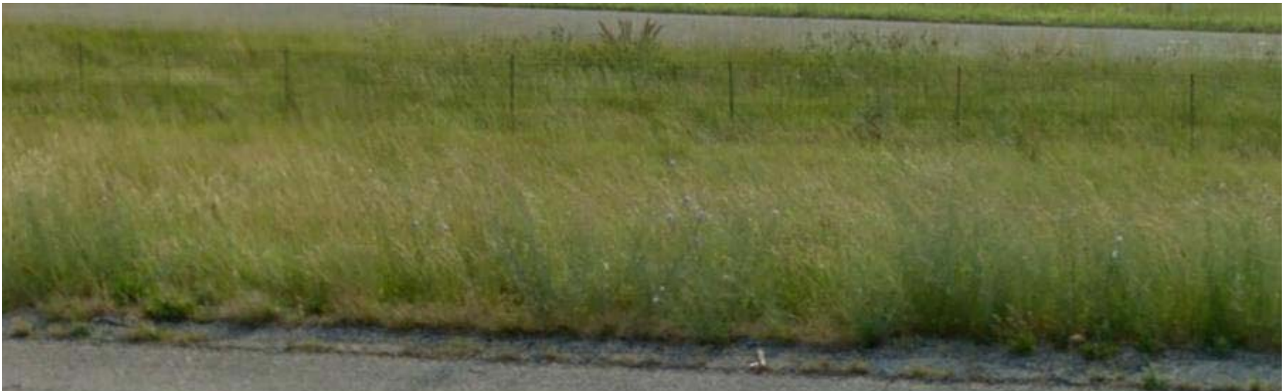
Photographs of existing ROW fencing in good condition along I-65 near the KY 224 interchange
