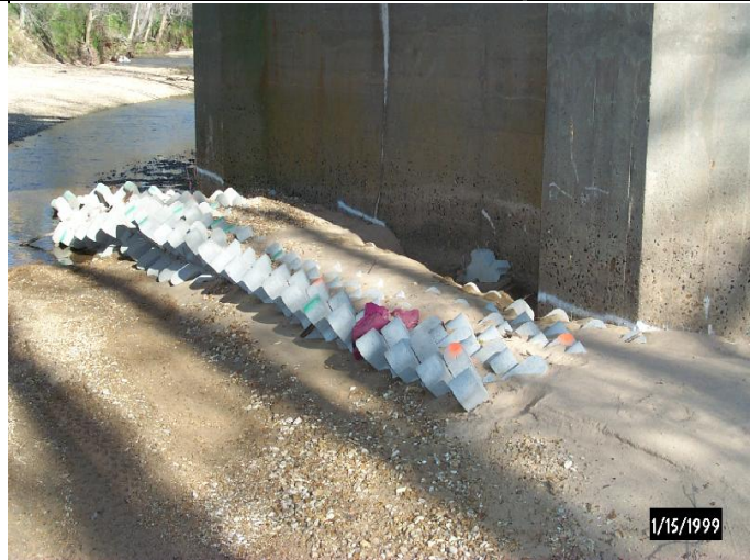
A-Jacks were used to encourage sediment deposits to fill in scour holes.
