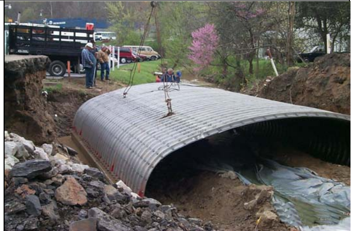
This bridge replacement includes stream isolation to minimize sediment discharge to the stream.
