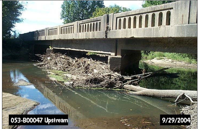
Large debris jam on bridge.
