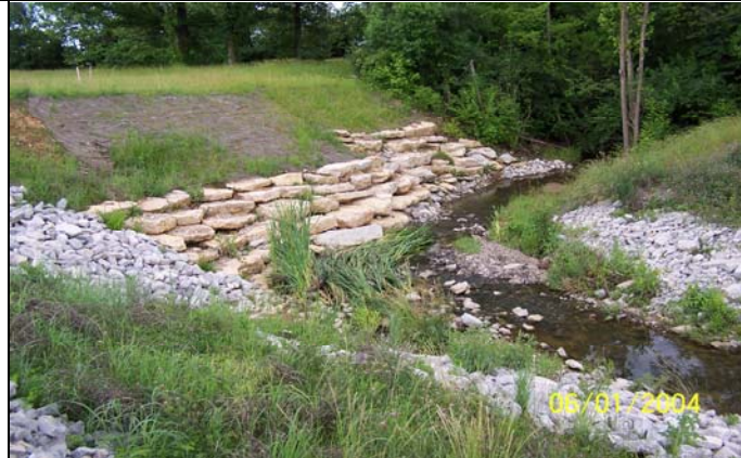
Class III channel lining, large stone and geotextile were used to prevent erosion of this steep embankment.
