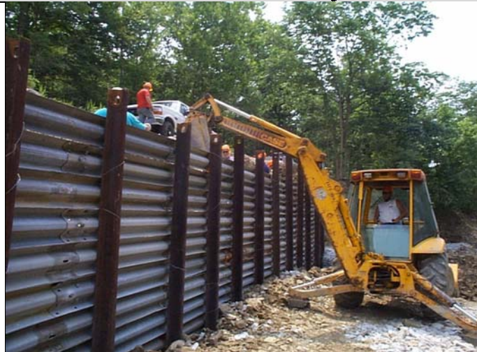
Railroad T- rails and cribs can be used to repair roadway slips adjacent to streams.
