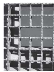
2 1/2" x 1/4" Missing Cross Bar
