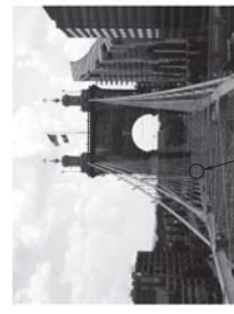
Location of Connection Plate
