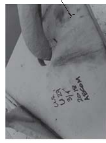
Upstream U29' Stay Cable Connection Plate
