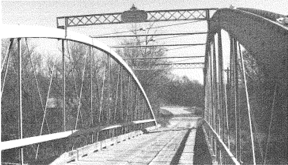
Interior view on the 148 foot long 1877 bowstring arch built by the King Iron Bridge Company next to Green Mill at Falls of Rough, Grayson County. (SF #14)
