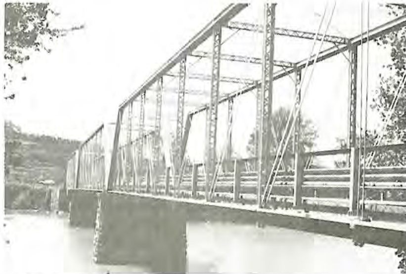
View from the bank of the Little Sandy River near its confluence with the Ohio River at Greenup. This 1884 three span Pratt through truss is by the King Bridge Company. (SF #48)
