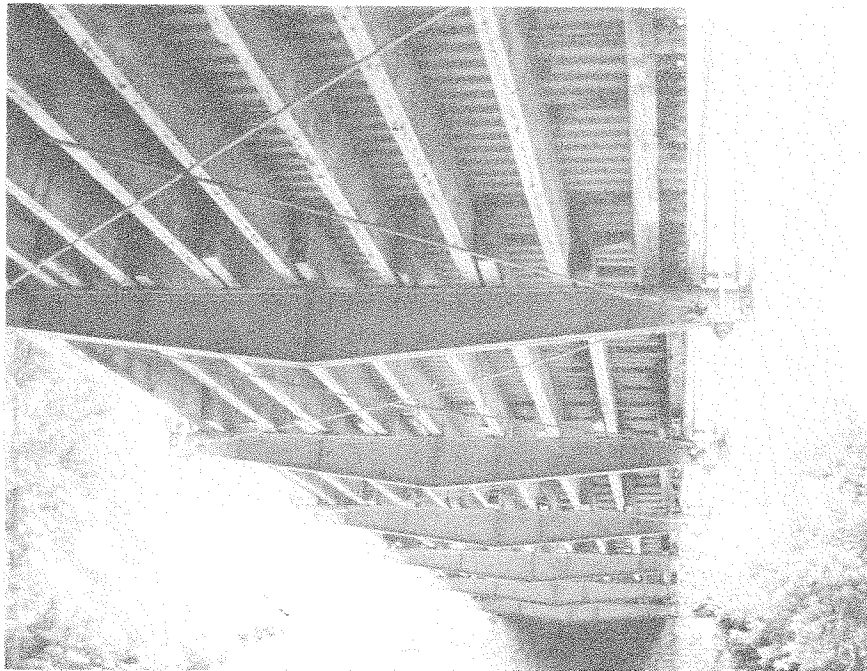
View of floor system showing corrugated metal deck, wood stringers, plate girder floor beams, and round rod bottom lateral bracing. Supports 1883 Pratt through truss by Smith Bridge Company. (SF #27)
