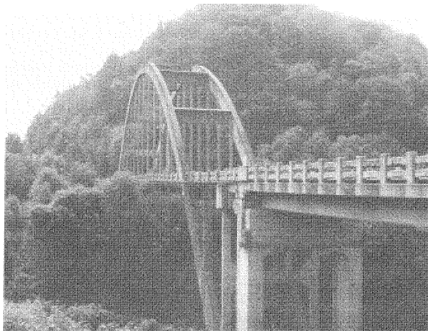
General view of the open spandrel reinforced concrete through arch bridge in Prestonsburg. This 161 foot long span is the only arch of its kind on the Kentucky highway system. (SF #64)
