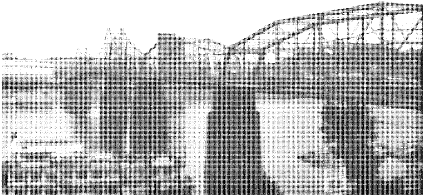
General view of the Central Bridge built by the King Iron Bridge Company in 1890 over the Ohio River between Newport and Cincinnati. The cantilever truss on the north end has a main span length of 520 feet with two 252 foot anchor spans. (SF #30)
