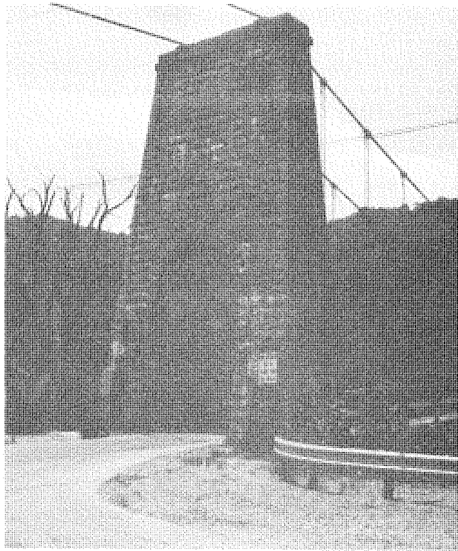
Rough cut stone tower of a 370 foot suspension bridge built by the WPA in 1938 at Pauley near Pikeville. This is one of five remaining "swinging" suspension bridges on the Kentucky highway system. (SF #70)
