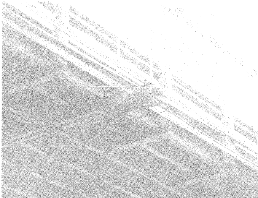
View of floor system on 1873 Warren through truss. The unusual truss floor beams are designed to be lighter and afford greater strength than solid floor beams. (SF #54)
