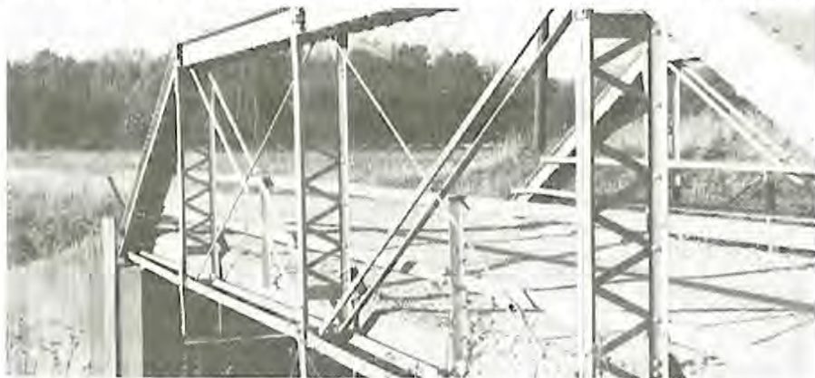
A 1923 pin-connected Pratt pony truss built by the Vincennes Bridge Company of Vincennes, Indiana. Note compression members are paired angles/lacing bars and tension members are two eyebar diagonals. Counters are one round rod eyebar with turnbuckles for field adjustment. (SF #6)
