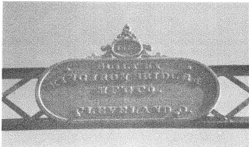
Earliest builder/date plate on a metal truss bridge in Kentucky. The King Iron Bridge Company was established by Zenas King in 1858. (SF #14)
