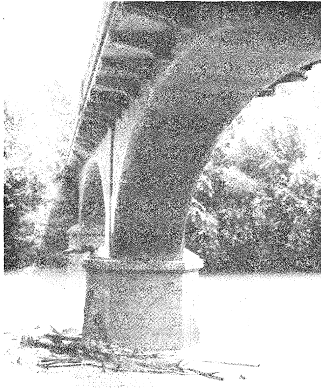
Concrete arch deck bridge with three spans and stone piers built in 1925 by the Luten Bridge Company of York, Pennsylvania. (SF #59)
