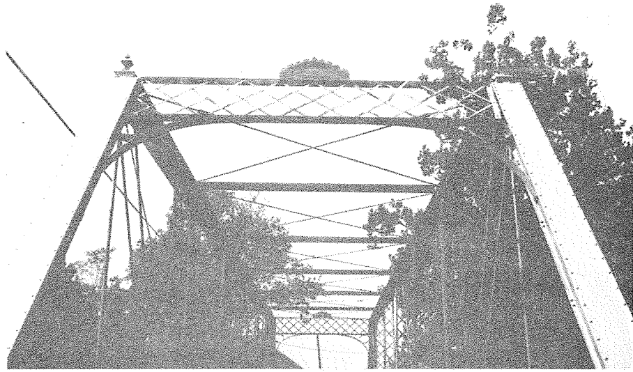
Plate on portal strut identifies the Champion Bridge Company of Wilmington, Ohio, as the builder but does not give the erection date. This unique builder plate and decorative finials are found on only one other Champion bridge in Kentucky. (SF #37)
