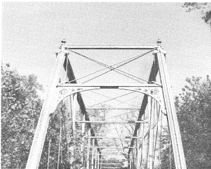
View of Phoenix column end posts, cut-out portal bracing, and finials on a Whipple-Murphy truss in eastern Kentucky. (SF #49)
