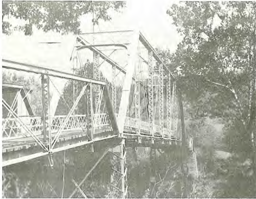
This 3/4 view shows a pin-connected Pratt through truss center span and two pin connected Pratt half-hip end spans resting on unique piers built of steel sections. (SF #52)
