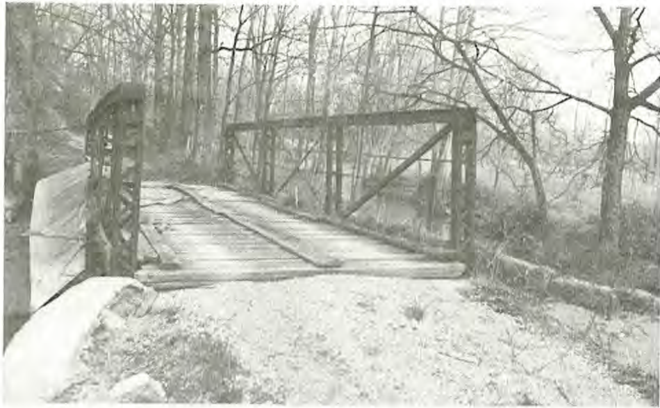
General view of 1905 Brackett Bridge Company bedpost pony truss with end posts that extend below the deck of the bridge. (SF #9)
