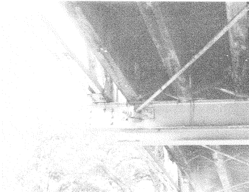
Detail floor system view showing rolled I-beam floor beam with wood stringers on top. Note round rod bottom lateral bracing passing through and bolted to the floor beam flange. (SF #26)
