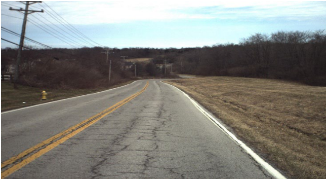
PATTERN CRACKING = POOR
