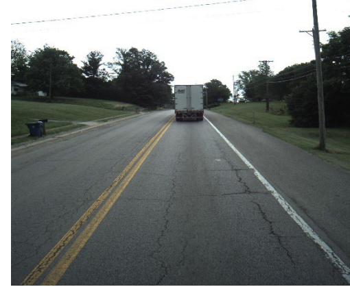
Longitudinal Cracking = Poor
