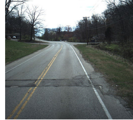
UTILITY CUTS = POOR
