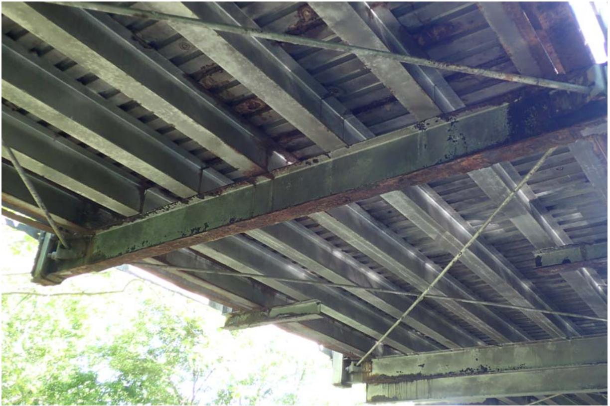
View of the floorbeam at L2. Notice that the retrofitted floorbeam that was welded to the bottom flange of the original floorbeam has fallen off. Note the floorbeam at L1.
