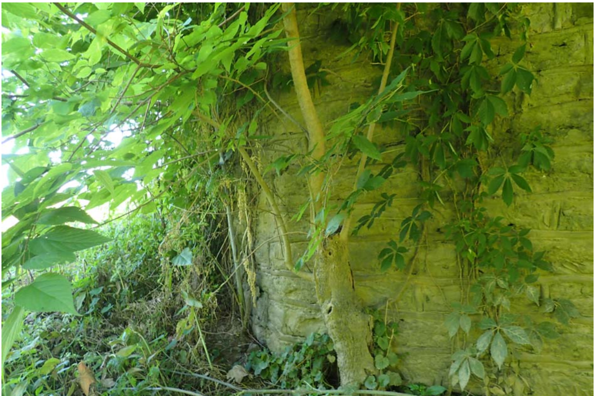
View of heavy vegetation growth at the downstream end of the east abutment.
