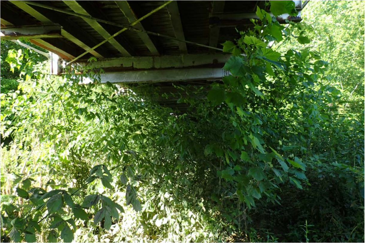
View of heavy vegetation growth at the east end of the bridge.
