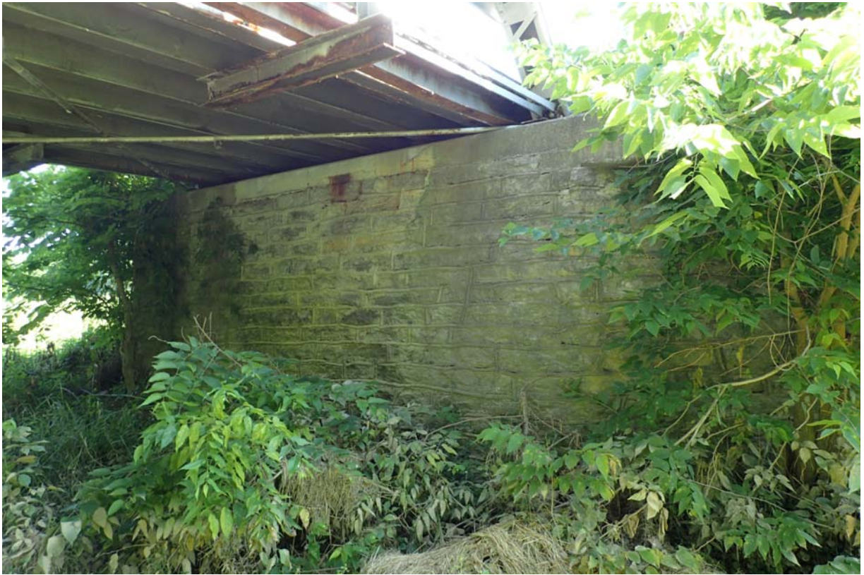
Typical view of the east abutment. Notice the minor sized horizontal cracking in the concrete cap.
