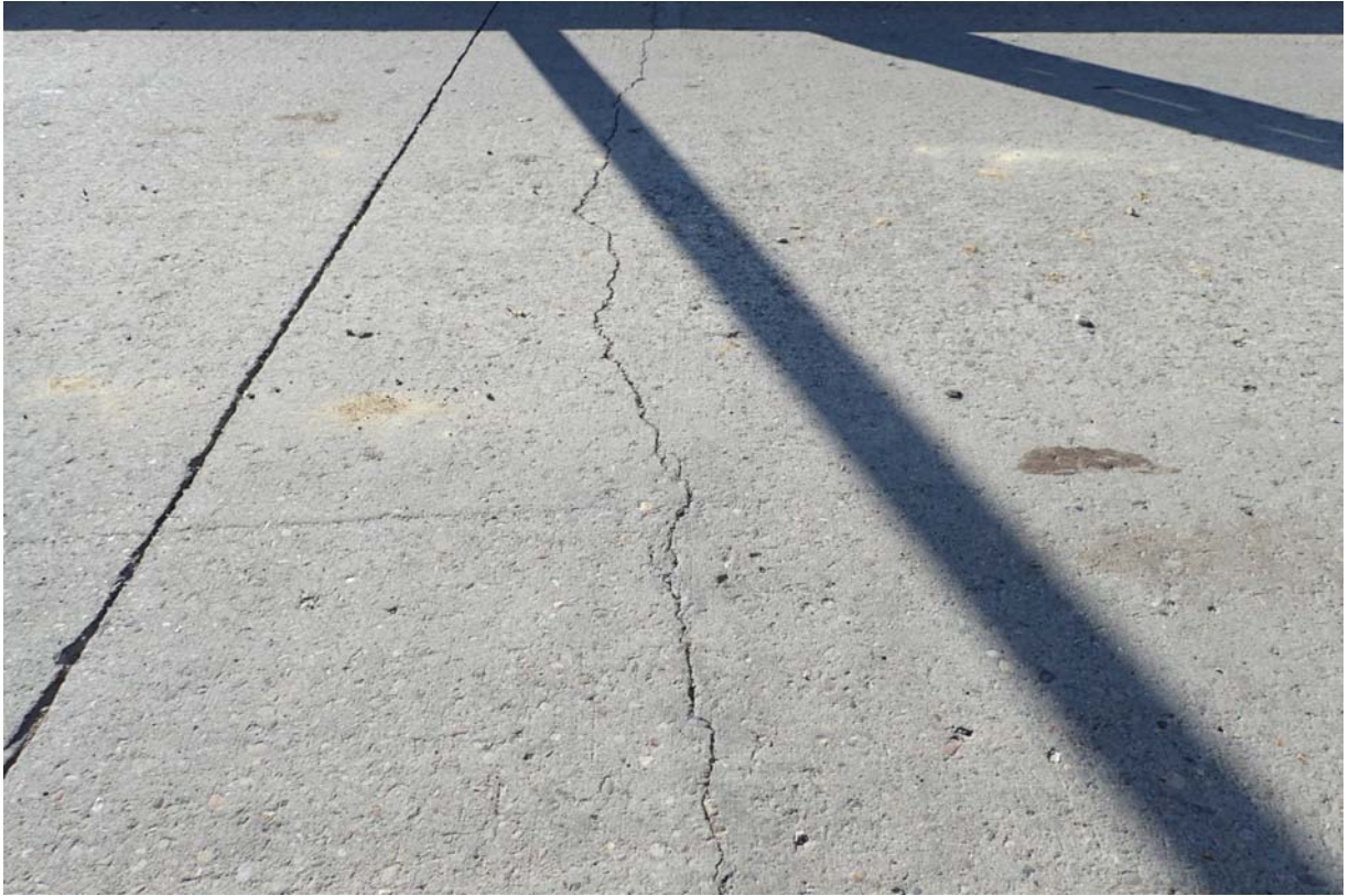
View of a more moderate sized (~1/16") full width transverse crack in the wearing surface near the L6 connection.
