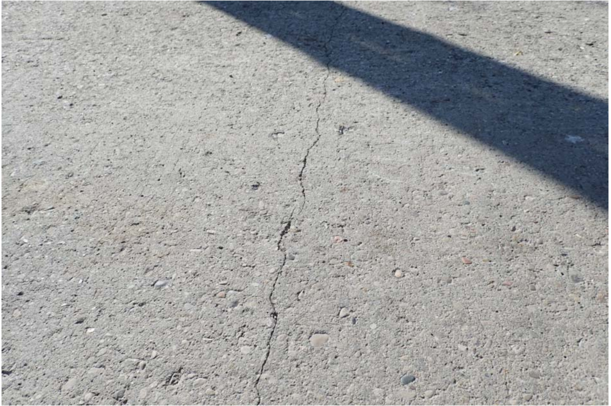
View of a minor sized full width transverse crack in the wearing surface between the L4 and L5 connections.
