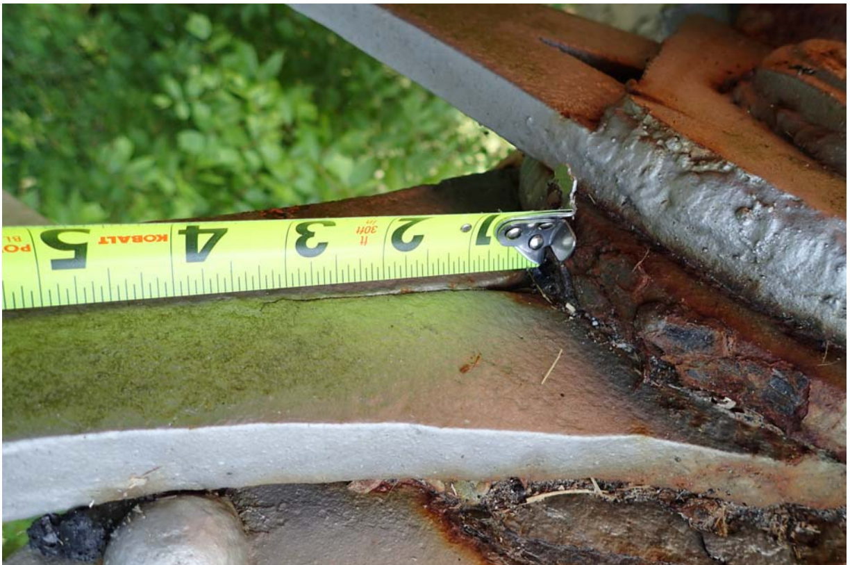
View of ~ 3.25" measured along the forge in the interior eyebar at the upstream L2 connection. There is a retrofit at this location.
