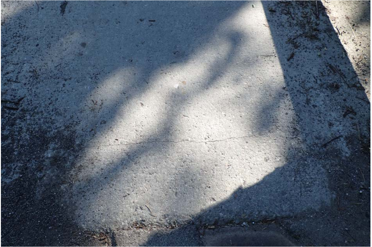
View of minor sized transverse cracking in the wearing surface near the west abutment.
