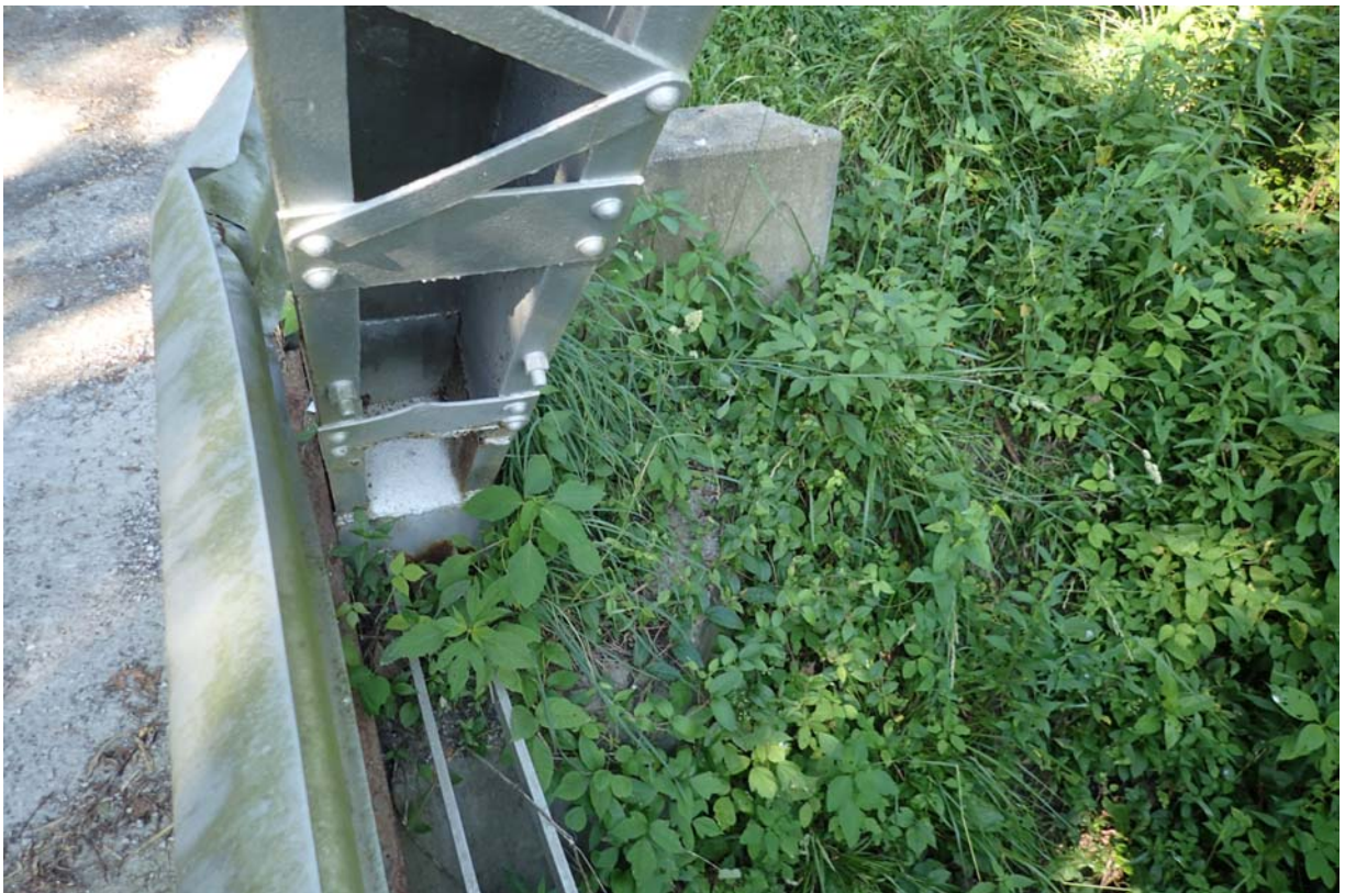
View of heavy vegetation growth at the east abutments downstream bearing.
