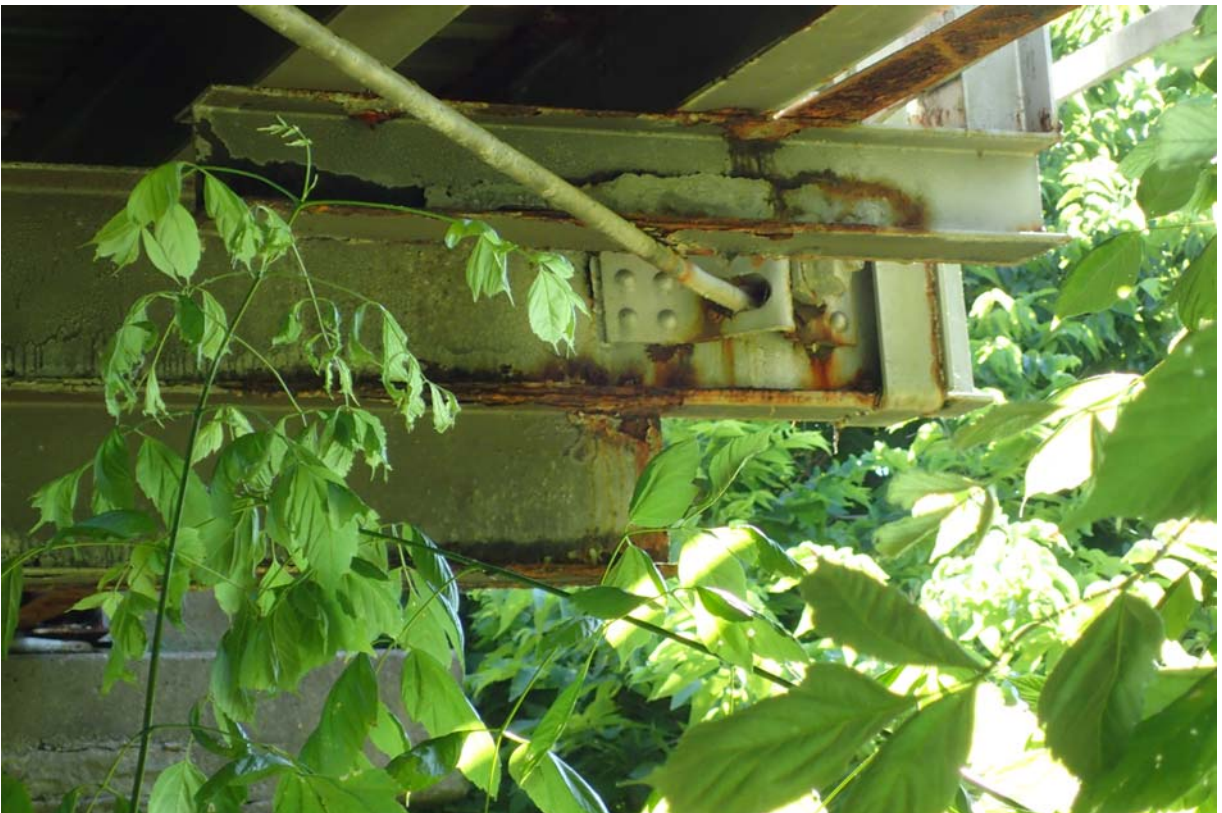
Typical view of heavy corrosion at the upstream end of the floorbeam at L7.
