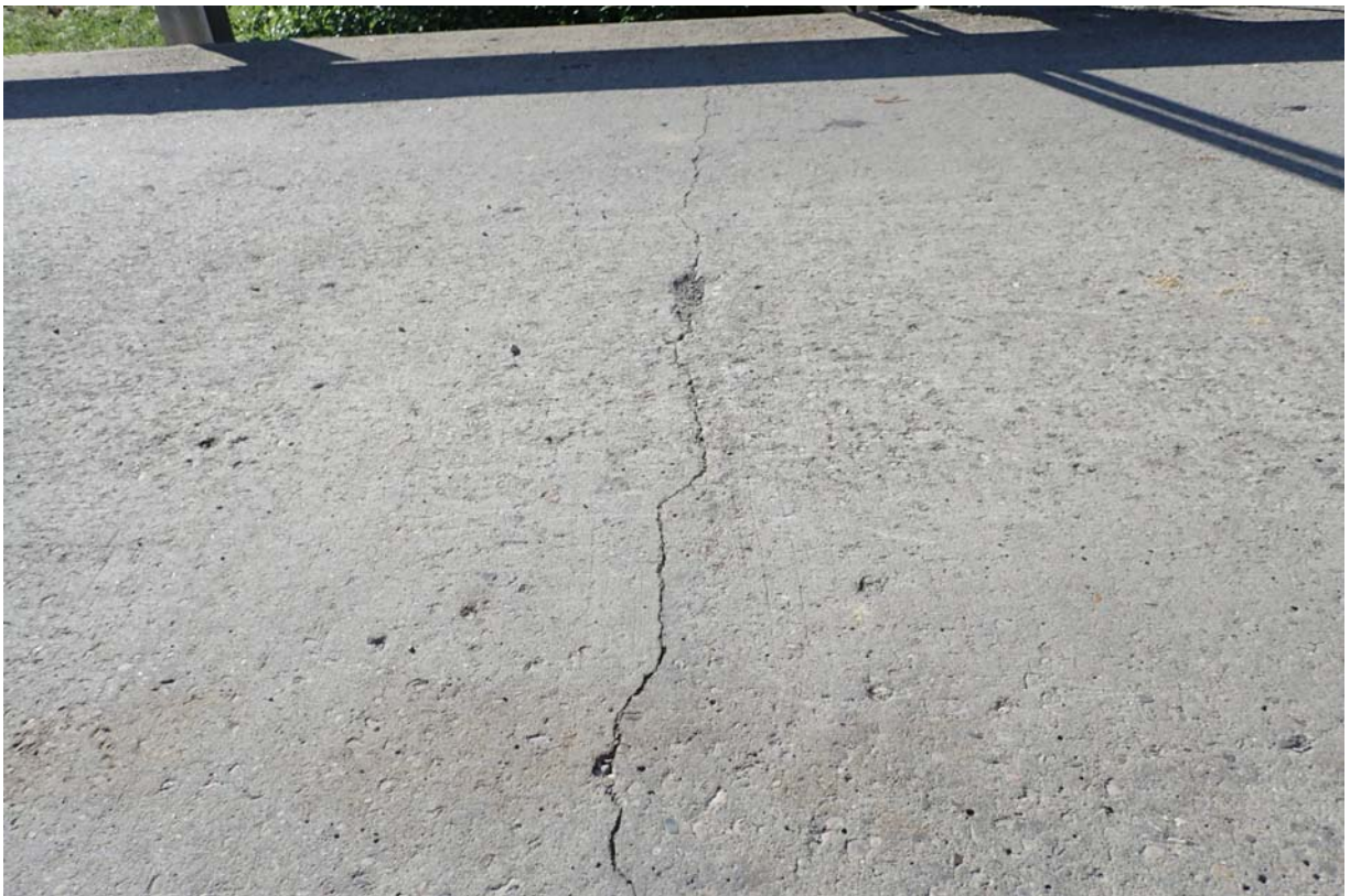
View of a more moderate sized (~1/16") full width transverse crack in the wearing surface near the L5 connection.
