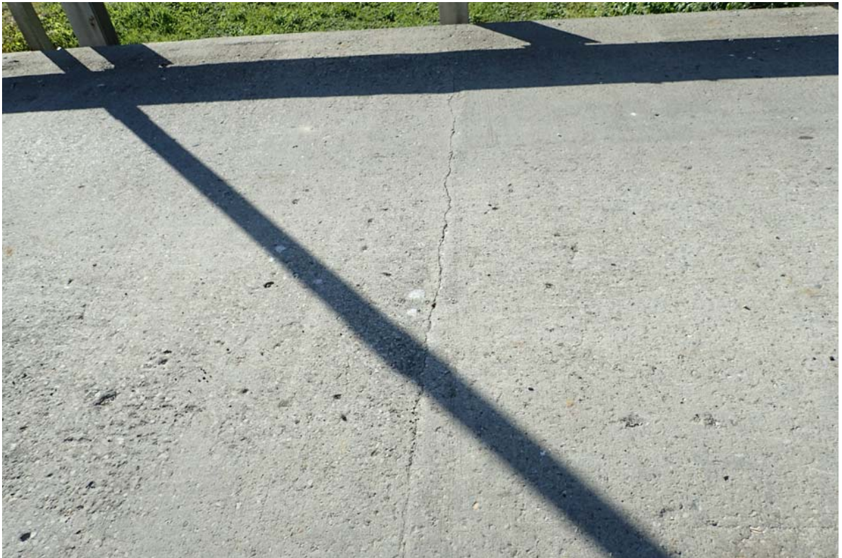
View of a minor sized full width transverse crack in the wearing surface between the L6 and L7 connections.
