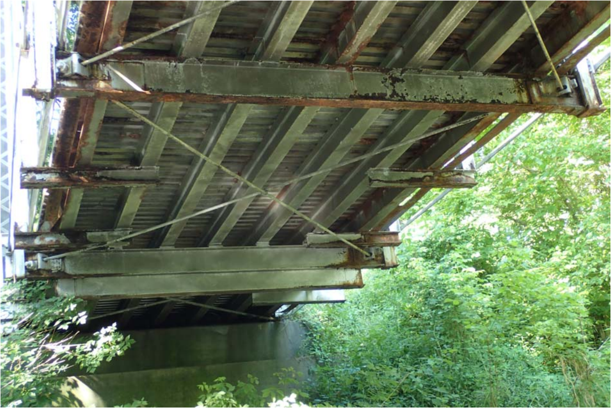
View of the floorbeam at L2. Notice that the retrofitted floorbeam that was welded to the bottom flange of the original floorbeam has fallen off. Note the floorbeam at L1.
