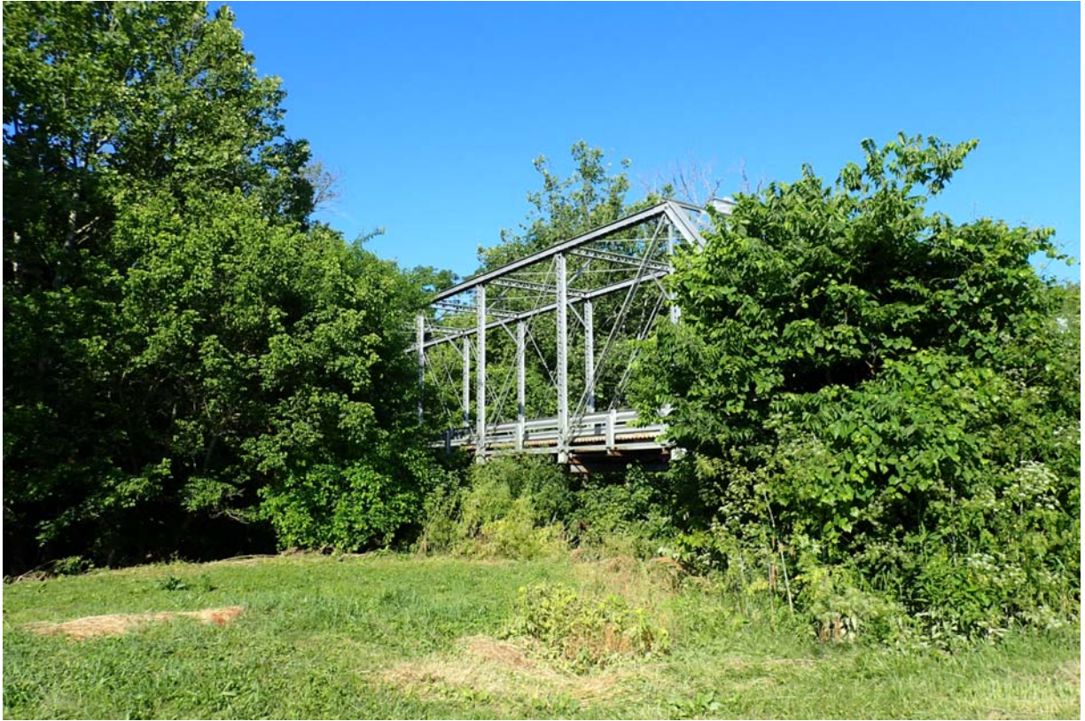
View from the upstream east end of the bridge. Notice the heavy vegetation growth.
