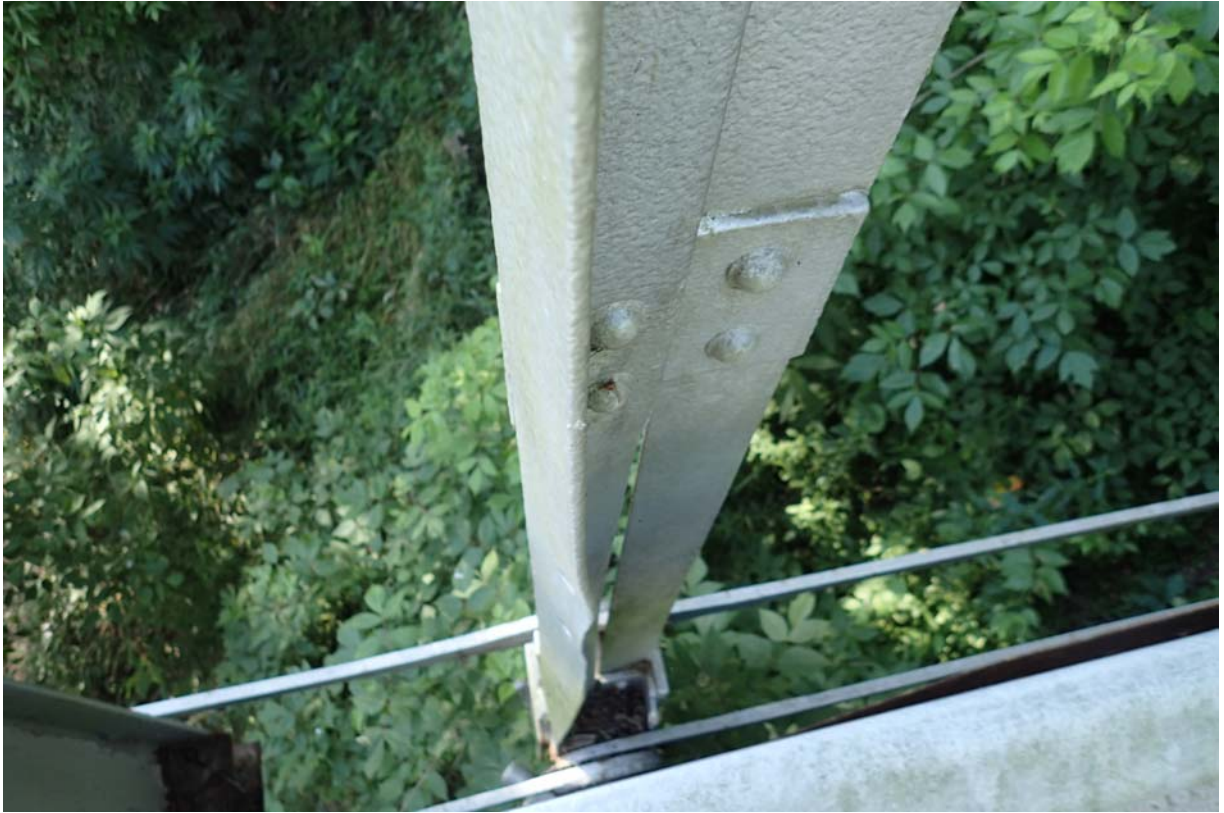
View of a bend in the lower section of the upstream L1 vertical.
