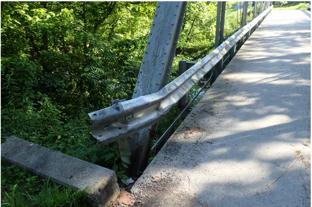
View of moderate impact damage to the downstream rail at the west abutment.
