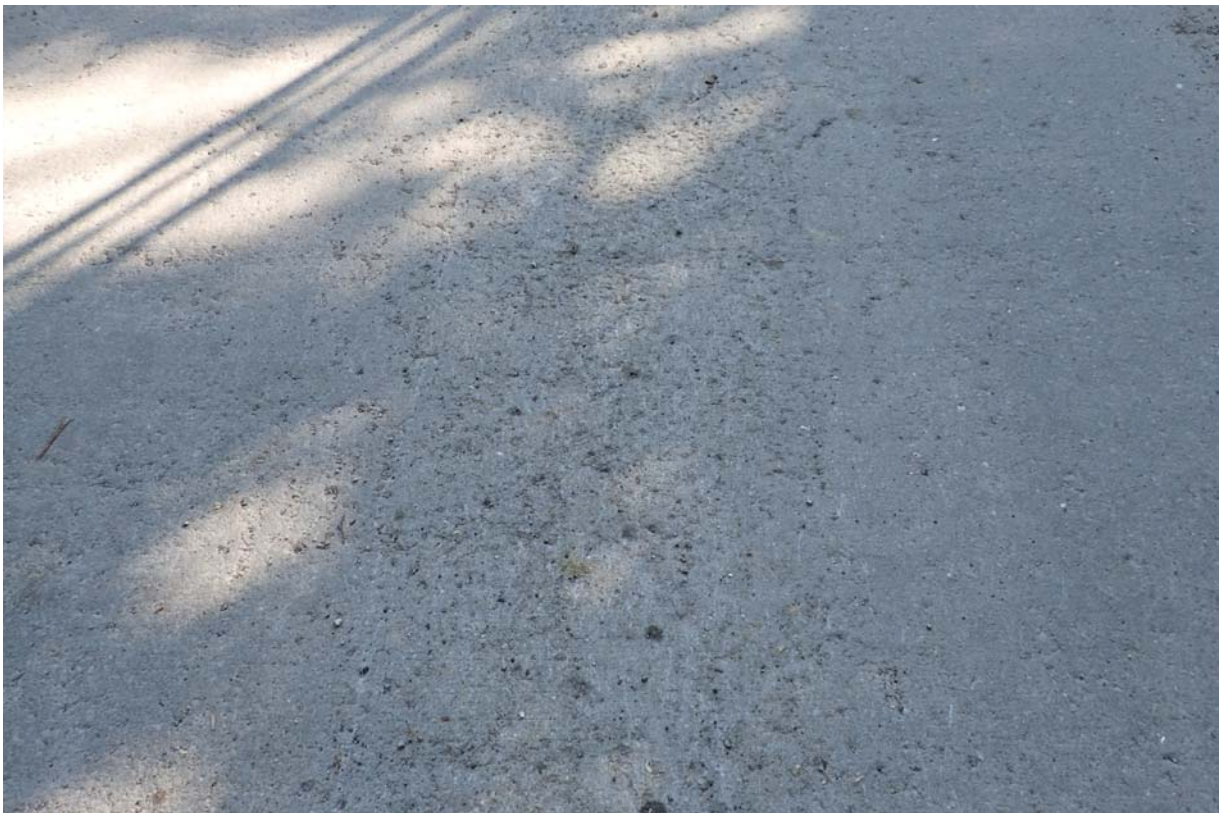
The wearing surface is rough along the centerline of the bridge. This is in Amish country and the bridge sees alot of horseshoes.
