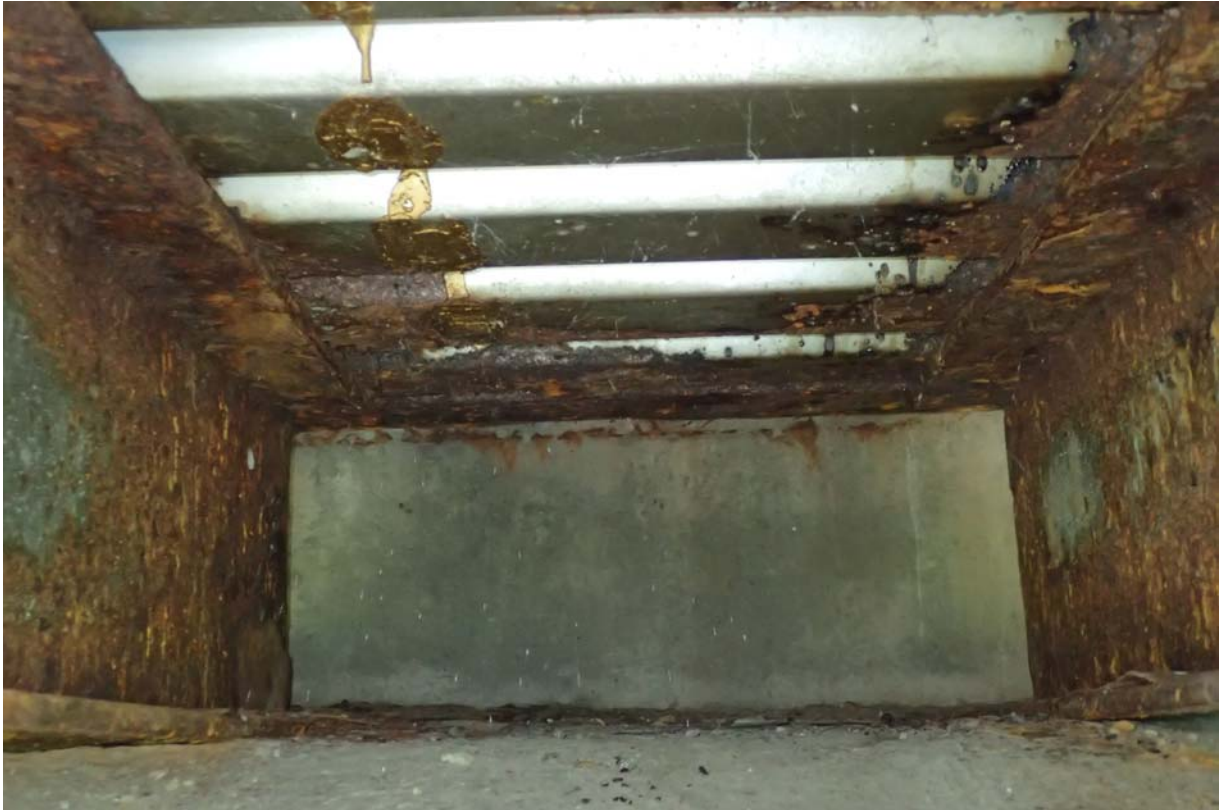
Typical view of moderate to heavy corrosion of the stringer ends at the west abutment.
