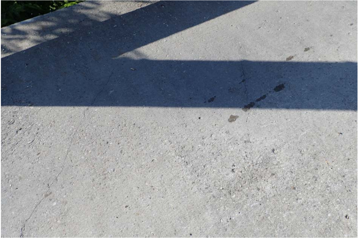
View of 2 minor (there is actually 3, one is not visible in photo) sized diagonal trending cracks in the wearing surface between the L7 and L8 connections
