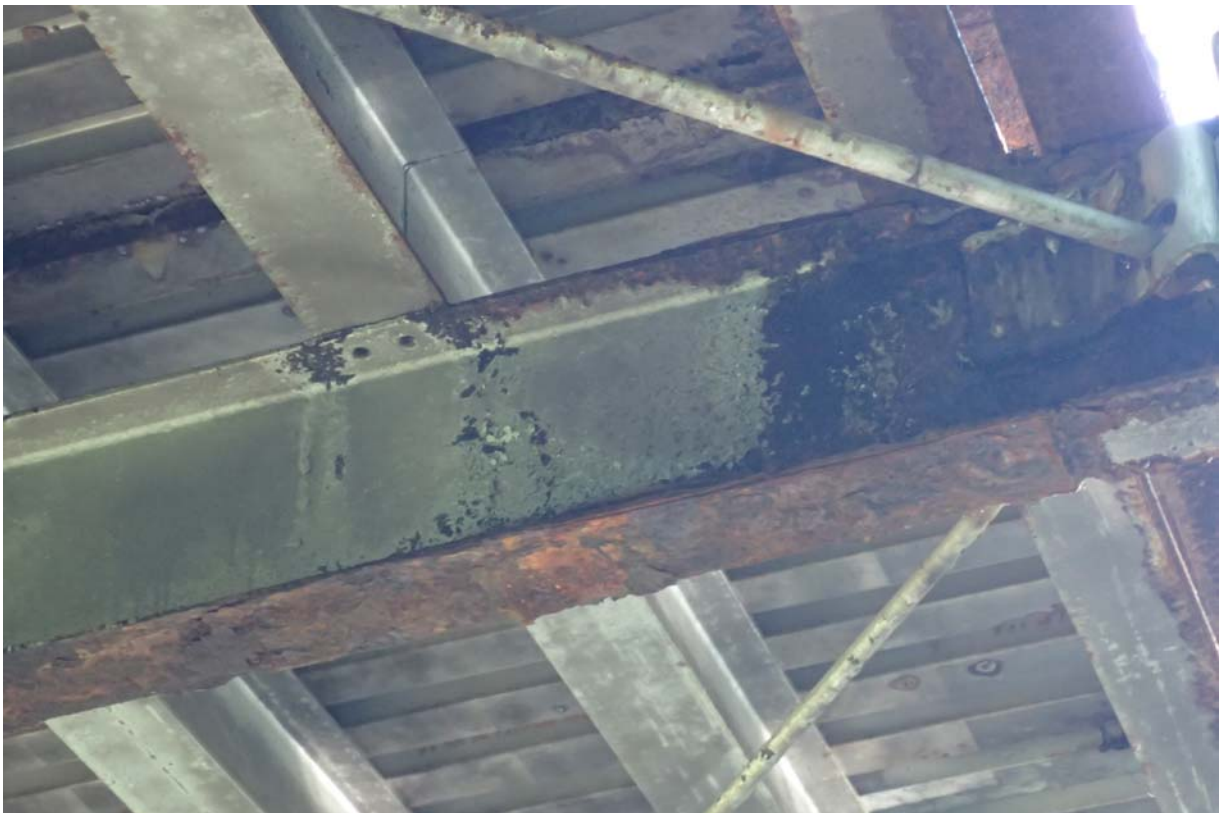
View of the floorbeam near the upstream L2 connection. Notice that the retrofitted floorbeam that was welded to the bottom flange of the original floorbeam has fallen off. Note the heavy corrosion.
