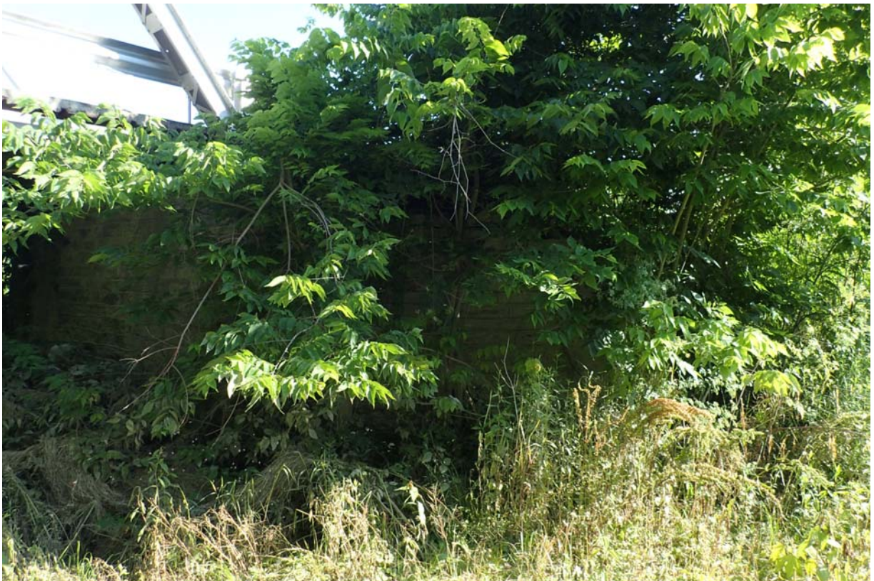
View of heavy vegetation growth at the upstream end of the east abutment.
