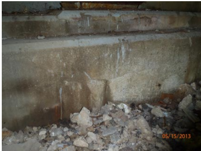
View of light cracking in abutment 4's breast wall below bearing 3 from the south.
