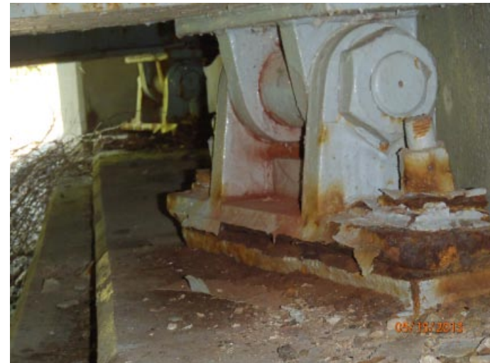
View of bearings 3 and 4 from the south. They are rocked back toward the backwall.
