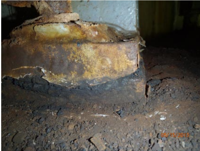
View of the rocker of bearing 2 from the south. The rocker is slightly behind the front edge of the masonry plate.
