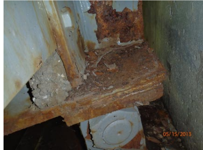
View of moderate rusting and corrosion at the end of beam 2 from the south at abutment 4.
