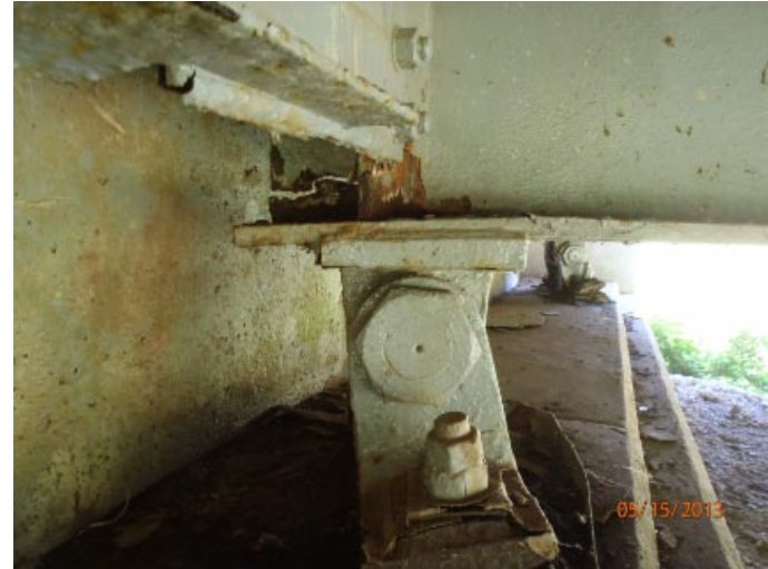
View of beam 3 from the south at abutment 1. Notice the bottom flange bending downward toward the backwall.
