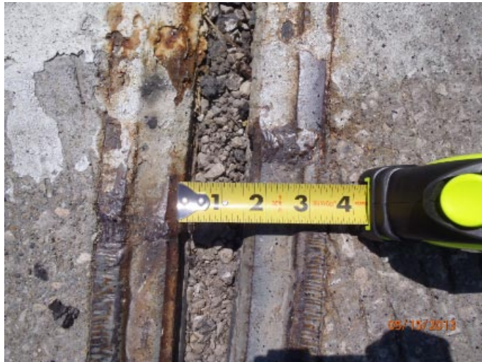
View of a 1.5" measurement taken at the expansion joint at abutment 1 at the roadway centerline.
