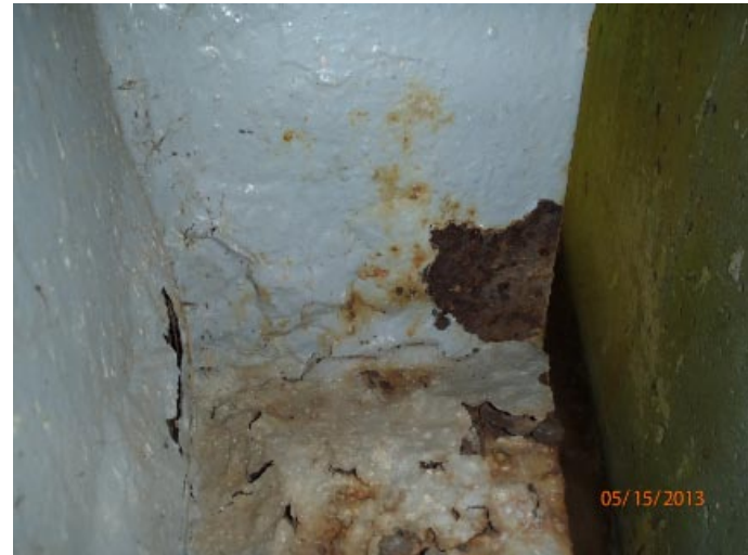
View of moderate pitting in the lower web of the north beam behind the bearing at abutment 1.
