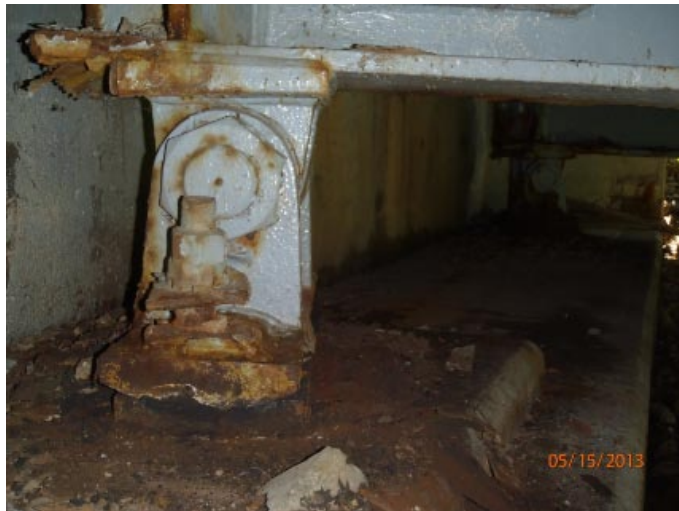
View of bearings 1 and 2 from the south at abutment 4. Bearing 1 is rocked back toward the backwall and bearing 2 is almost straight.
