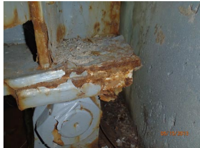
View of moderate rusting and corrosion at the end of the bottom flange of the north beam at abutment 4.
