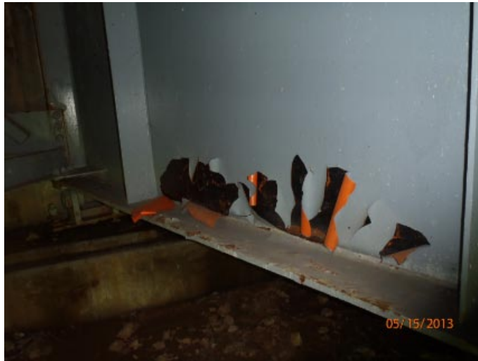
View of flaking paint along the north face of beam 3's web.
