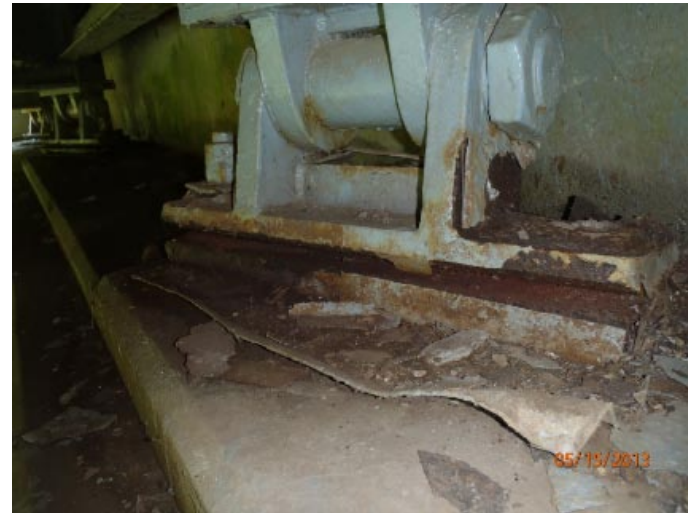
View of bearing 3 at abutment 1. Notice the north anchor bolt is missing.
