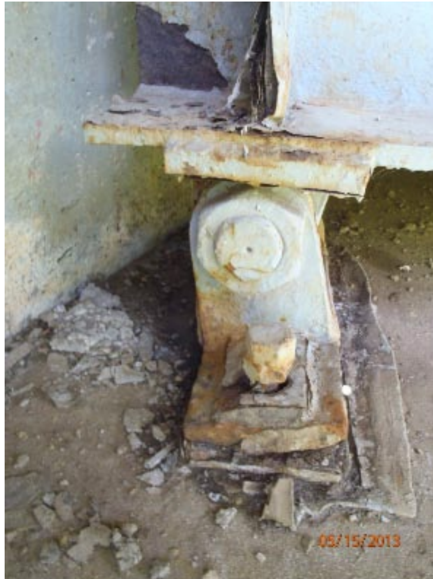
View of the south bearing at abutment 1. Notice the pack rust at the bottom of the vertical stiffener.
