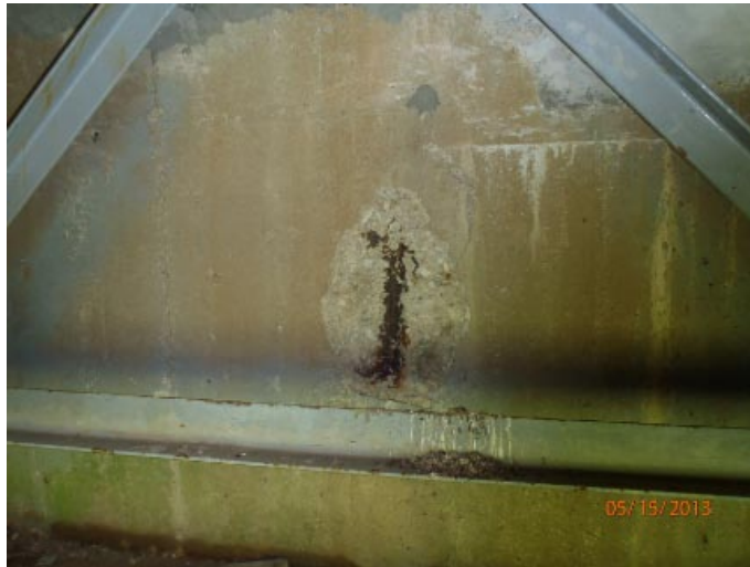
View of a moderate sized shallow spall with exposed steel in the backwall of abutment 1 between beams 3 and 4 from the south.
