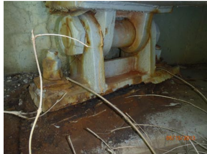
View of the north bearing at abutment 4. It has flaking paint and moderate corrosion of the masonry plate.
