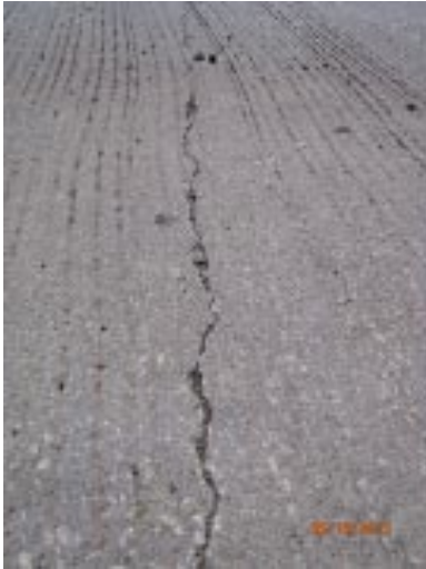
View of transverse cracking that is beginning to open up in the right lane near midspan in span 2.
