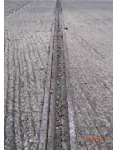
View of the transverse joint at abutment 4. It is partially full of dirt and debris.
