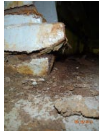
View of the rocker of bearing 3 extending approximately 1" beyond the front edge of the masonry plate.
