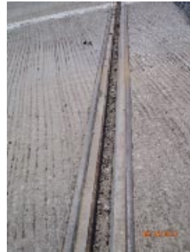
View of the expansion joint at abutment 1. It is partially full of dirt and debris.
