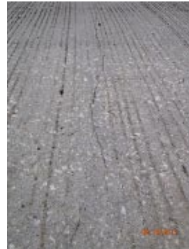
View of light transverse cracking in the right lane in span 2.
