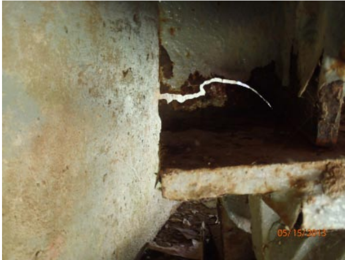
View of the previously noted crack in the web of beam 3 from the south at abutment 1. This crack is at the end of the web and stops at the bottom of the vertical stiffener.
