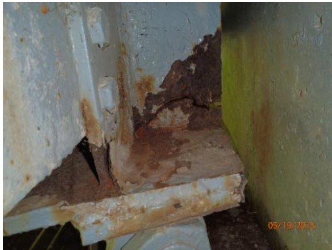
View of the previously noted crack in the web of beam 3 from the south at abutment 1. This crack is at the end of the web and stops at the bottom of the vertical stiffener.
