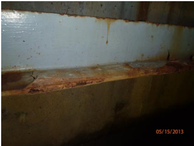
View of some moderate rusting and corrosion of the steel diaphragm between beams 1 and 2 from the south at abutment 4.
