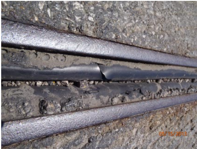
View of a small tear in the seal at the center of the left lane at abutment 4.
