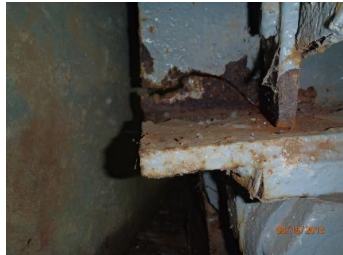
View of the previously noted crack in the web of beam 3 from the south at abutment 1. This crack is at the end of the web and stops at the bottom of the vertical stiffener.
