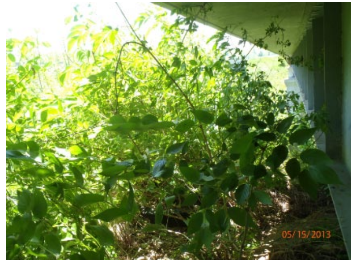
View of vegetation growth at the south end of span 3.
