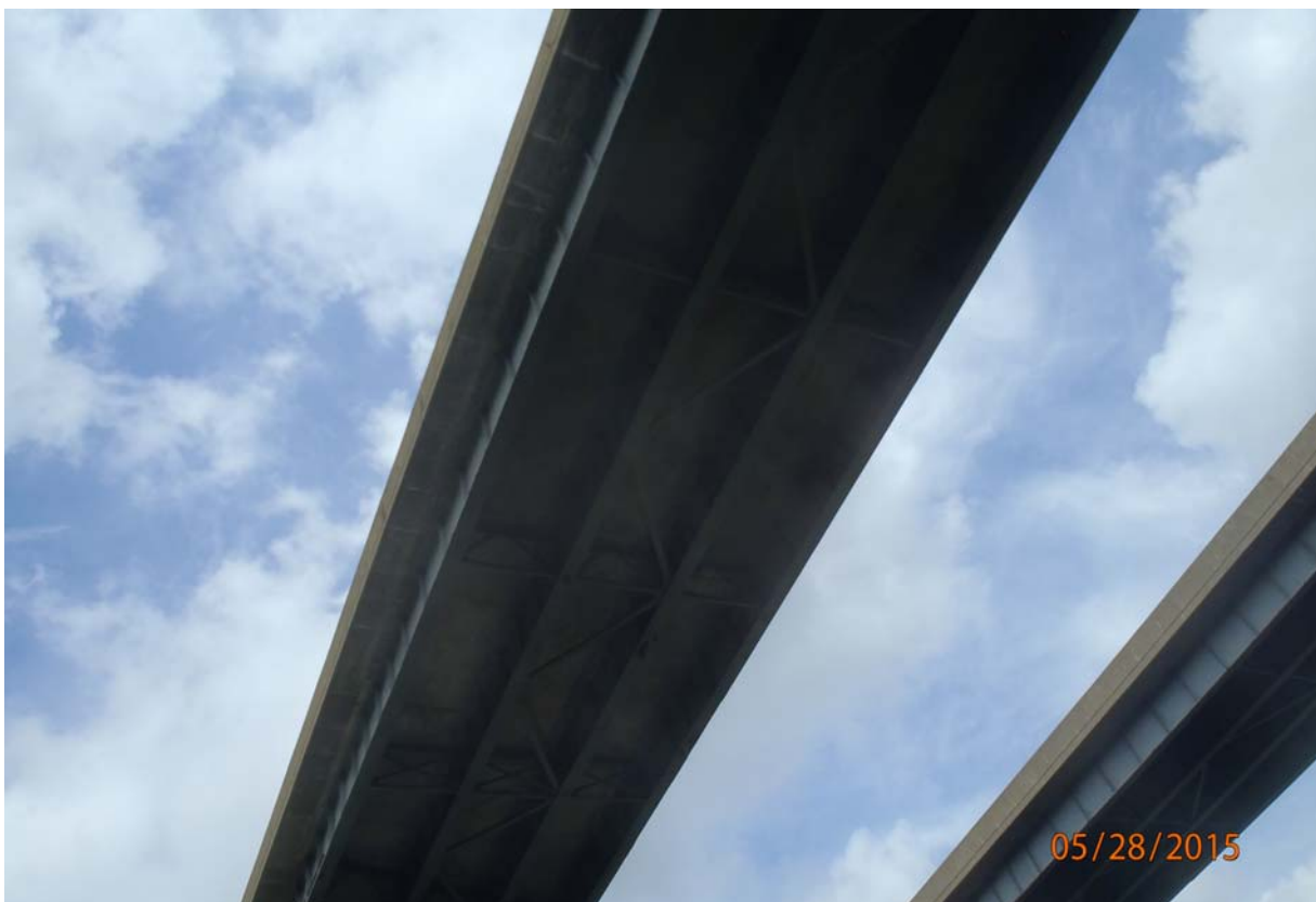
View of the underside of span 3. Note the transverse cracks with efflorescence on the underside of the downstream overhang.
