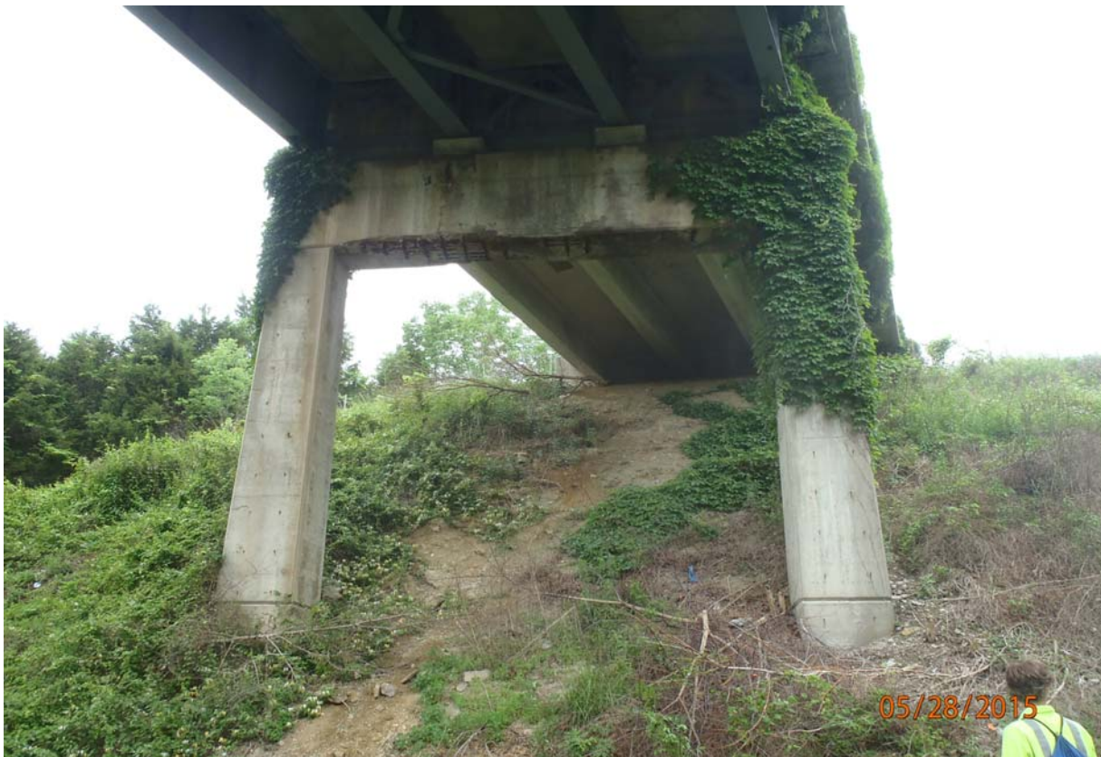
Elevation view of the east face of pier 2. Note the exposed rusting/corroding reinforcing steel in the pier and heavy rust staining on the pier cap see below photo for more info. Note 1 area with exposed rusting/corroding exposed vertical reinforcing steel in the east face of the cap (under beam 3 bearing). This pier cap needs to be cleaned and patched.
