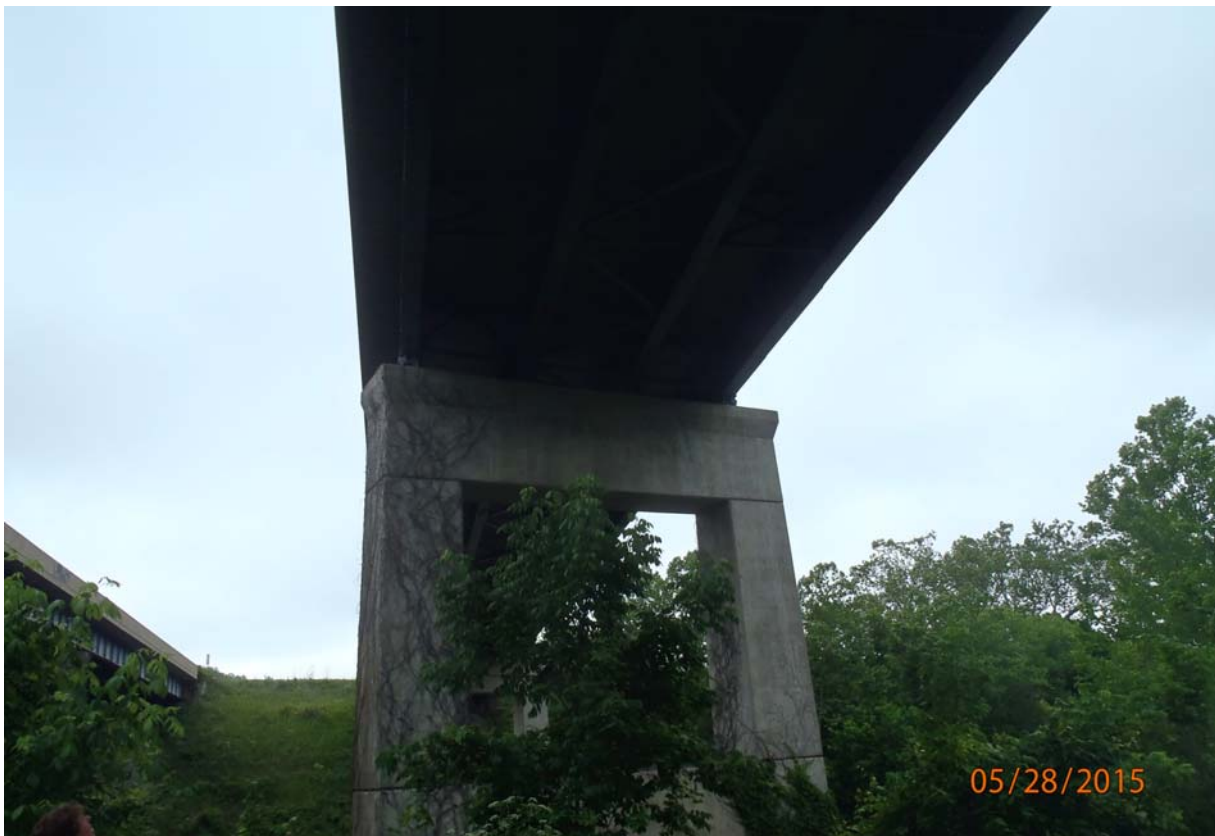
Elevation view of the west face of pier 3. Note the vegetation growth.
