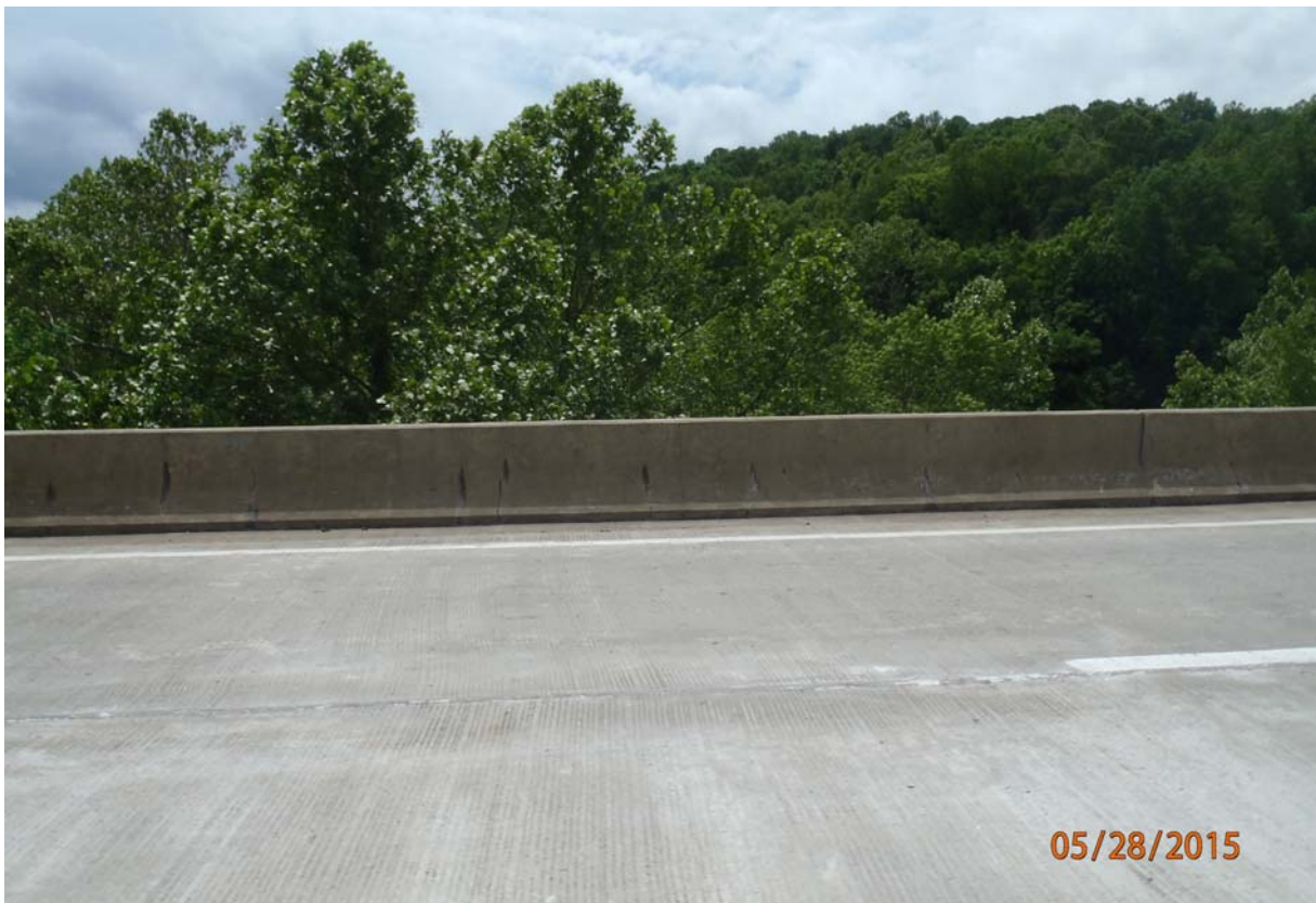
View of the downstream barrier wall. Note minor vertical cracking in the face of the barrier wall along the entire length of wall and many areas of scaling of the masonry coating on the face of the barrier wall.
