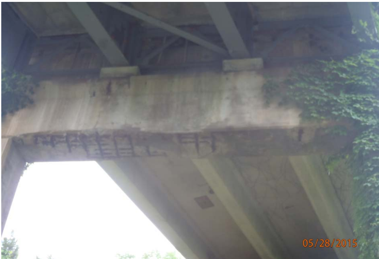
Looking up at the underside of the pier cap of pier 1. Note the heavily rusted and corroding (w/ section loss) exposed reinforcing steel. There is a deck joint directly above this pier (between the steel girder span and reinforced concrete girder span). The plans called for 2 rows of 6 #11 Bar. 4/19
