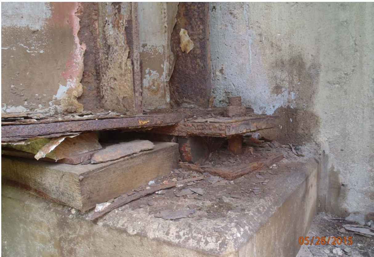
View of the bearing and beam end of beam 3 @ abutment 5. Note the heavy active corrosion and section loss at this location.
