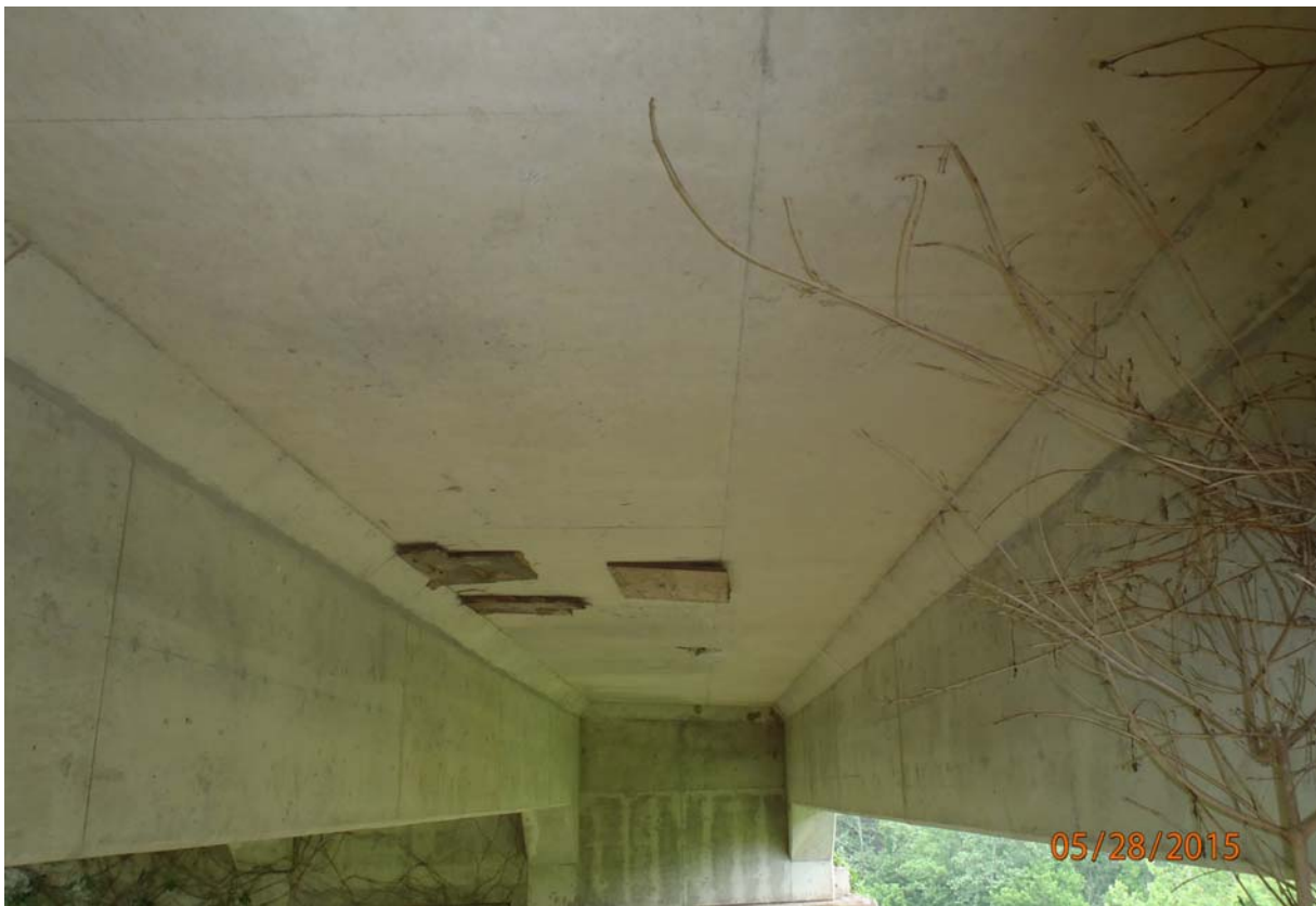
Looking up at the underside of the deck in span 1 between beams 3 & 4. Note the plywood forms still in place, minor vertical cracking in the concrete beams, minor map cracking on the underside of the bridge deck near abutment 1 and light scaling of concrete on the deck underside.
