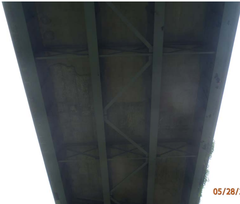
Looking up at the underside of span 2. Note the transverse cracks with efflorescence on the deck underside throughout the span; these cracks are more dominant near mid-span; there is evidence of water staining near mid-span on the deck underside. Note the areas of patching on the deck underside.
