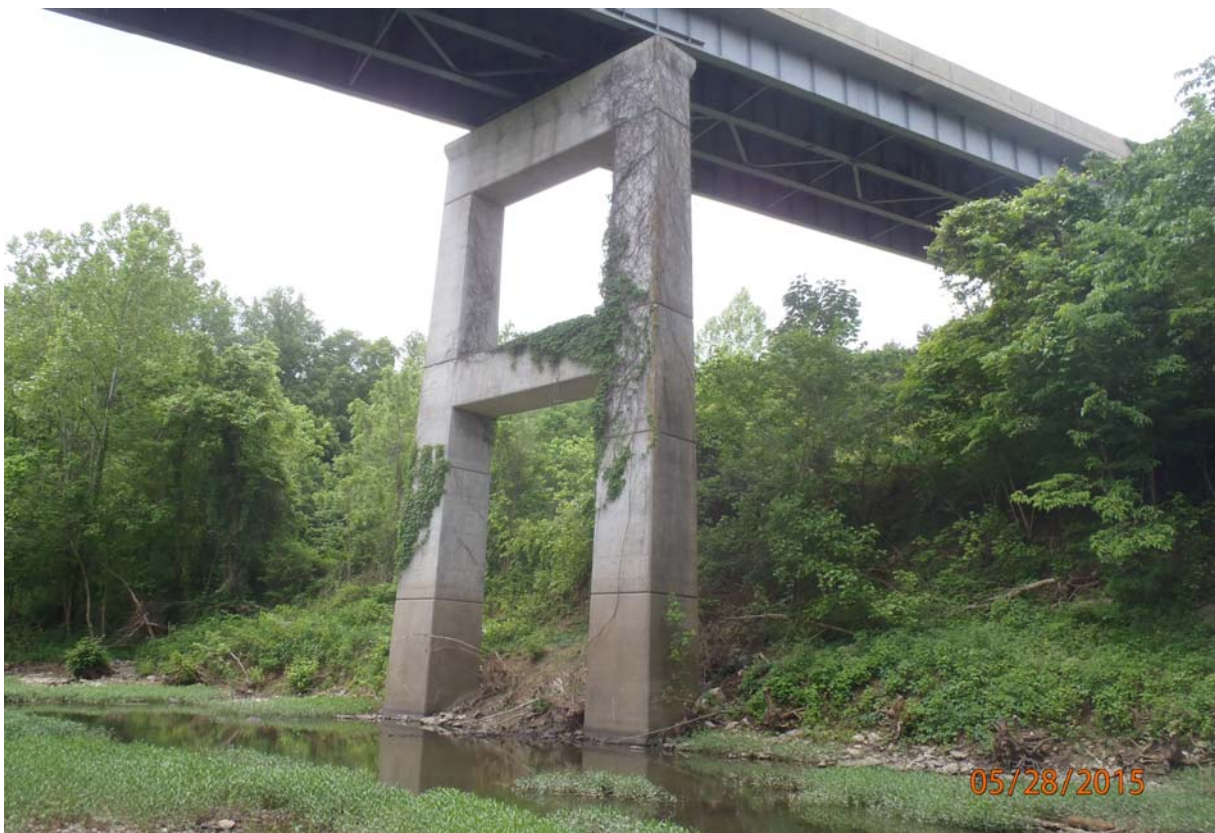
Elevation view of pier 3. Note the heavy vegetation growth.
