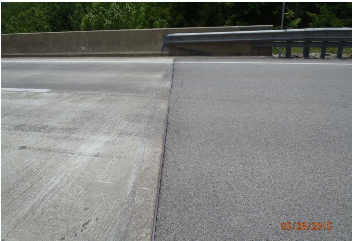
Transition between the west roadway approach and west end of the bridge deck.
