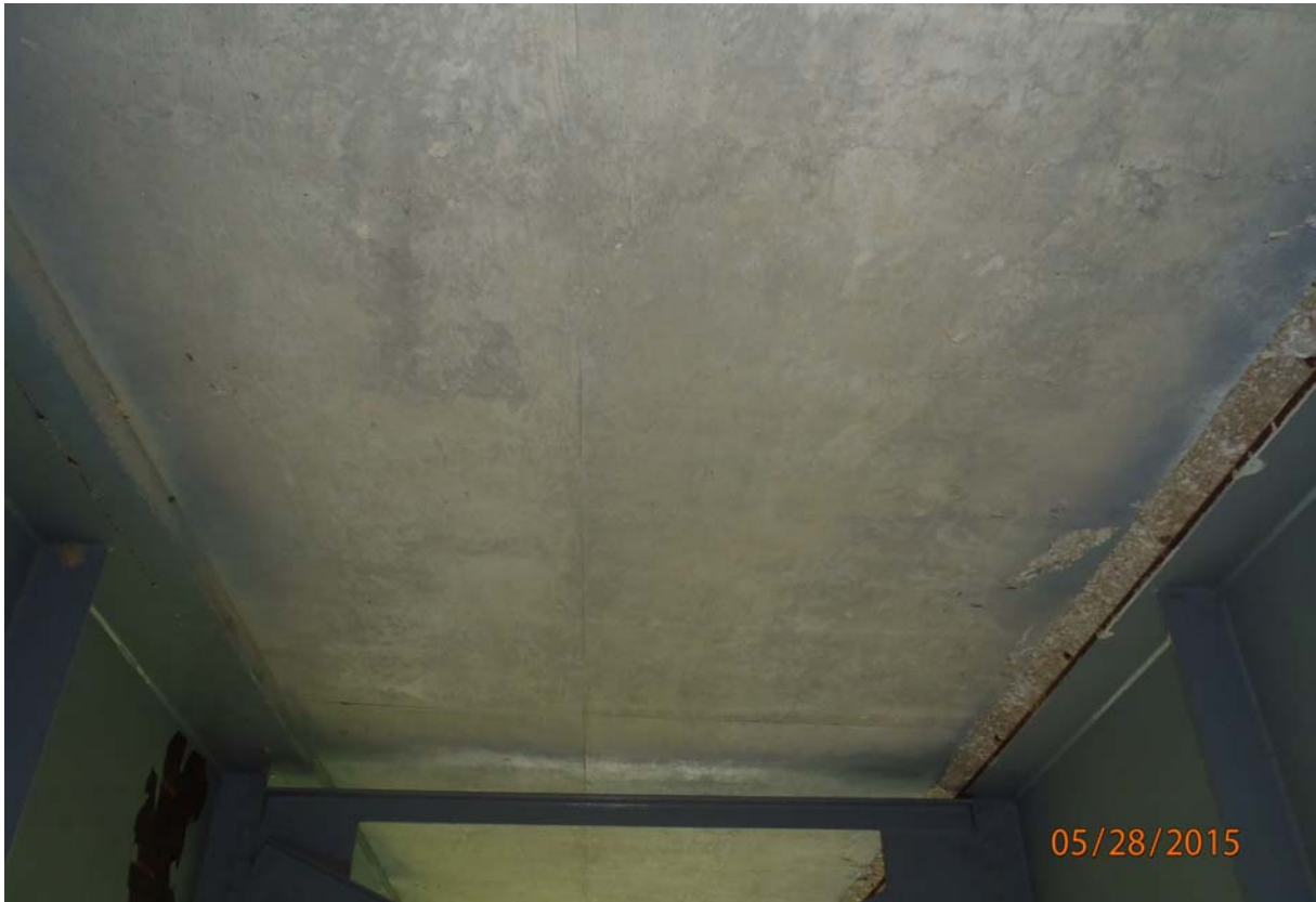
Looking up between beams 1 & 2 in span 4. Note the spalls with exposed reinforcing along the top flange of beam 4.
