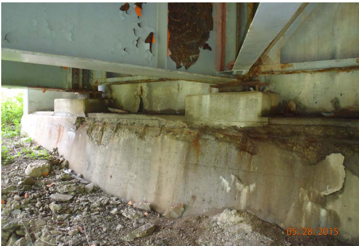
View of the abutment face between beams 1 & 2 of abutment 5. Note the heavy spalls and delimitations with exposed rusting/actively corroding reinforcing steel in the abutment face.
