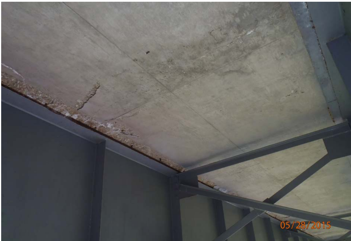
Looking up between beams 3 & 4 in span 4. Note the spalls with exposed reinforcing along the top flange of beam 4.
