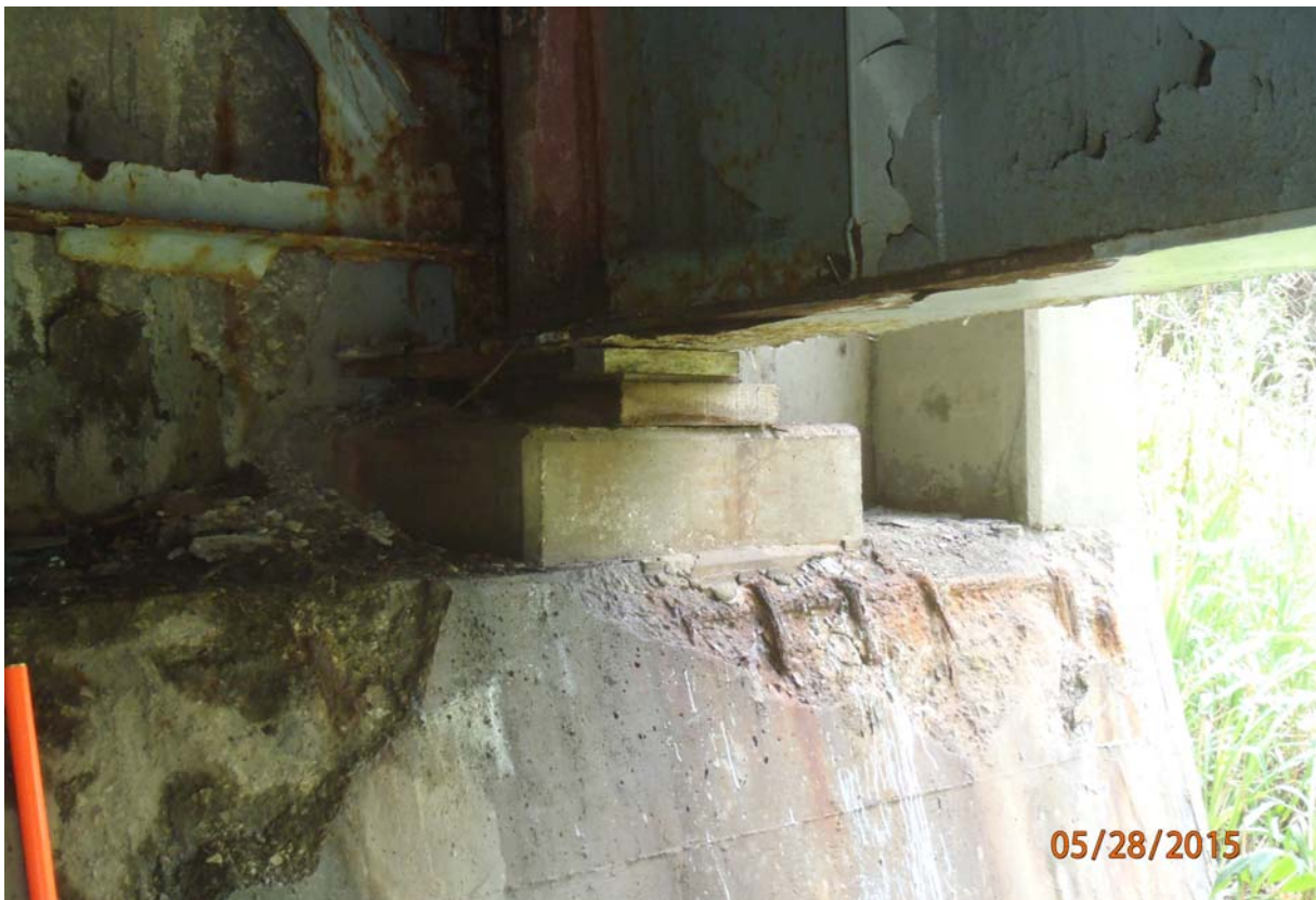
View of wooden blocks placed under the bearing of beam 4. Note the section loss of the beam at the bearing and exposed rusting and actively corroding reinforcing steel of the abutment face. 15/19
