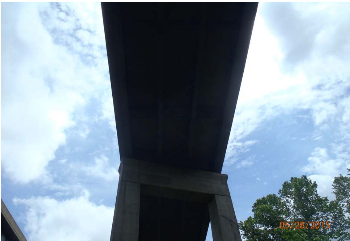
Looking up at the pier cap of pier 4 and deck underside of span 3.
