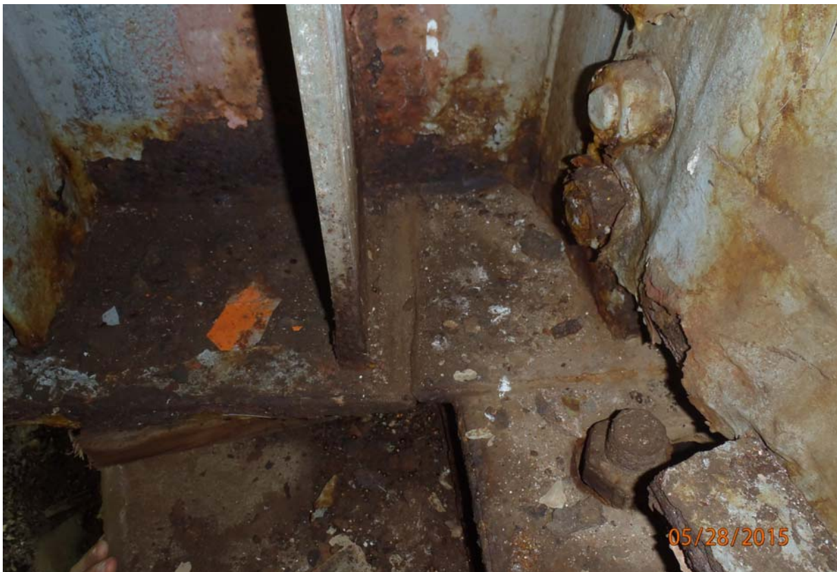
View of the cracking through the lower flange of beam 3 @ the bearing of abutment 5. This crack extends the entire length of the bottom flange. This photo is looking at the downstream face of the beam's bottom flange.
