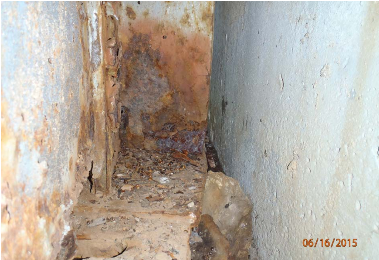
View of the beam end located behind the first vertical stiffener (stiffeners # east to west) of beam 3 @ abutment 5. See the above photo on page 1 for notes.
