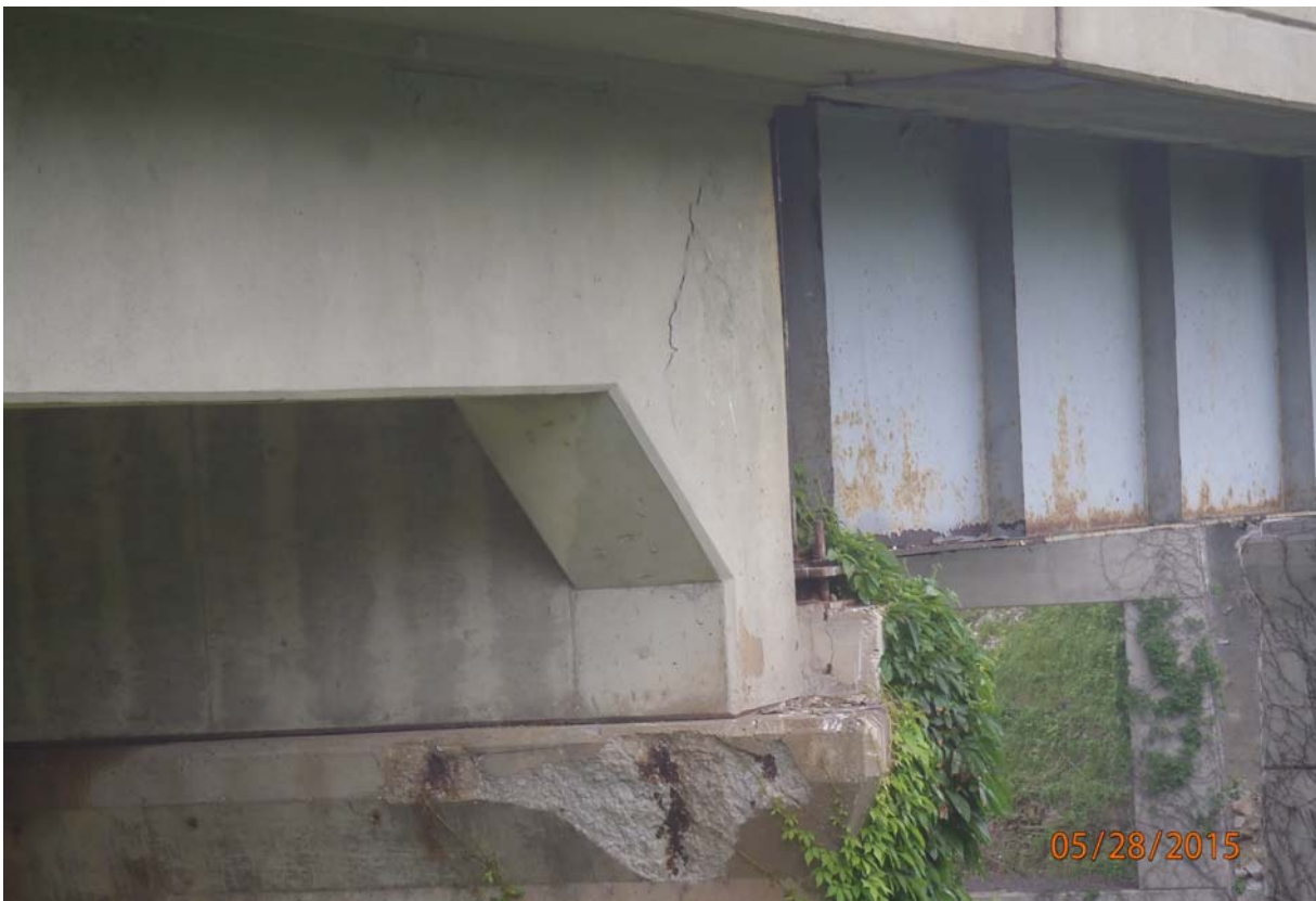
Exterior downstream beam @ pier 2. Note the 5'x2' spall with exposed rusting/corroding steel in the pier cap under the bearing of beam 4. Note the beam has an area above the bearing has light scaling and the start of light delimitation.
