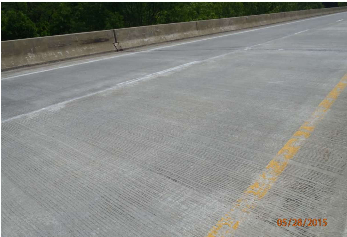
Looking down at the typical condition of the deck/driving surface. Note the deck has recently been overlaid. Note the scaling of the masonry coating on the face of the barrier wall (this is typical along many locations of the wall).
