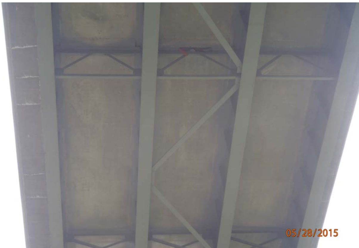
Looking up @ the underside of the superstructure in span 3. Note the transverse cracking with efflorescence on the underside of the downstream overhang.
