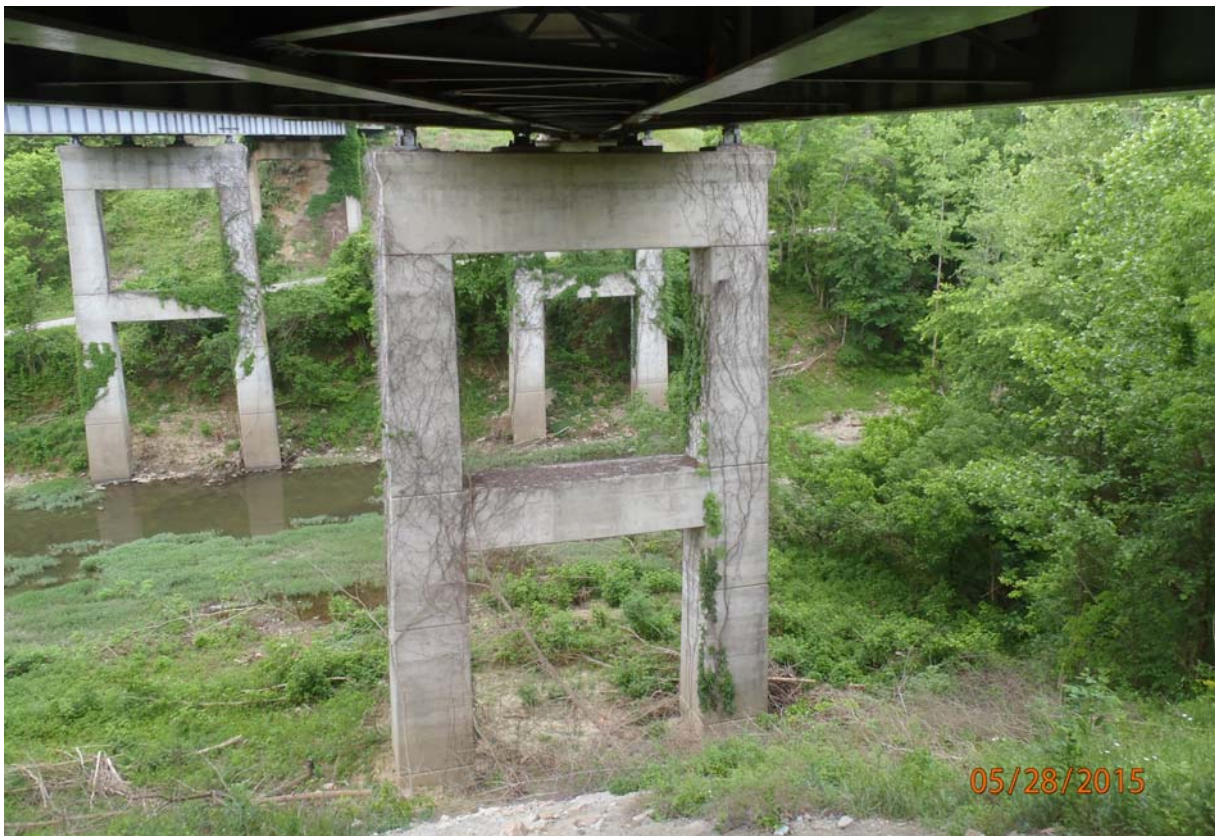
Elevation view of the east face of pier 4. Note the vegetation growth.
