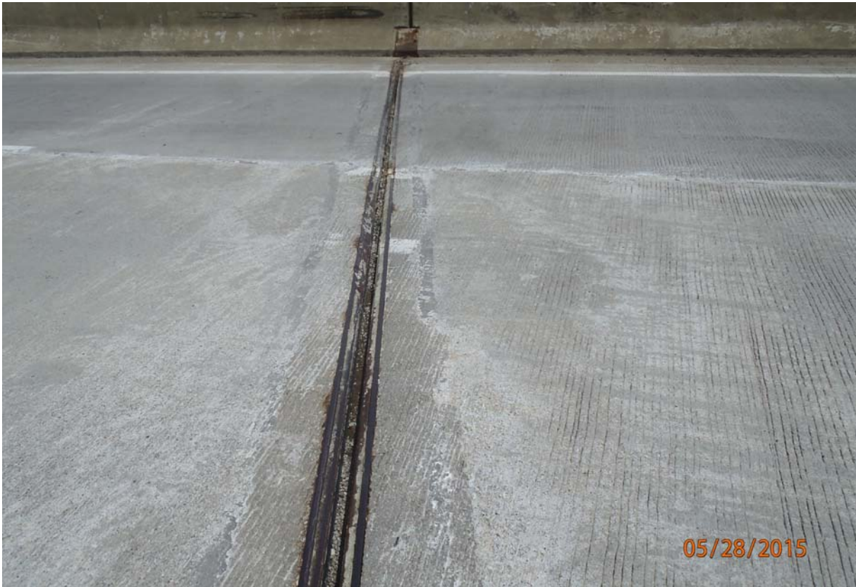
View of the joint over pier 2. Note the joint was recently replaced; only minor amounts of debris are trapped in the joint at this time.
