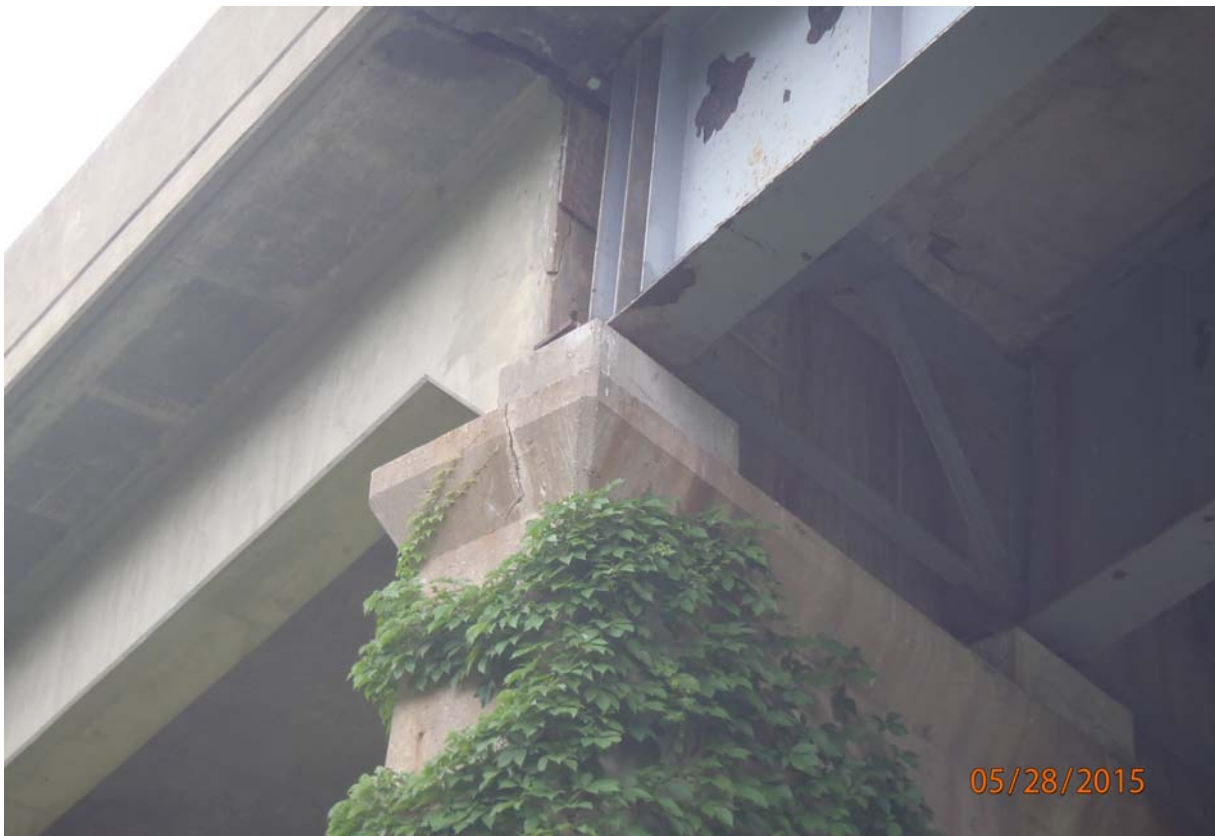
Looking up at beam 4 (#s from upstream to downstream). Note the vertical cracking @ the beam back-face and vertical crack in the exterior face of the pier cap under the bearing of beam 4.
