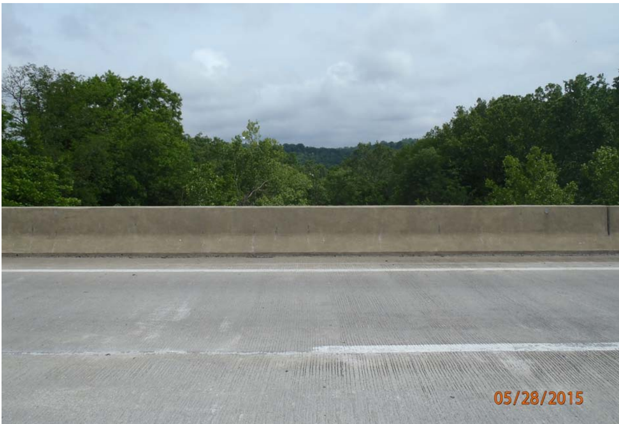
View of the upstream barrier wall. Note minor vertical cracking in the face of the barrier wall along the entire length of wall and many areas of scaling of the masonry coating on the face of the barrier wall.
