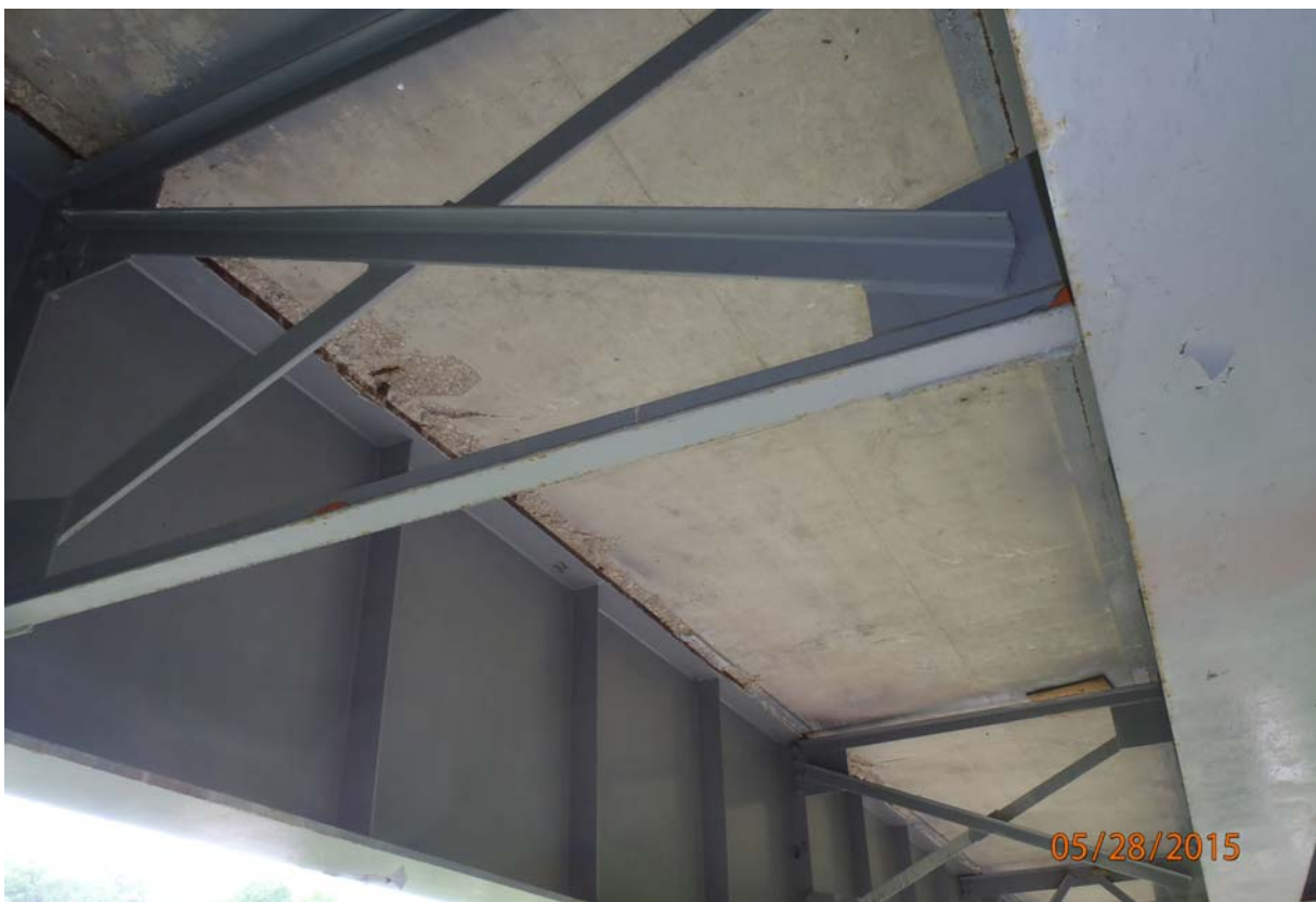
Looking up between beams 3 & 4 in span 4. Note the spalls with exposed reinforcing along the top flange of beam 4.
