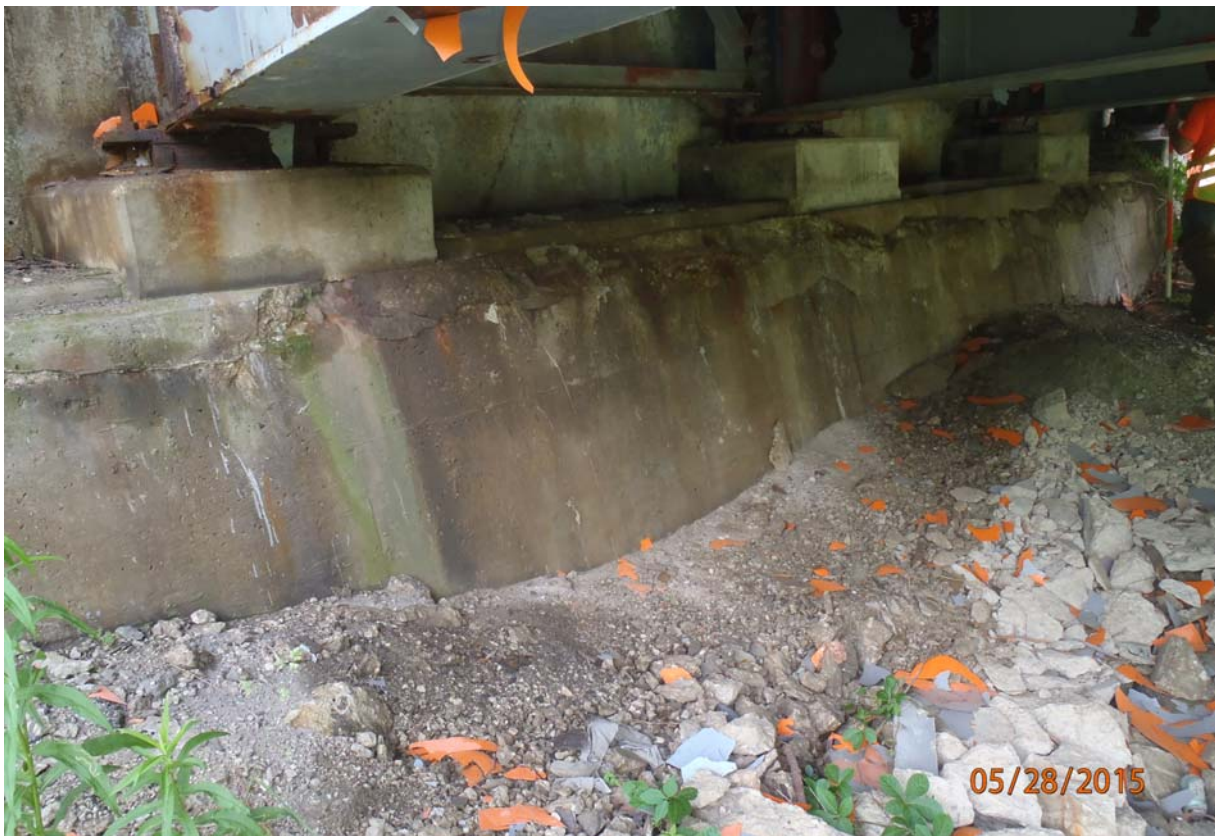
Elevation view of the east abutment (abutment 5). Note the heavy rust staining, horizontal cracking, efflorescence and spalling/delimitation along the abutment seat with rusting/active corrosion of the reinforcing steel. The joint has recently been replaced at this abutment and the abutment needs to be patched.
