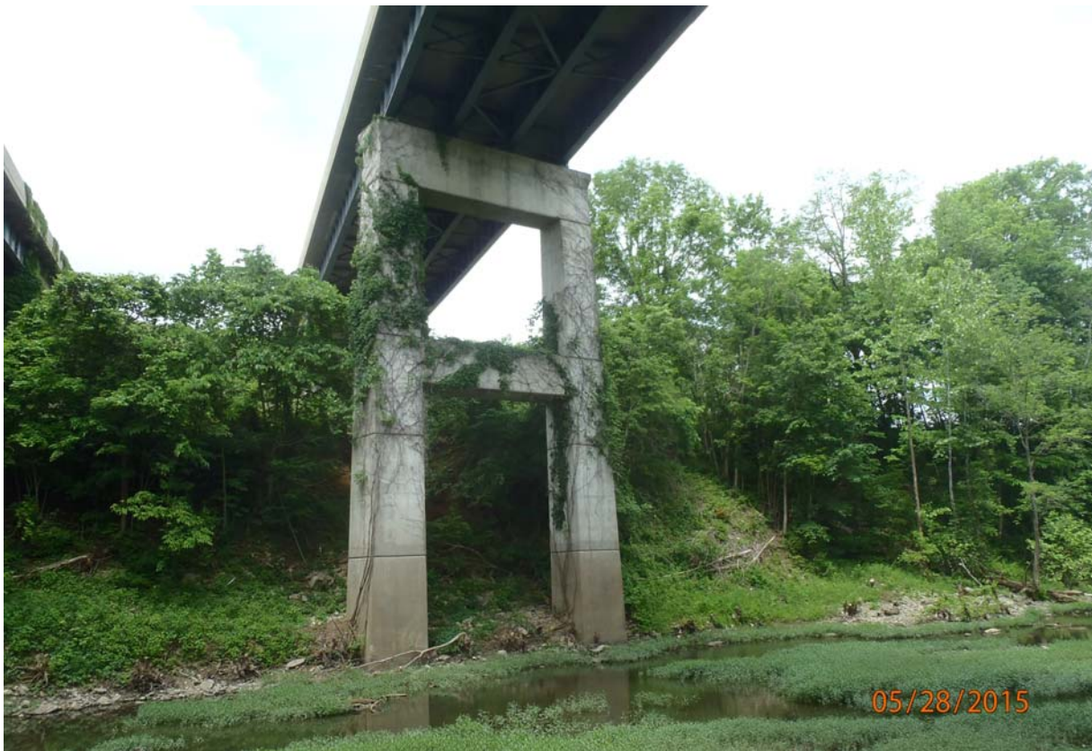
Elevation view of the east face of pier 3. Note water staining on the pier columns and heavy vegetation grown.
