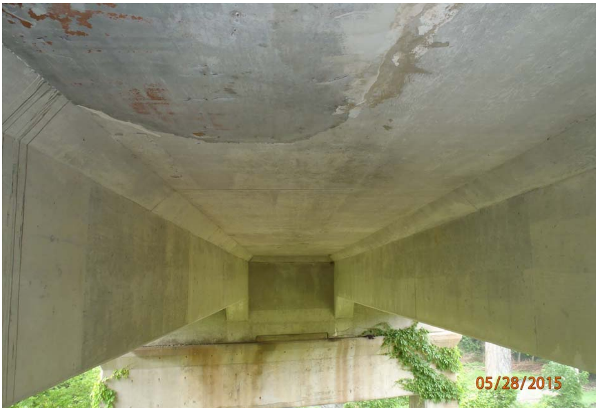
Looking towards pier 2 at the underside of the deck between beams 2 & 3 of span 1. Note the minor pop-outs and spalls with no reinforcing exposed throughout the deck underside in span 1.
