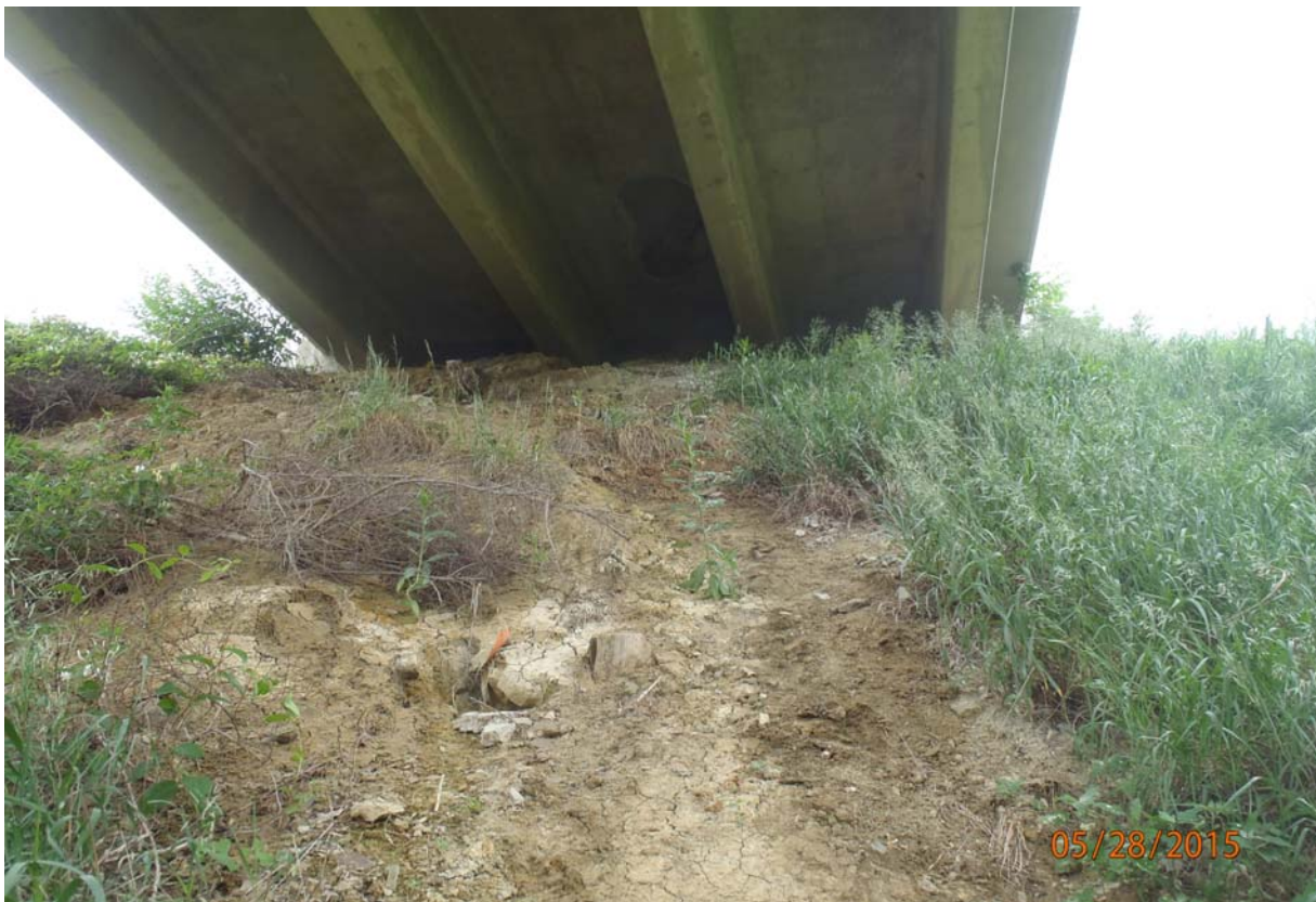
Looking at the embankment in-front of the west abutment. Note the minor erosion.
