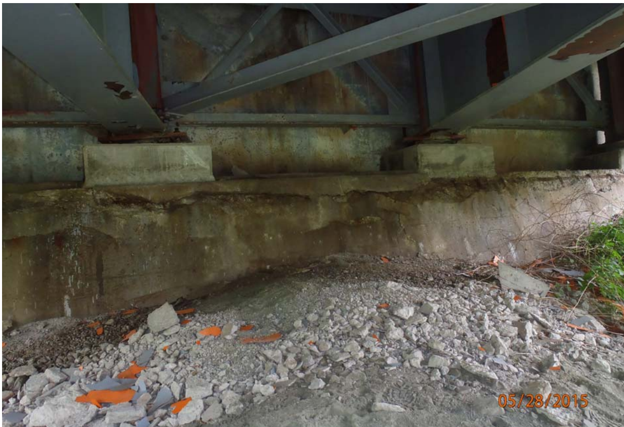
View of the east abutment (abutment 5) between 2 & 3. See notes above for abutment notes.
