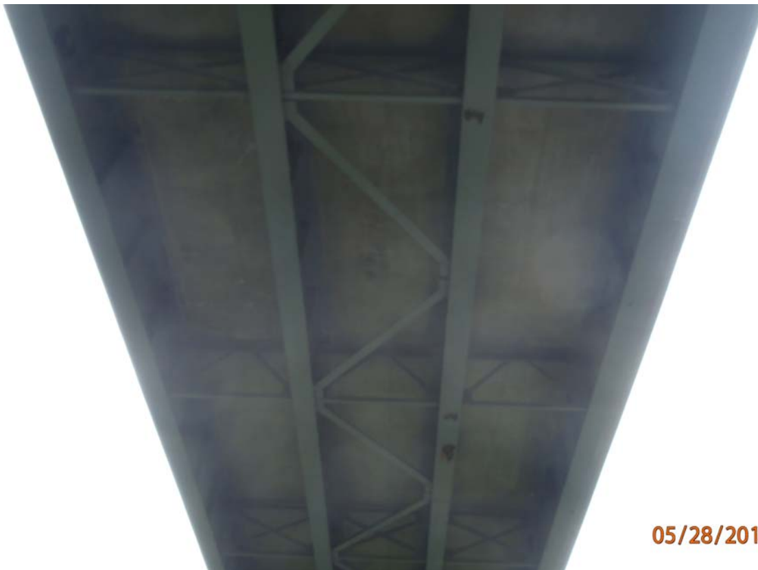
Looking up at the underside of span 2. Note the transverse cracks with efflorescence on the deck underside throughout the span; these cracks are more dominant near mid-span; there is evidence of water staining near midspan on the deck underside. 5/16
