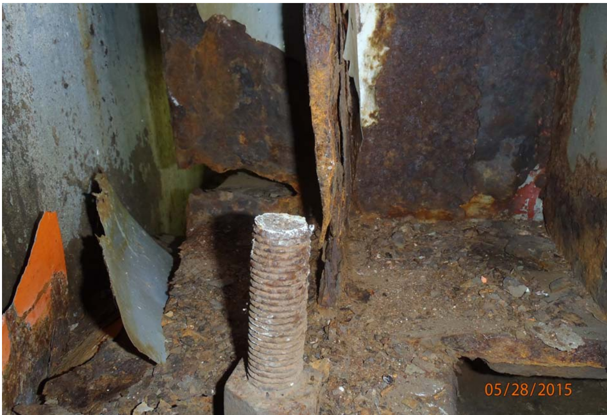
Looking at the upstream face of beam 1 @ abutment 5. Note the 6 5/8" long crack in the web near the bottom flange extending from the beam end towards the 1st vertical stiffener; this crack initiated from a corrosion hole. Note the bottom flange is heavily corroded and thinner @ the bearing location (up to 1/8" section loss).
