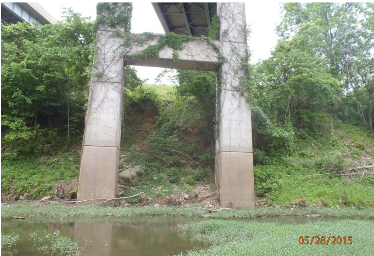
View of the east face of pier 3. Note the water staining and light wearing of the concrete surface from the normal stream level.
