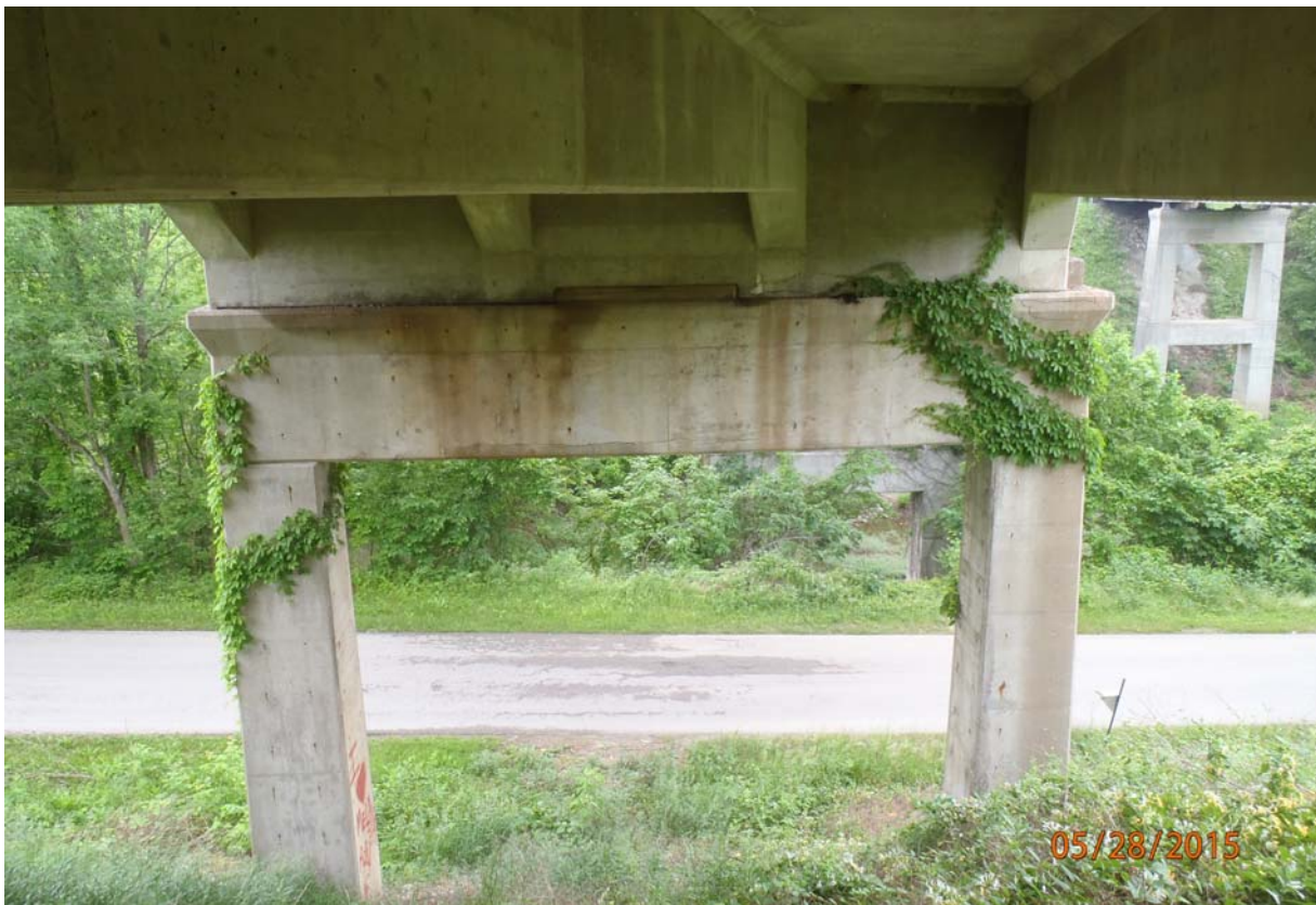
Elevation view of the west face of pier 2 (#s start at the west abutment and account for both piers and abutments). Note the vegetation growth and horizontal cracking in the pier cap and diaphragm. The cracking in the diaphragm is under beams 2, 3 and 4.
