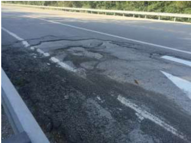
Asphalt mat tearing
