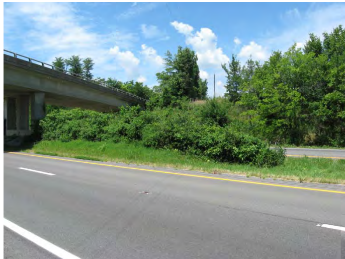
Eight overpass bridges have crash pier protection that does not meet current standard
