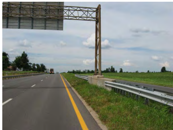
Mayfield Bypass median and inside paved shoulder width does not meet current interstate standard
