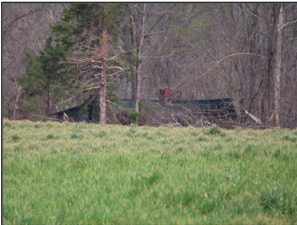
Figure A-10: TR 88: Overview towards the residence showing the partially collapsed roof, looking northwest.
