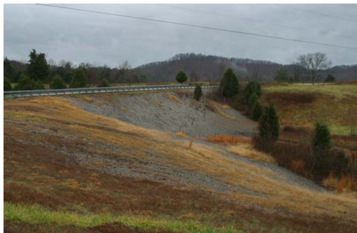
Photo 8. Existing Roadway Fill Composed of New Albany Shales - Shows Lack of Vegetation Probably Due to Acidic Drainage from the Shale
