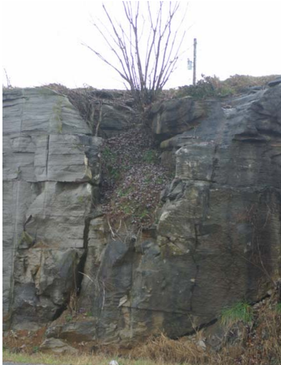
Photo 6. Solution Weathering Observed Within Cut Along KY 55 in the Mississippian Plateaus Physiographic Region
