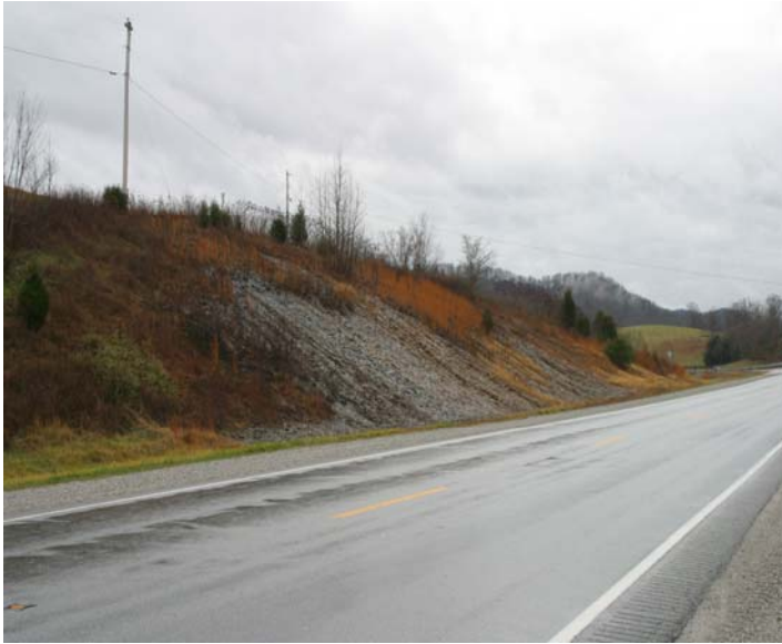
Photo 7. Existing Roadway Cut Along KY 55 South of Lebanon Within The Knobs Region - Cut in New Albany Shales Exhibiting Sparse Vegetation Because of Acidic Drainage
