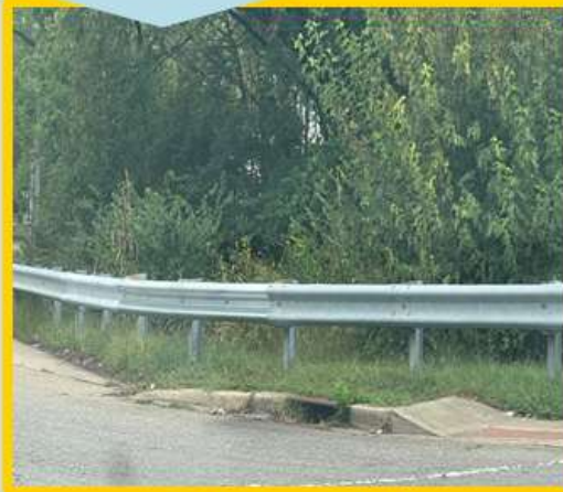
ADA Ramp with No Connectivity
