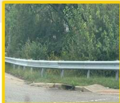
ADA Ramp with No Connectivity
