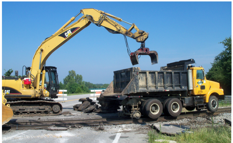
Source: Kentucky Transportation Cabinet
