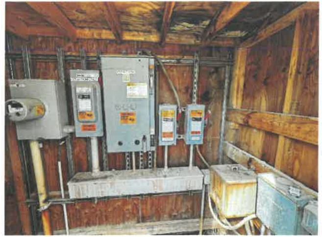
Electrical control room
