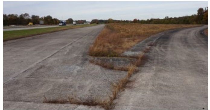
Figure 7-6. I-24 Closed Parking (Lyon County) ID29 Site Photo
