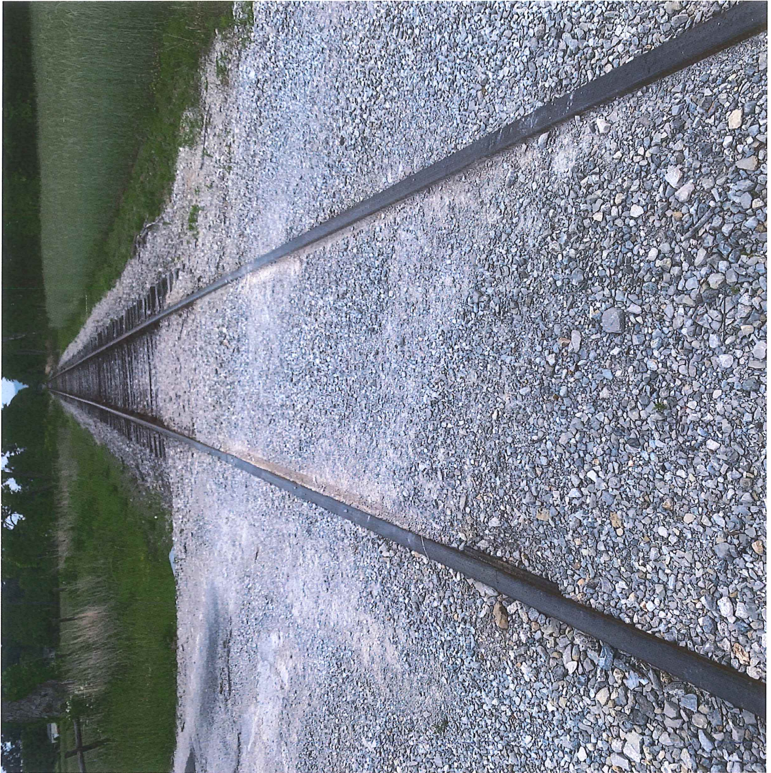
GRAVEL WAS PUT DOWN OVER DEGRADED ASPHALT & TIMBER/TIES TO SMOOTH CROSSING SURFACE UNTIL CROSSING COULD BE REDONE
