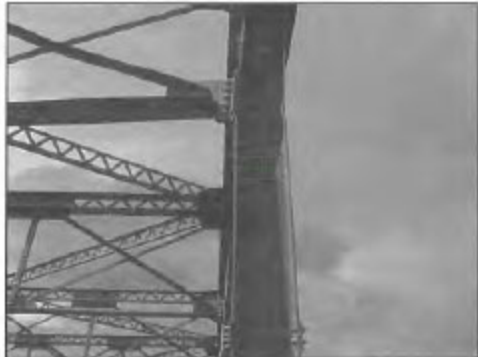
Figure B-15—Sway Bracing Impact Damage in Span 1
