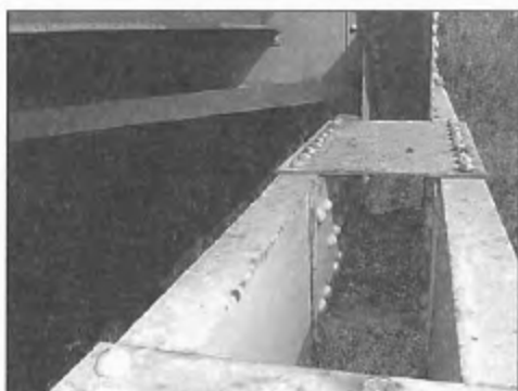
Figure B-16—Freckle Rust, Typical, Both Trusses, Both Spans
