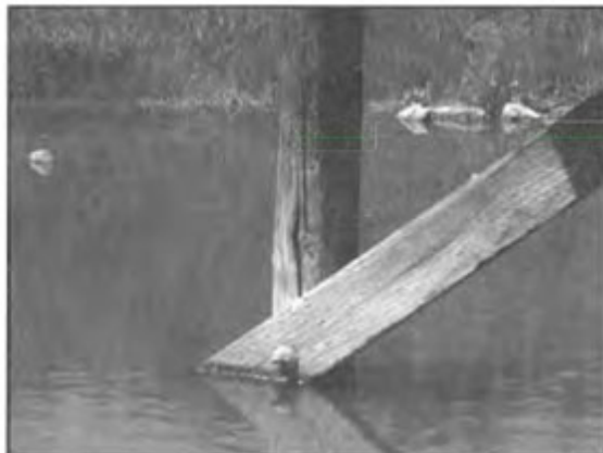
Figure B-4-7-in. Deep Check in Right Exterior Pile of Bent 2
