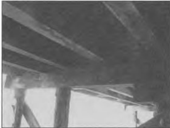
Figure B-3-1-in. Deep Check in Bent Cap at Bent 2
