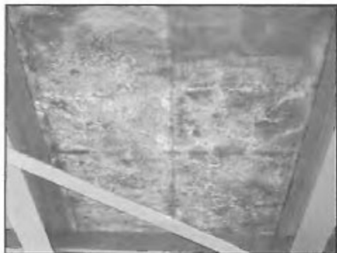
Figure B-14—Efflorescence on the Underside of the Deck in Span 1
