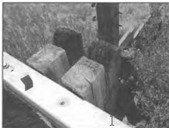
Figure B-5-Decay in Timber Rail Posts
