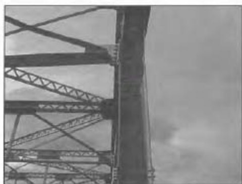
Figure B-15—Sway Bracing Impact Damage in Span 1
