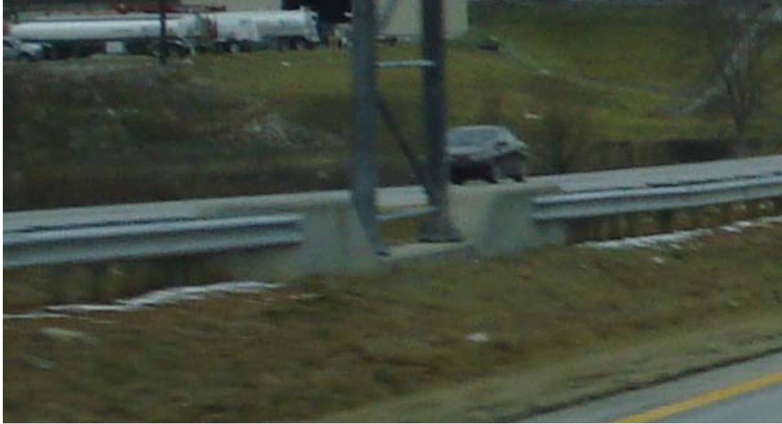
GAP IN SIGN TRUSS SUPPORT
