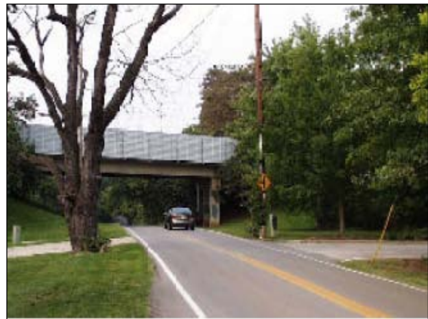
G. "Before" Wolf Pen Branch Road Bridge near Springdale Road, Prospect, KY.
