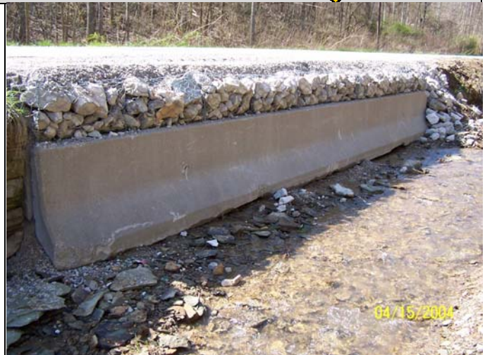
Embankment repair using movable concrete barrier walls and channel lining prevents erosion of the embankment and roadway collapse along a stream.
