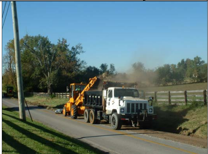
This dump truck will be covered to transport soil removed during this ditching operation.
