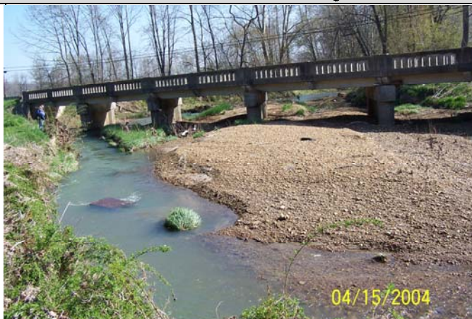
Loose rock and sediment may deposit at culvert and bridge openings and should be removed to prevent misalignment of the stream and erosion of the structures and nearby roadway.
