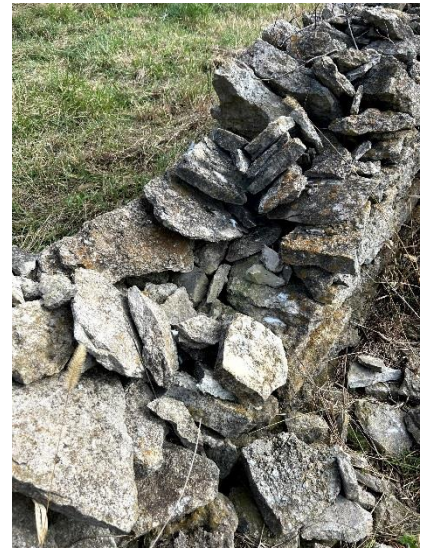
North F close up, showing face stone lengths oriented inward with minimal space and packing between faces.
