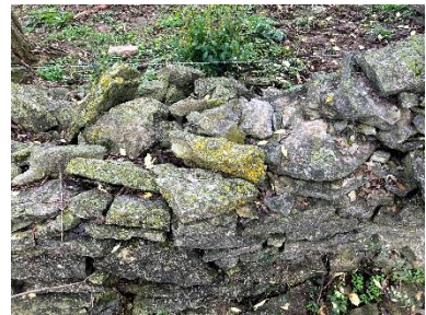
South F perpendicular fence, failure at 75', showing face stones length in.
