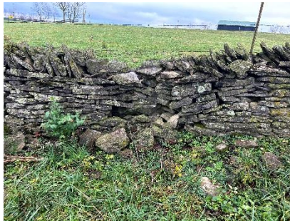
South perpendicular F, showing full depth tie stone in the center that prevented total collapse.
