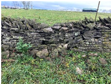
South F perpendicular fence, showing tie holding fence up.
