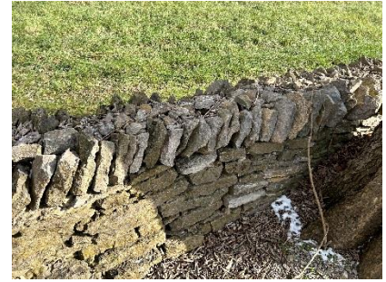
Groverland roadside fence, showing an unrepaired section with original double copes, random build and no face chinking.
