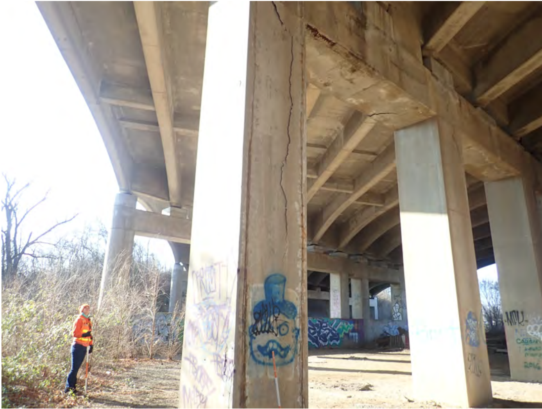
Pier 5-Column 2 with side vertical cracking on multiple faces
