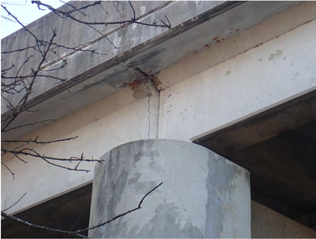
Pier 2-Girder 14 with vertical cracking at beam end
