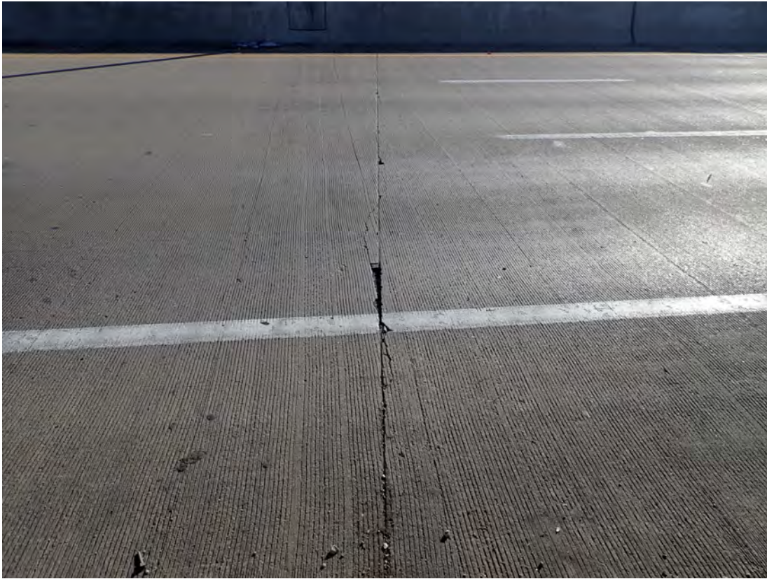
Relief cut over Pier 4 EBL with what appears to be a pourable sealant material across 53 feet of the deck with edge failure at random locations along length of joint. 10 feet affected by sealant failure
