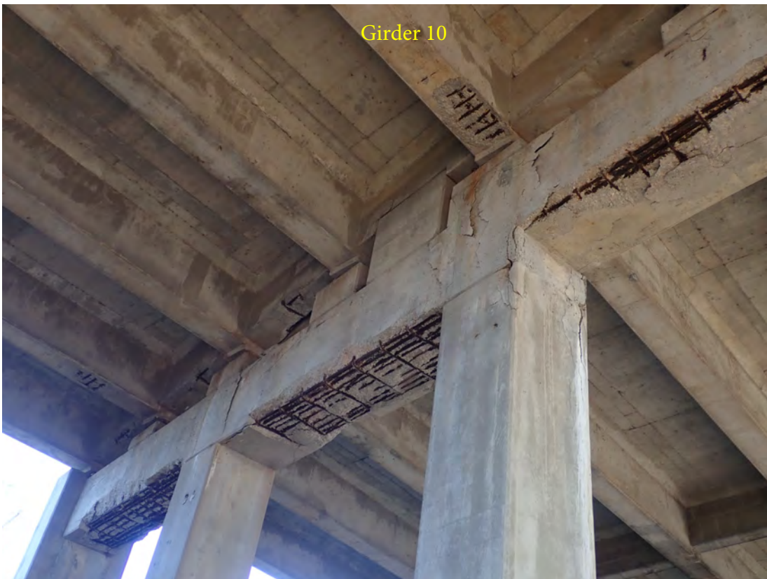
Span 3-Pier 3-Girder 10 with spalling and exposed steel reinforcement
