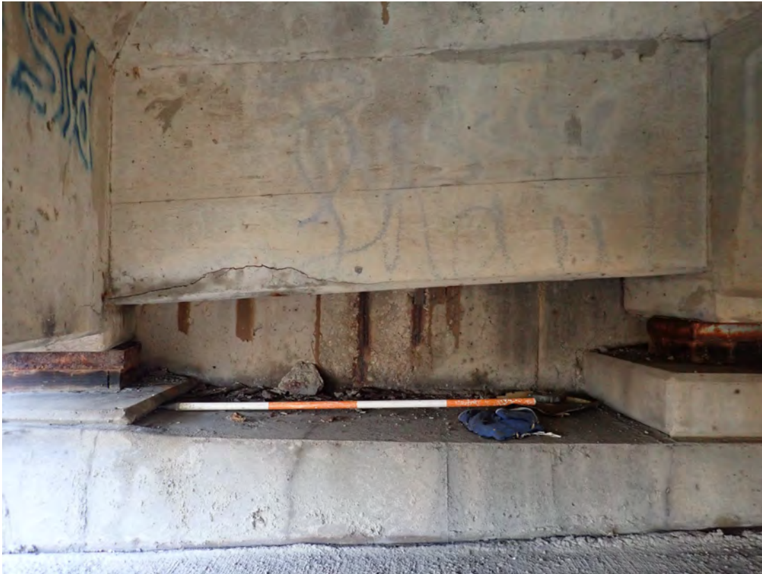
South end of Abutment 1 with spalling, exposed steel reinforcement with section loss
