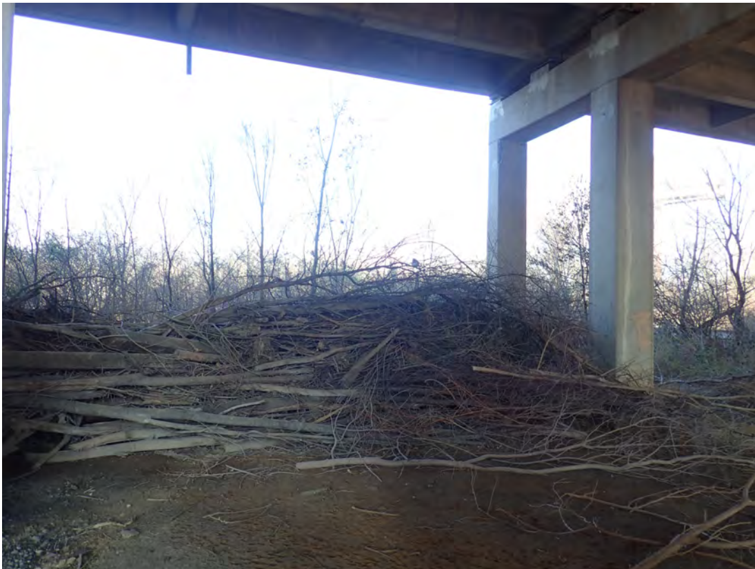
Closer view of debris pile through Span 4
