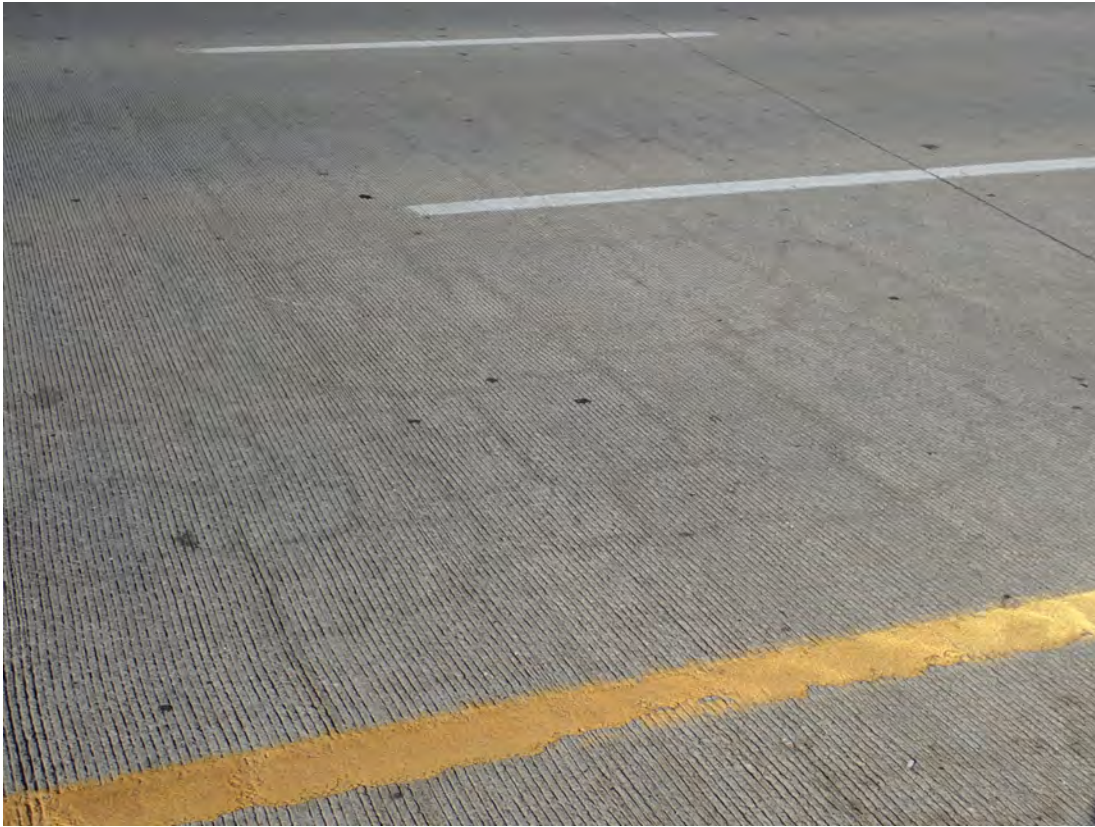
Map cracking noted in deck over Span 1
