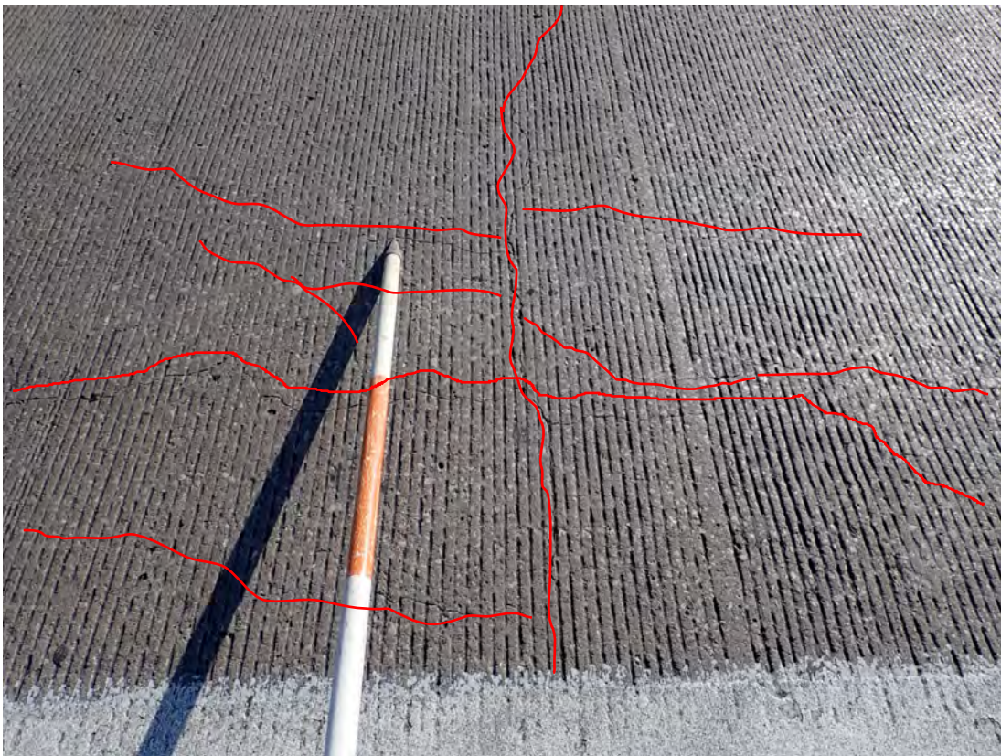
Map cracking typical of that found in deck over Span 2
