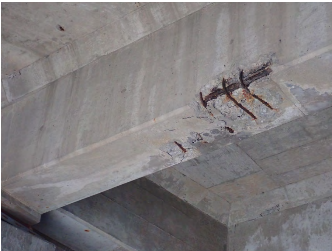
Span 2 girders have spalling with exposed steel reinforcement
