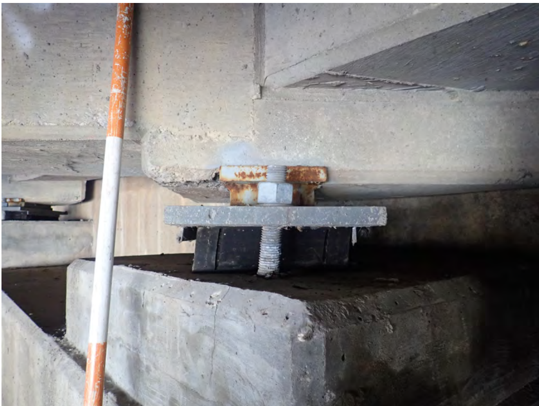
Abutment 8-Girder 12 with misaligned anchor bolt and slight expansion of the elastomeric pad toward the abutment backwall
