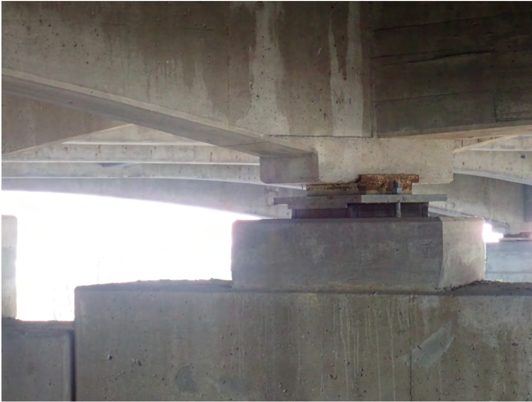
Typical repaired condition of bearing devices and pedestals at Pier 7
