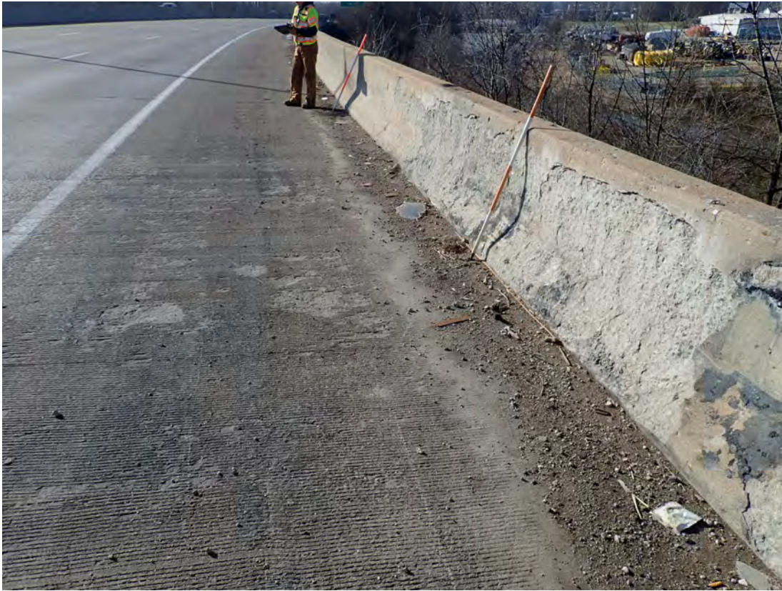
Fire damage along the south barrier wall of EBL in Span 2
