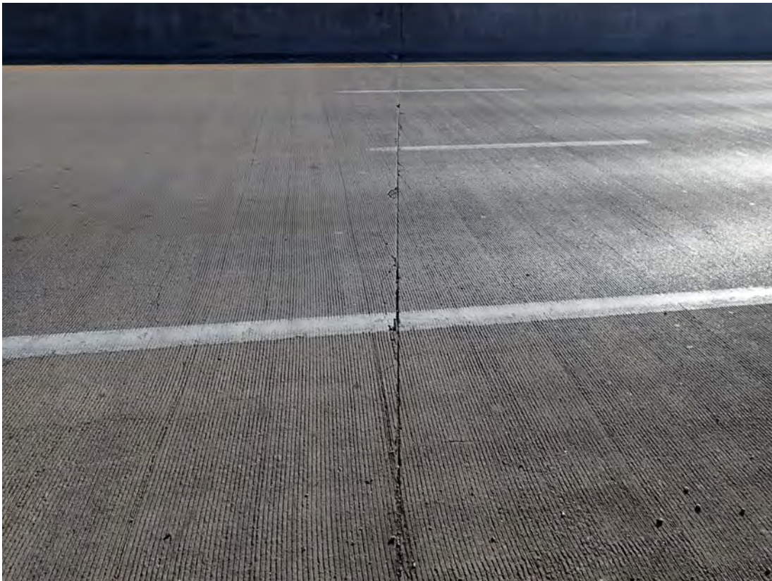
Relief cut over Pier 2 EBL with what appears to be a pourable sealant material across 53 feet of the deck with edge failure at random locations along length of joint. 16 feet affected by sealant failure
