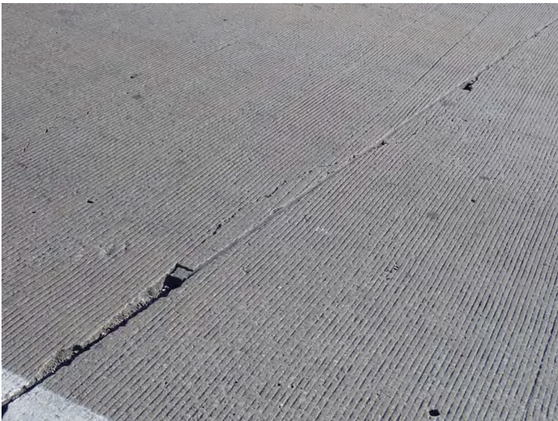
Closer view of edge failure over Pier 4 EBL
