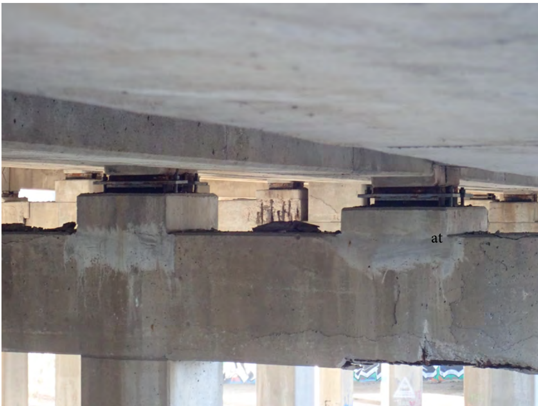
Typical repaired bearing device & pedestal condition at Pier 2
