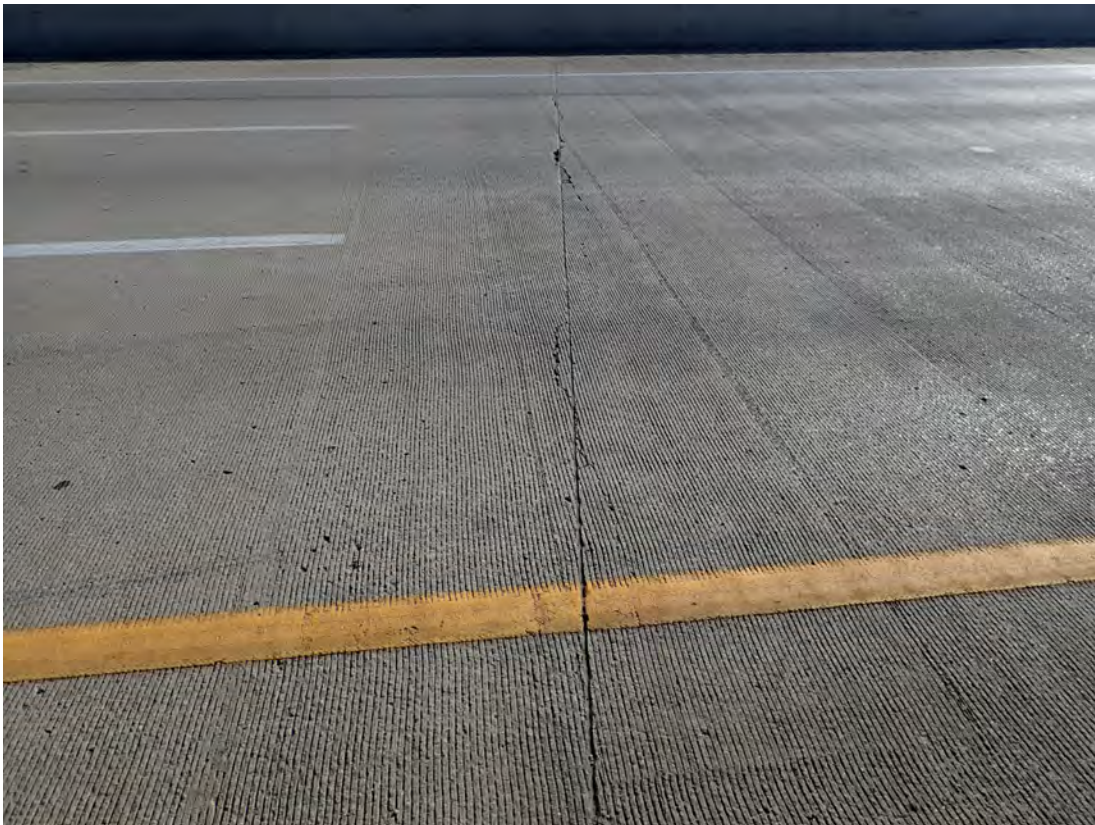
Relief cut over Pier 3 WBL with what appears to be a pourable sealant material across 53 feet of the deck with edge failure at random locations along length of joint. 4 feet affected by sealant failure
