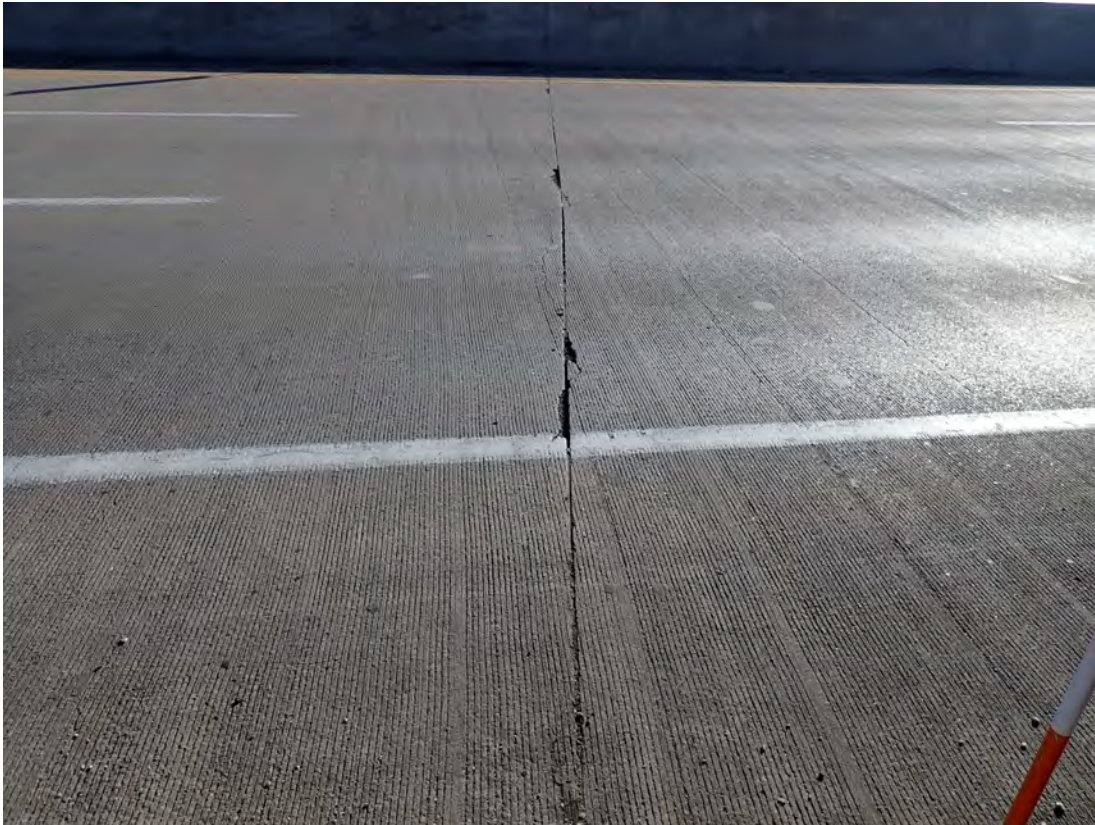
Relief cut over Pier 3 EBL with what appears to be a pourable sealant material across 53 feet of the deck with edge failure at random locations along length of joint. 14 feet affected by sealant failure
