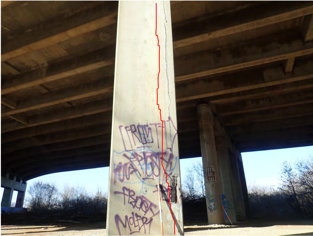
Pier 5-Column 2 south face with full height wide vertical cracking
