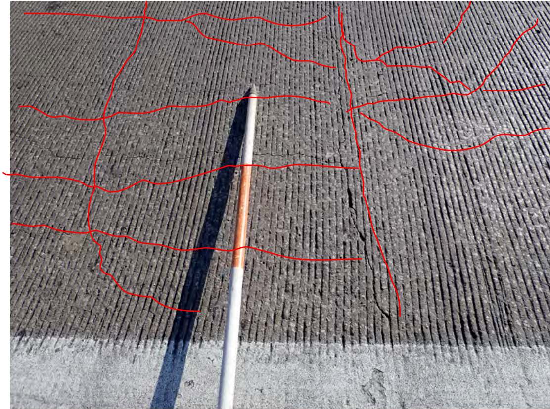
Closer view of dense map cracking in Span 1 -- heavier amounts typical of all but Span 4 EBL; affects full length of WBL & full lane widths in each direction of travel
