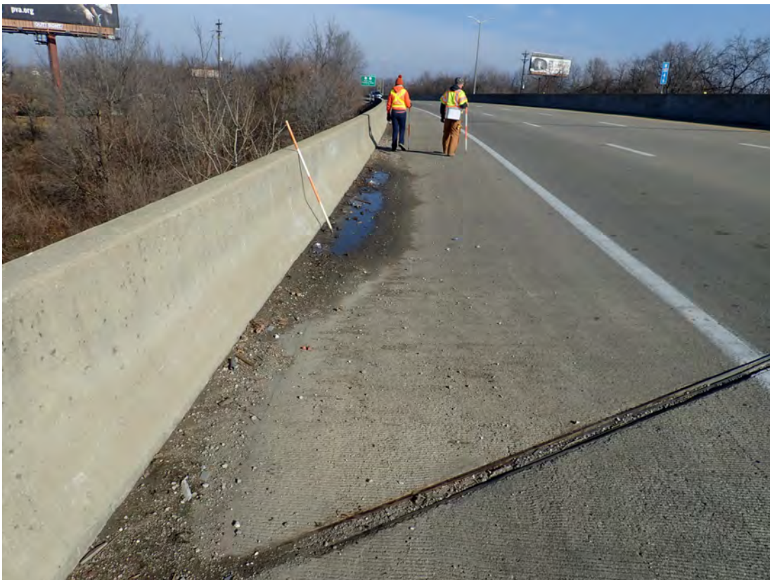
Ponding against barrier wall in Span 4 EBL
