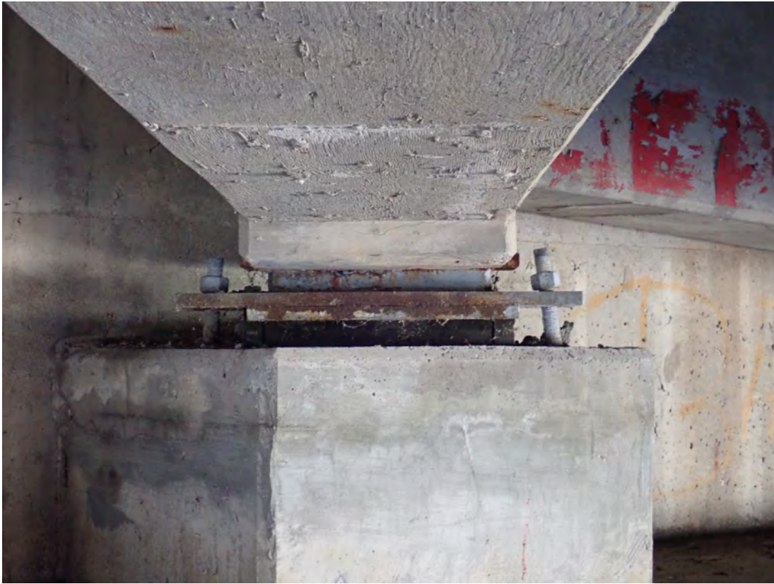
Abutment 8-Girder 12 with misaligned anchor bolt
