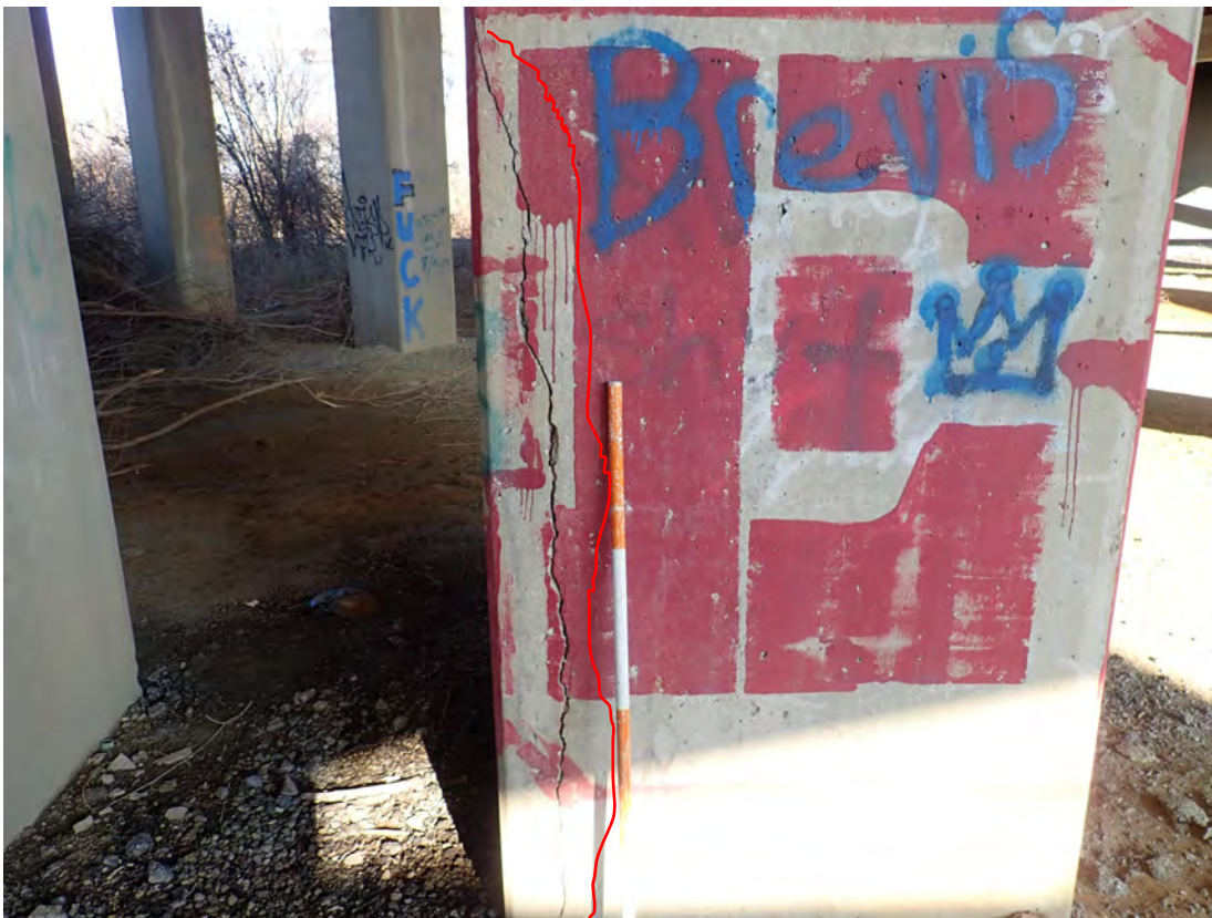
Pier 5-Column 4 with wide vertical cracking
