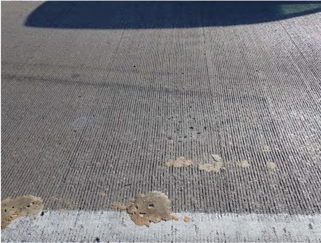
Deck has popout aggregate failures throughout
