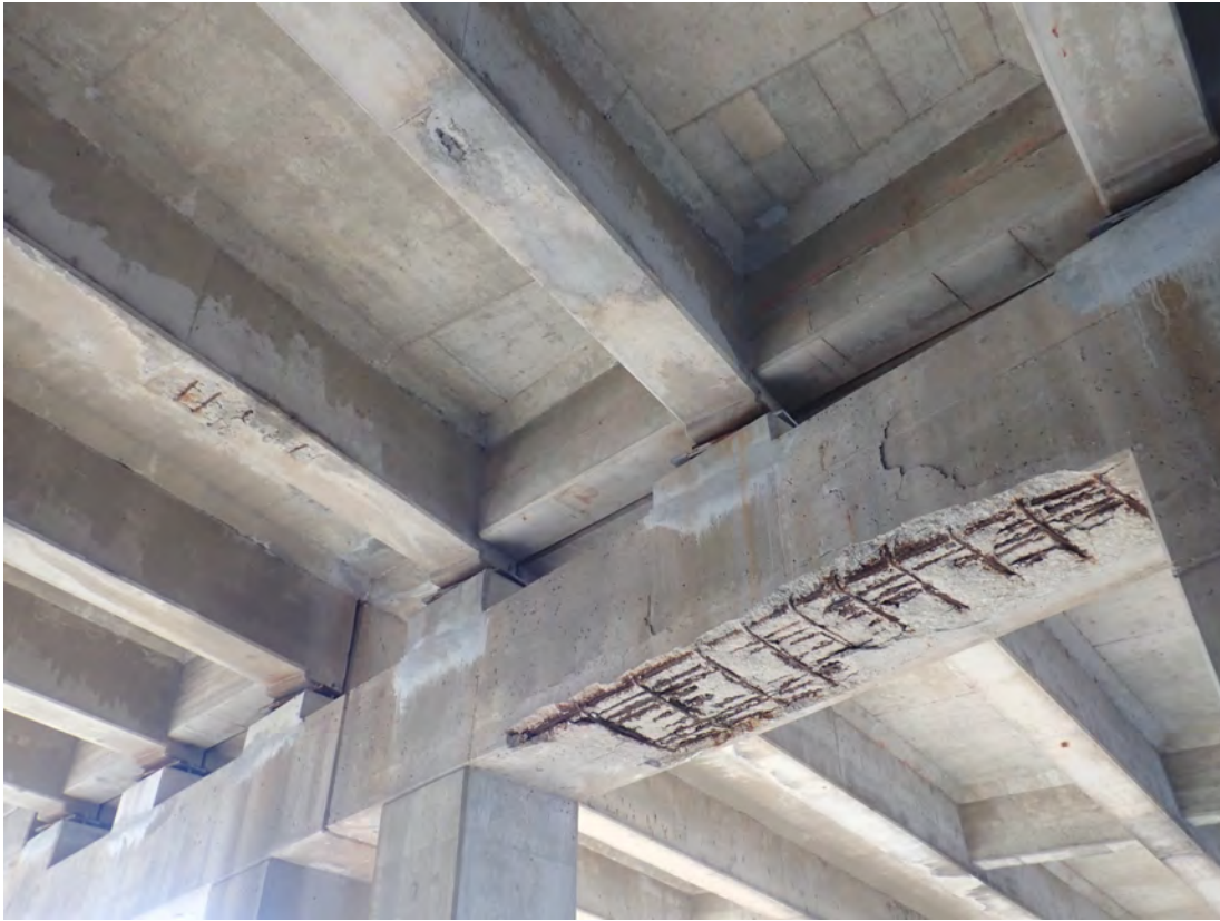
Looking up at Span 2 girders with patched areas & Pier 2 cap deterioration
