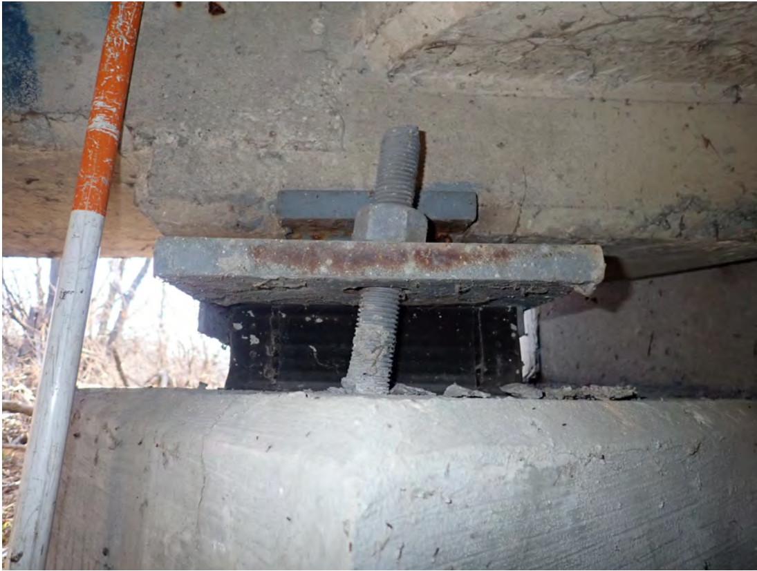
Abutment 8-Girder 1 anchor bolt appears to have been epoxied out of vertical plumb, as the bearing pad has no sign of expansion
