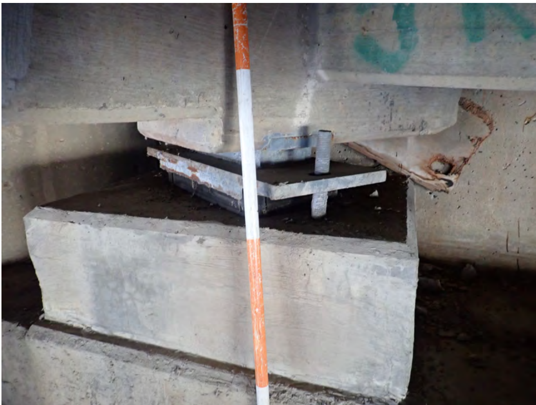
Abutment 8-Girder 5 missing nut on north side
