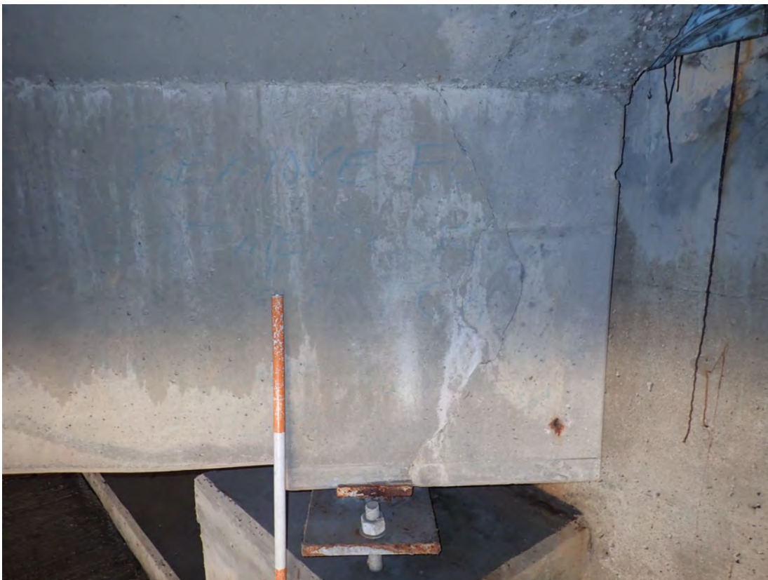
Abutment 8-Girder 10 with vertical/diagonal cracking just behind the sole plate of bearing device
