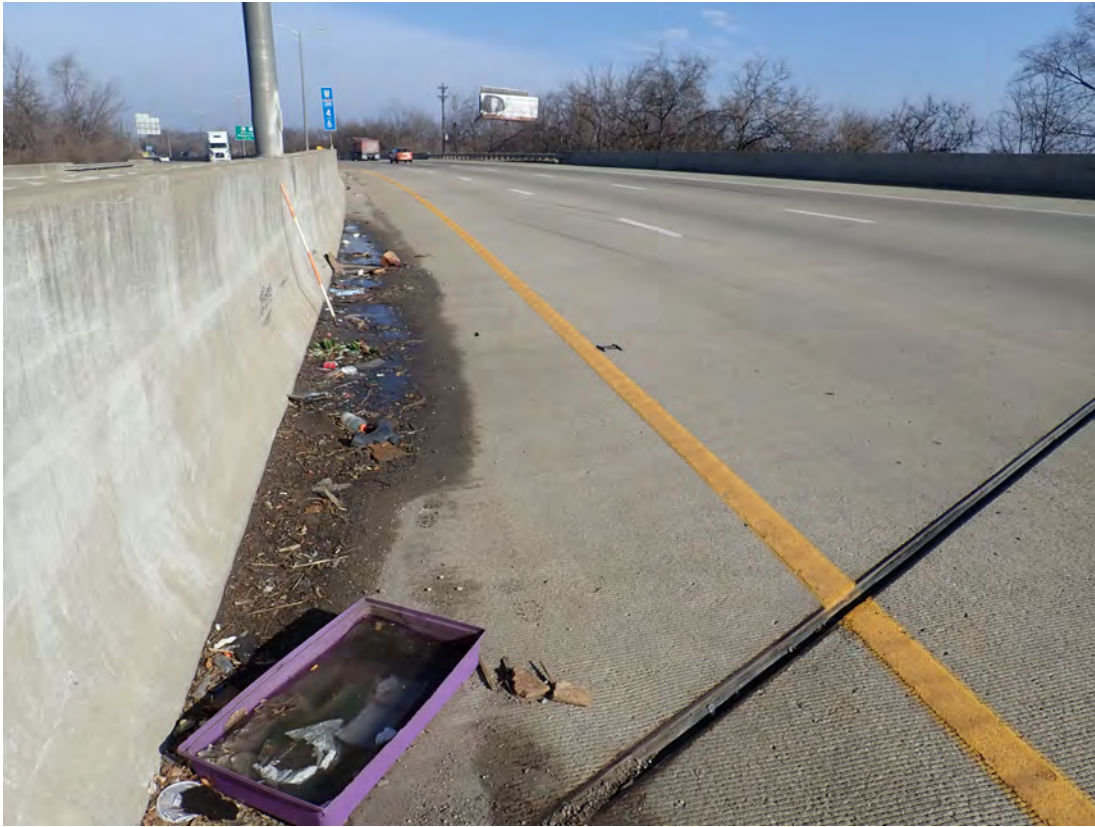
Ponding along barrier wall in Span 4 WBL
