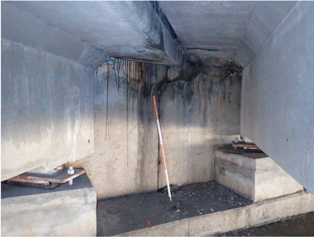
Centerline of Abutment 8 backwall with cracking and staining
