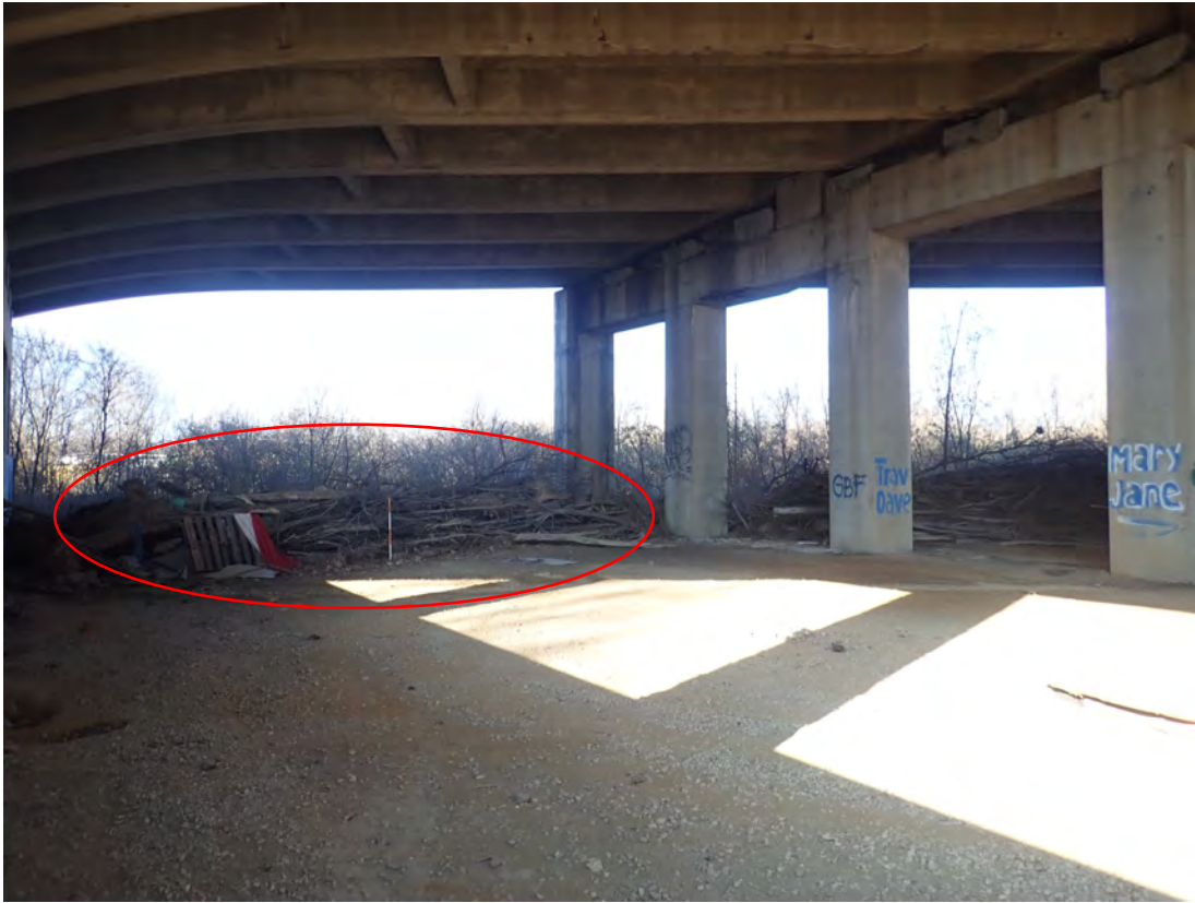
Cut brush debris stacked up between Spans 4 & 5
