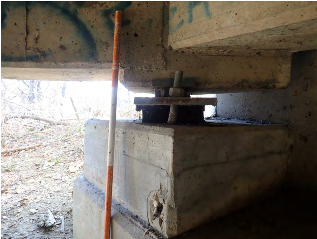
Abutment 8-Girder 1 pedestal spalling
