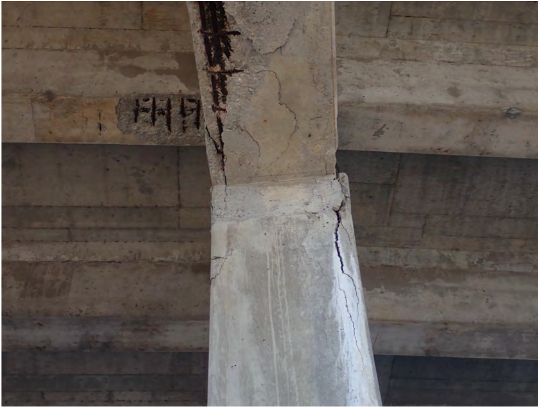
Pier 3-Column 6 with wide cracking & delamination near bottom of cap
