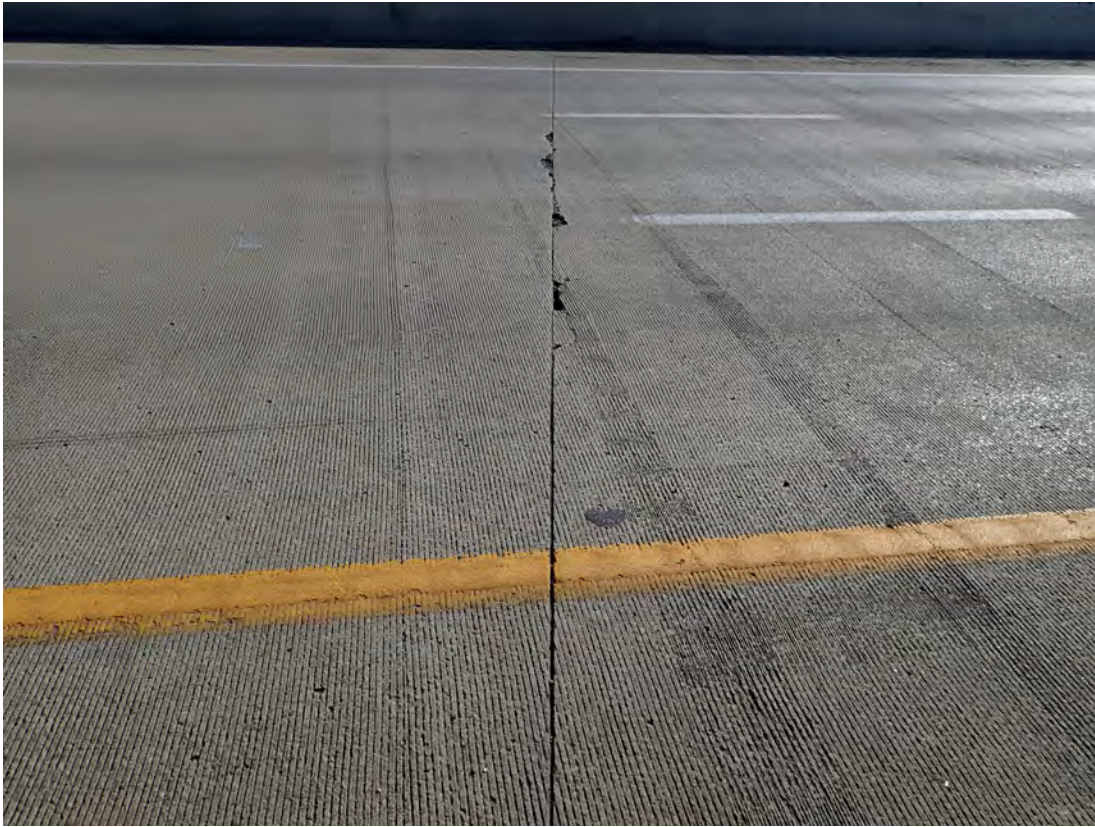
Relief cut over Pier 2 WBL with what appears to be a pourable sealant material across 53 feet of the deck with edge failure at random locations along length of joint. 9 feet affected by sealant failure
