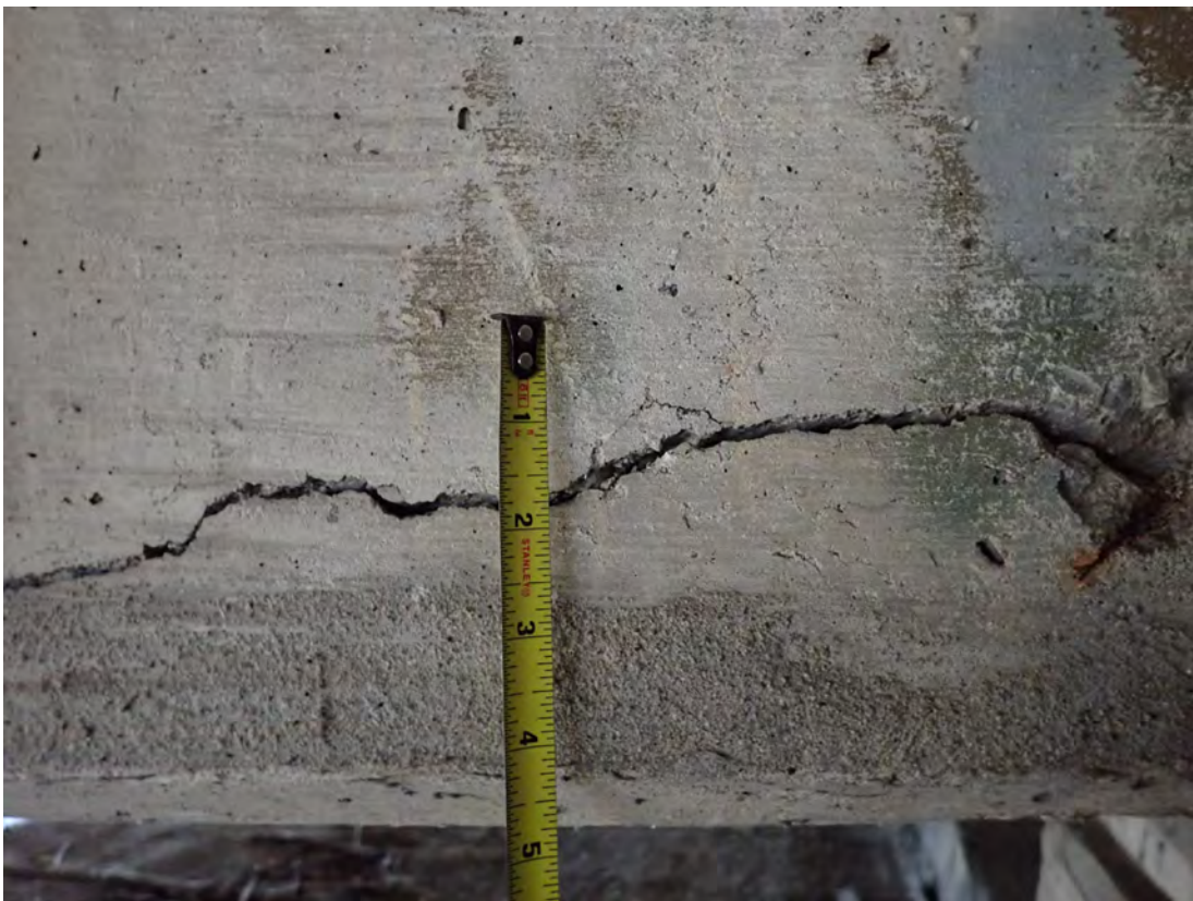
Closer view of Abutment 1-Girder 12 with side longitudinal cracking in lower portion of beam web
