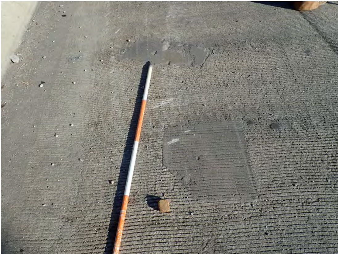
Some areas in emergency lane EBL with sound patching
