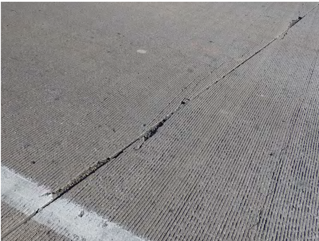
Closer view of edge failure over Pier 3 EBL
