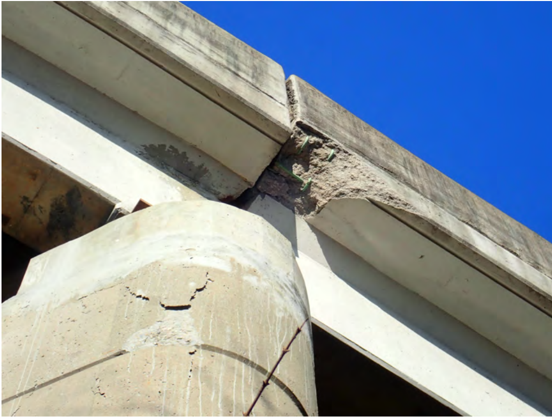
Deep large spalling in overhang above north end of Pier 5
