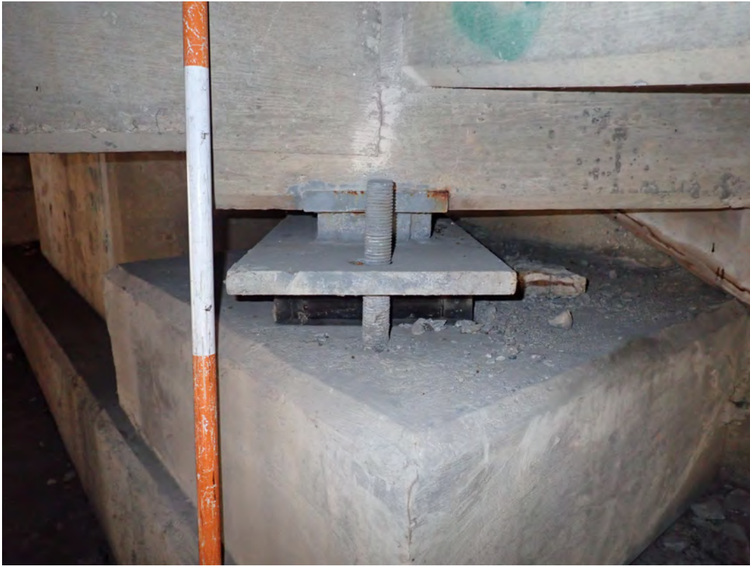
Closer view of Abutment 8-Girder 7 missing nut on north side -- note vertical cracking over bearing
