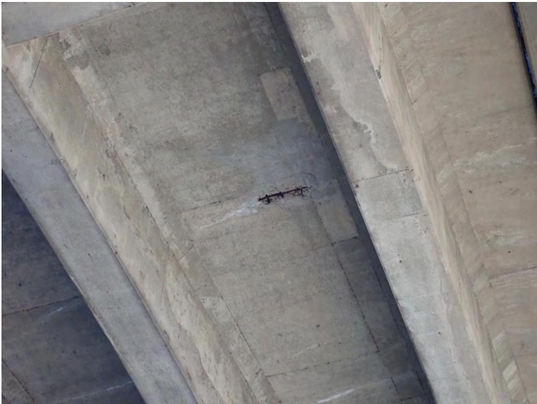
Deck soffit has some spalling with exposed steel reinforcement
