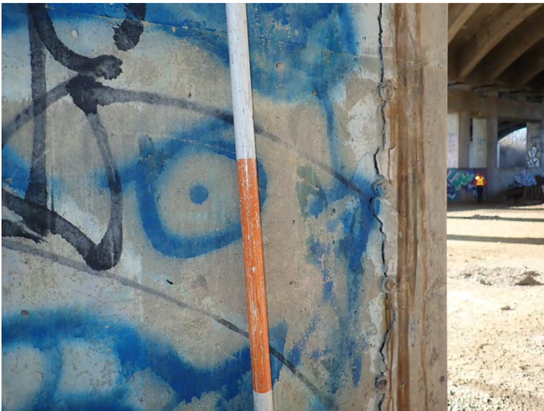
Pier 5-Column 2 west face with full height wide vertical cracking along a line of epoxy injection locations made as part of 2003 rehab project
