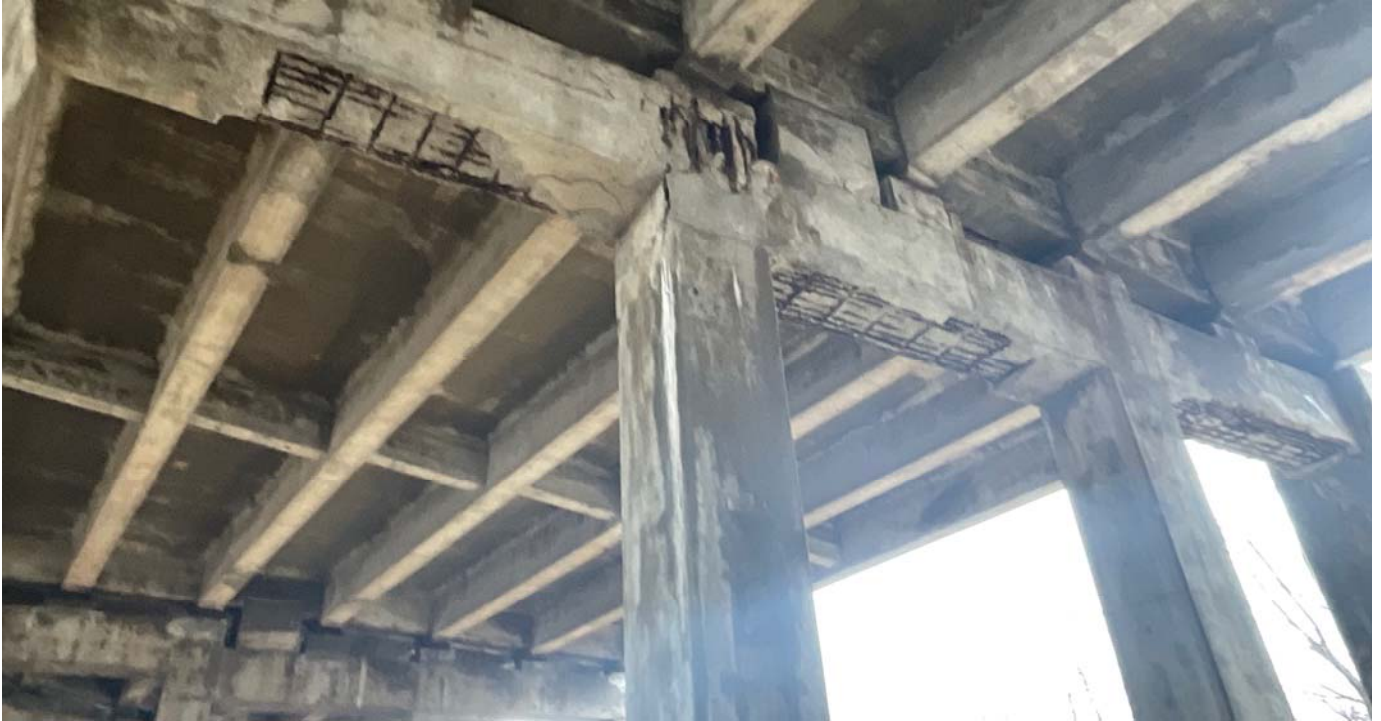
Pier 3 - Column 6 spalling at top
