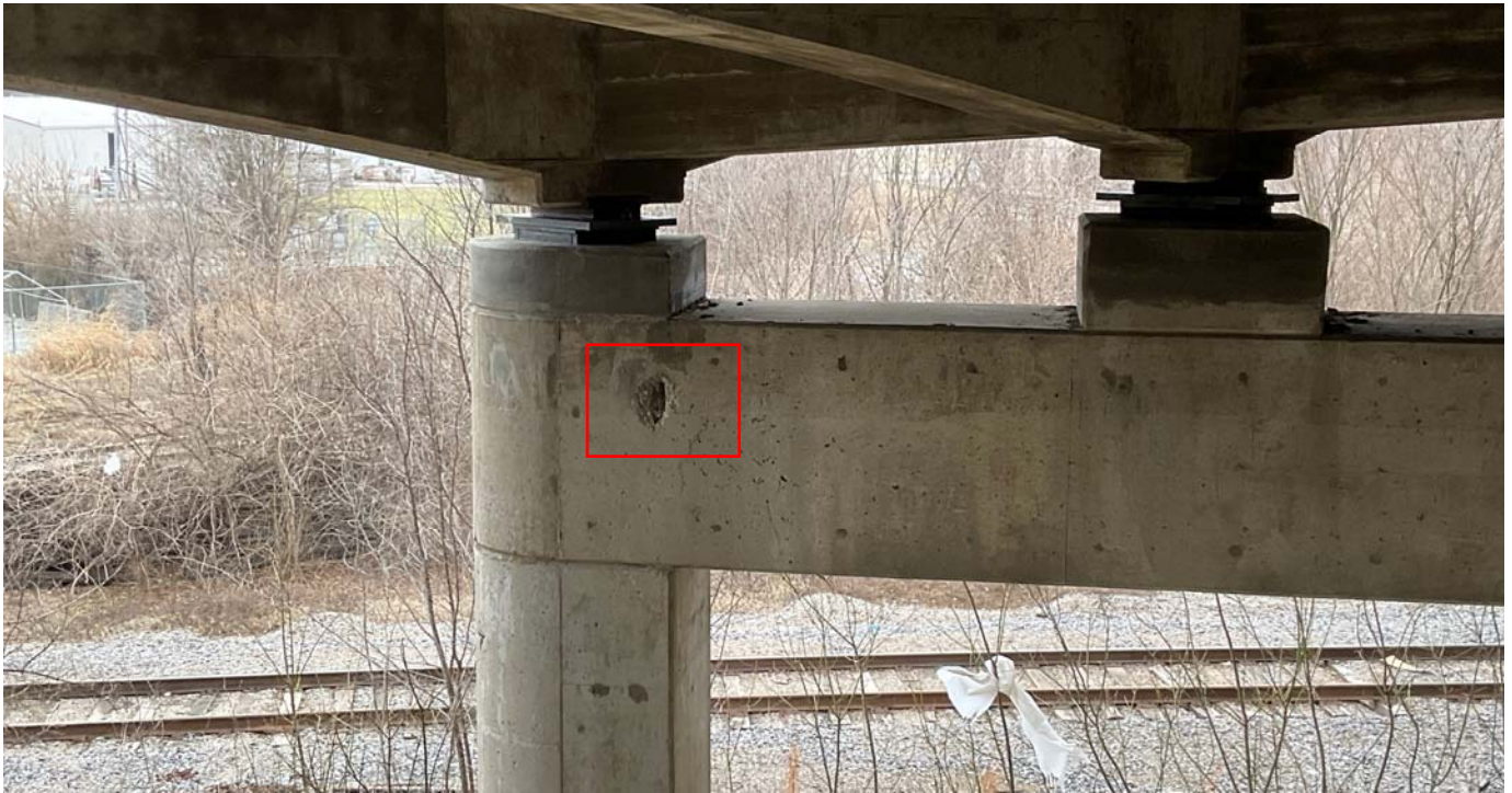
Spall - Pier 7 Span 7 under Beam 14.
