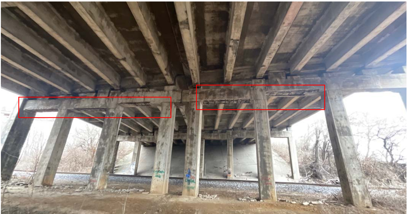
Spalling along underside of Pier 3 cap
