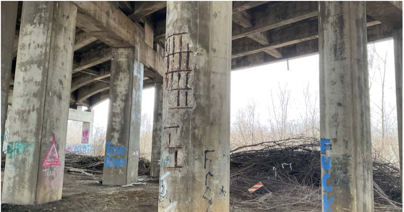
Spalling in Column 1 - Pier 4
