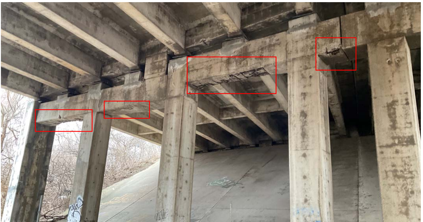
Spalling along Pier 2 cap
