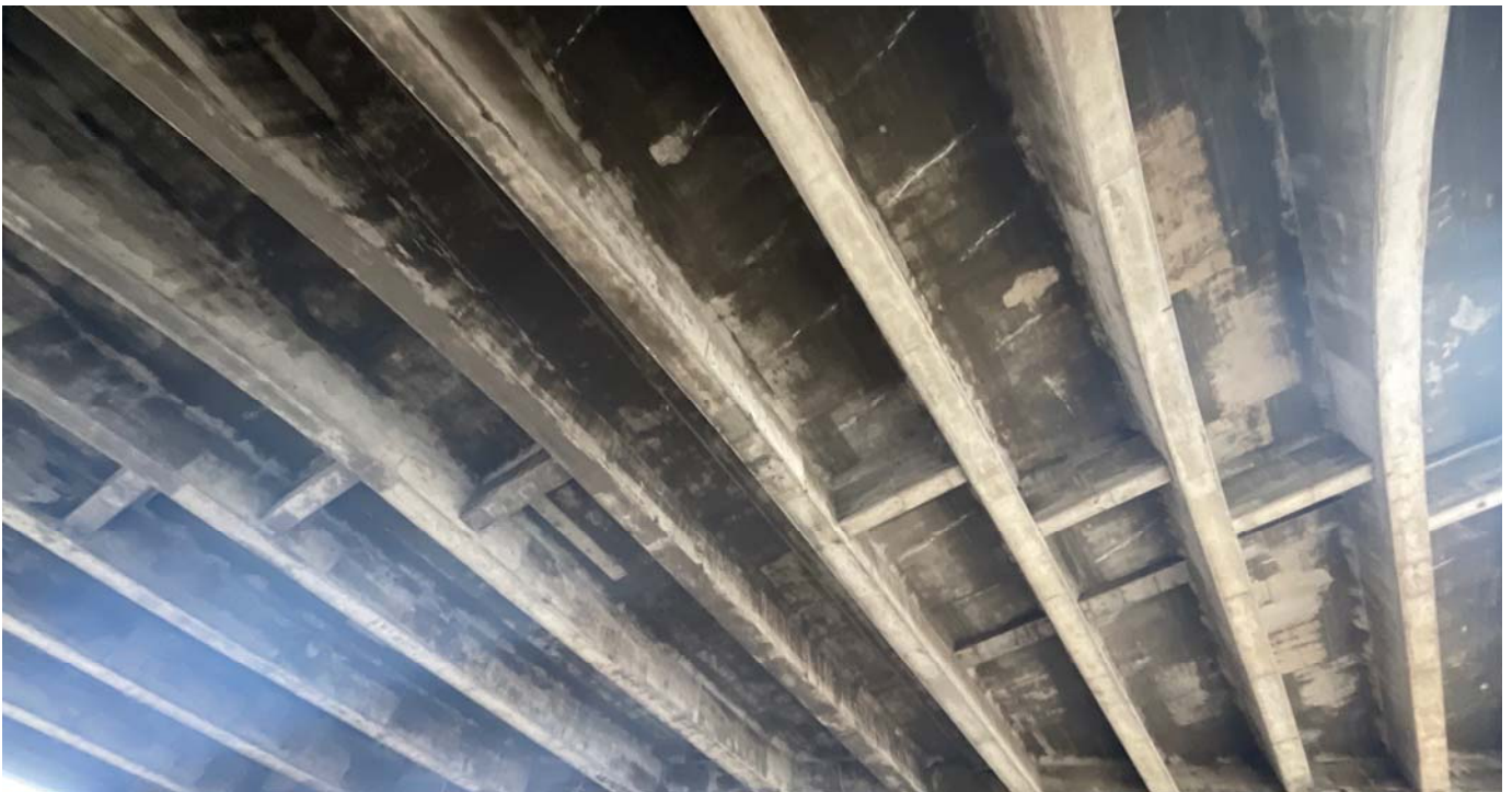
Span 5 Soffit - note cracking with efflorescence
