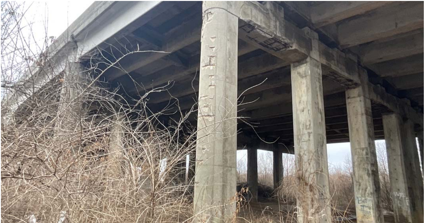
Pier 3 Column 1 spalling
