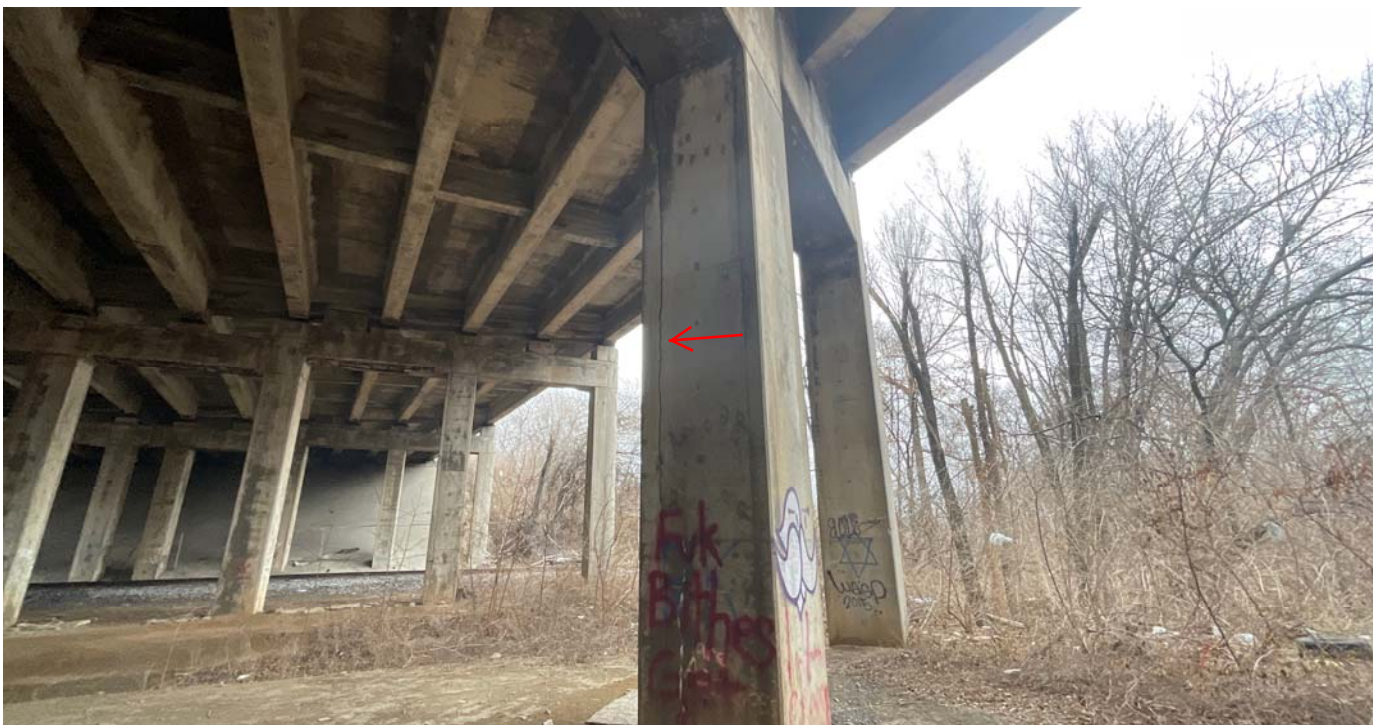
Vertical crack in Pier 5 - Column 2
