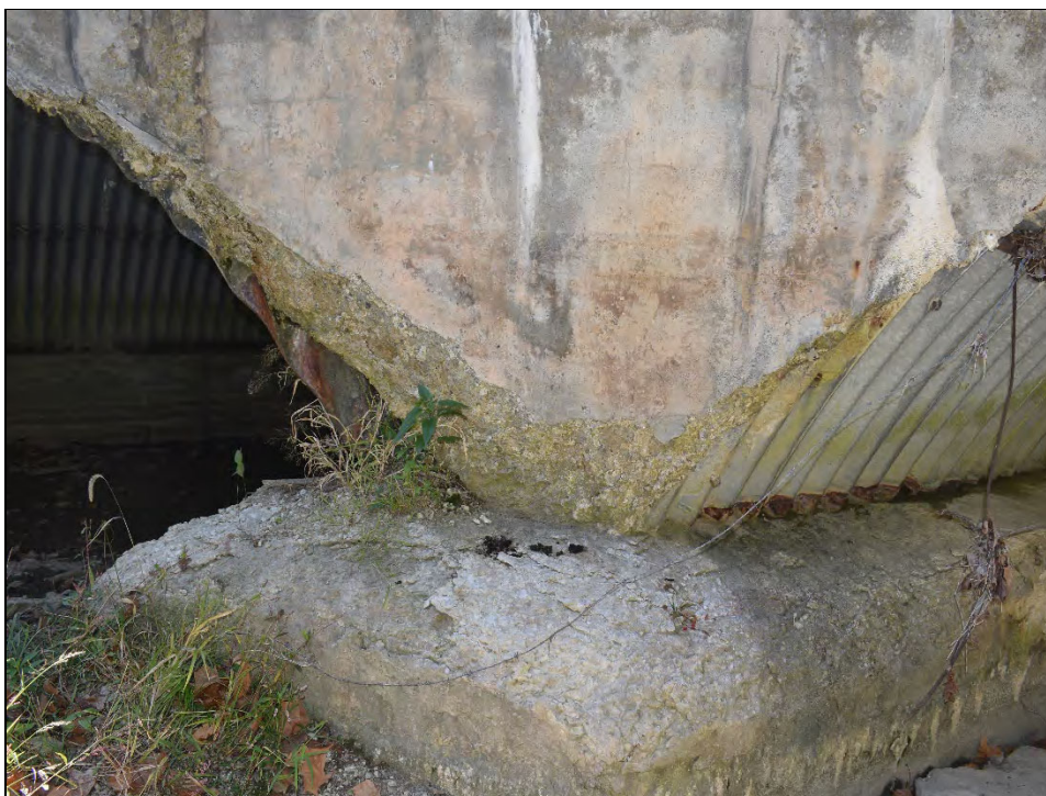
Photo 10: Evidence of spalling on footer.
