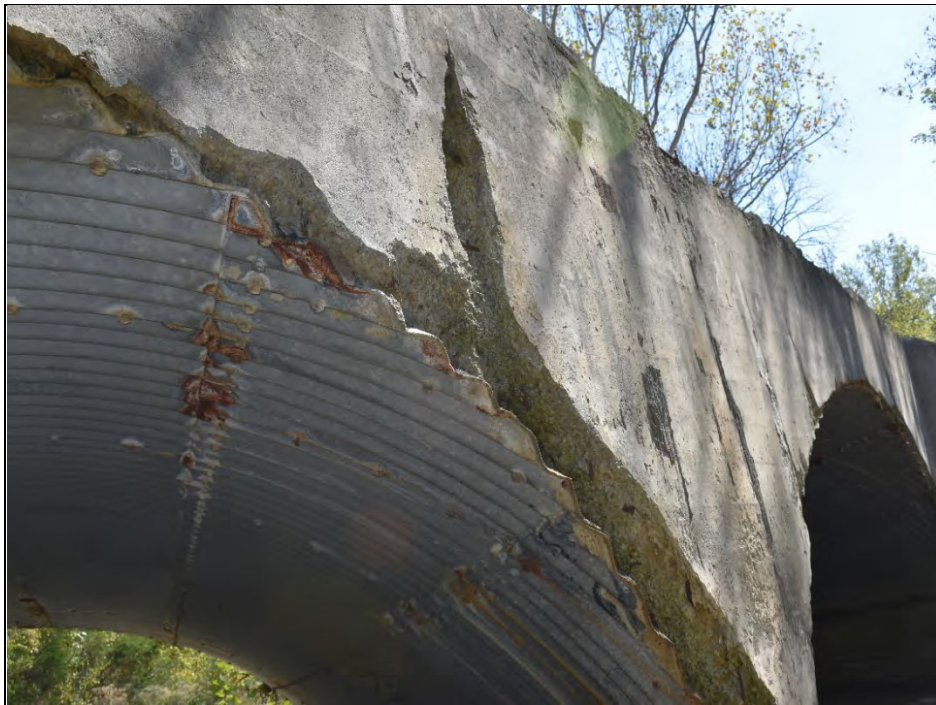
Photo 9: Evidence of spalling on the upstream curtainwall.
