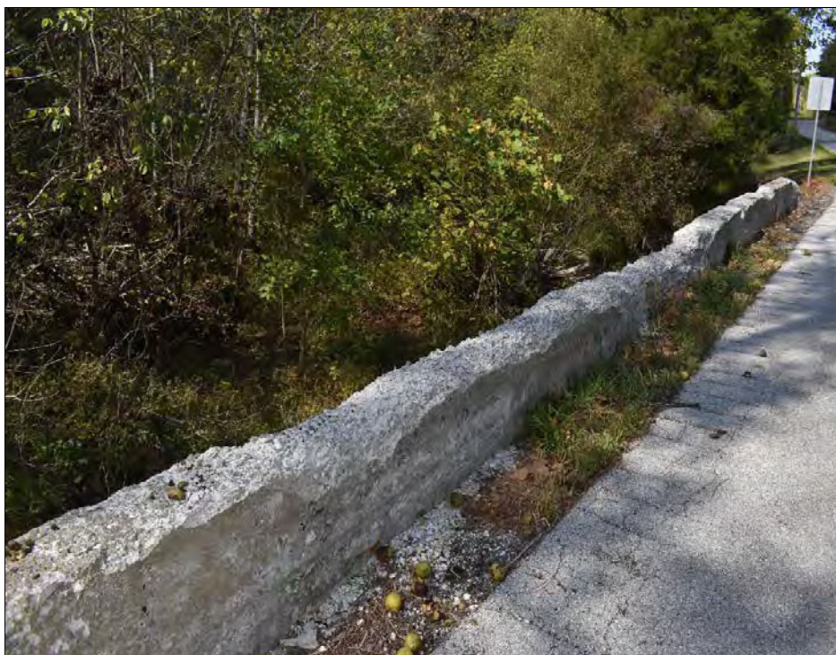
Photo 6: Evidence of deterioration on the upstream headwall.
