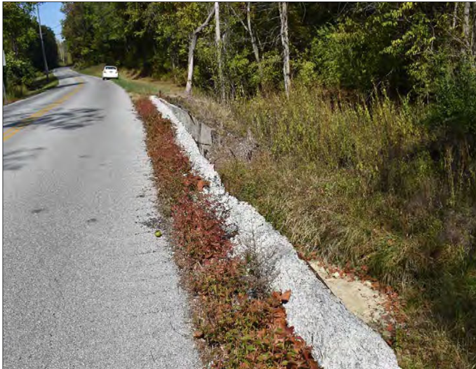
Photo 5: Evidence of deterioration on the downstream headwall.
