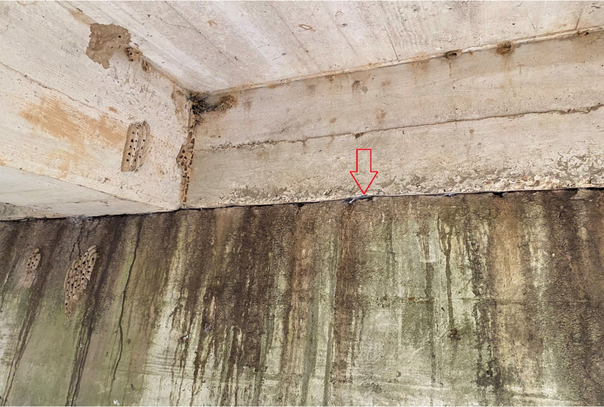
3 - IMG_2747 Abutment Joint - Facing N - Sample I-10105-1.JPG
