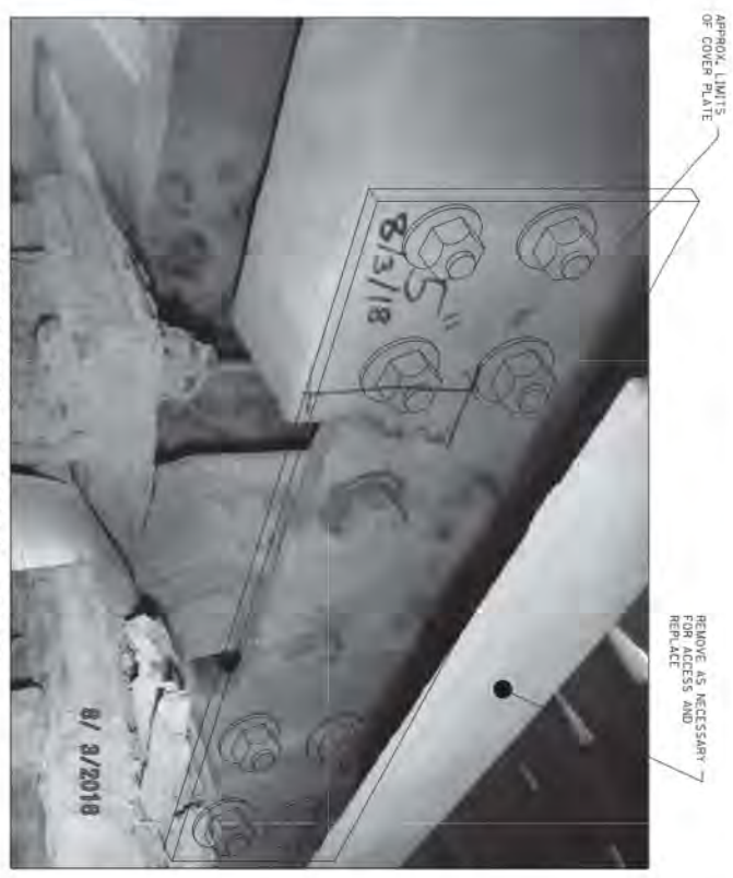
CRACKED SUPPORT CHANNEL REPAIR LOWER DECK AT PP 17, STRINGER 3
