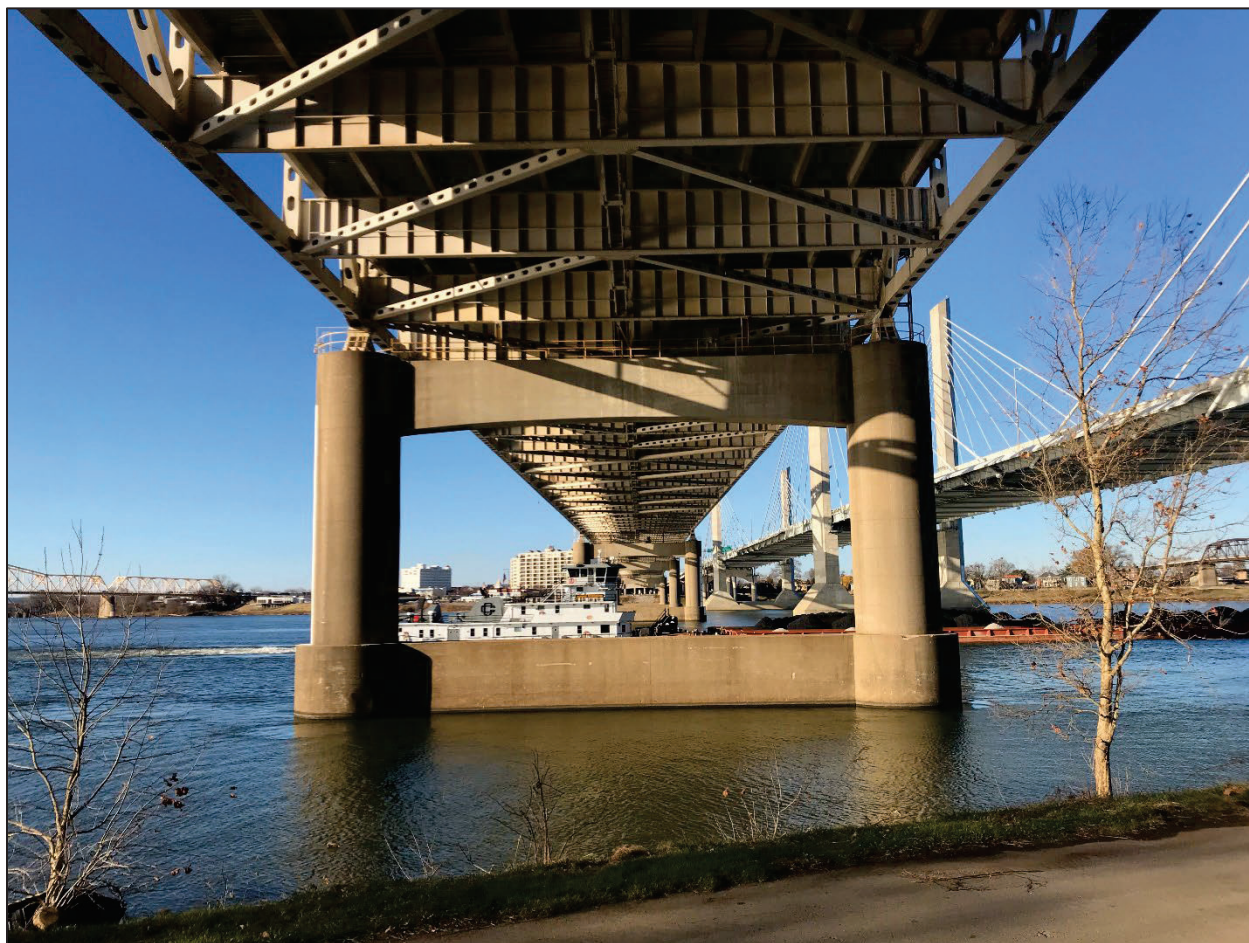
Figure 4. JFCB-722, underside of the John F. Kennedy Memorial Bridge from the Kentucky banks of the Ohio River, facing north.
