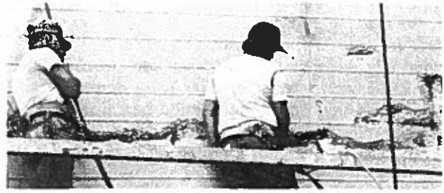
Fig. 13d. Deteriorated or redundant reinforcing bars are removed after evaluation by a structural engineer. An acetylene torch is being used to cut out the bars.
