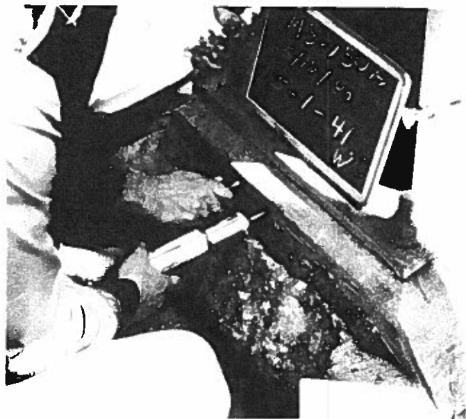
Fig. 9. Nondestructive sonic tests are one way of determining the location and soundness of internal reinforcing bars and the hardness of the concrete. There are a variety of other nondestructive tests provided by professional consultants that will help in the evaluation of the structural integrity of concrete prior to major repair work. Photo: Feld, Kaminetzky and Cohen and American Concrete Institute.
