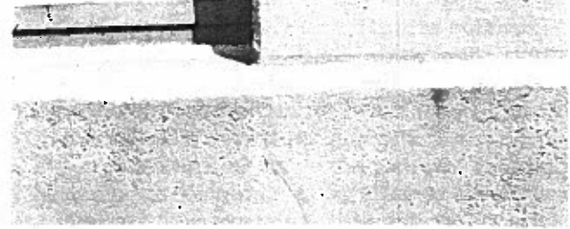
Fig. 13h. This active crack at a window sill and in the foundation wall has been filled with a flexible sealant. This area was subsequently painted with a masonry paint compatible with the sealant.
