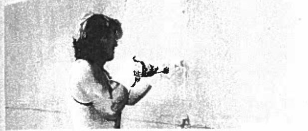
Fig. 13c. Narrow cracks often need to be widened to receive concrete patches. Here a pneumatic chisel is being used.
