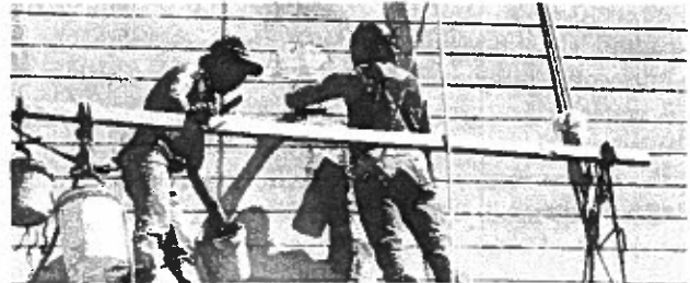
Fig. 13f. Workmen are applying patching concrete and using a trowel to form ridges to match the appearance of the historic concrete ridges that were originally created by the form boards.
