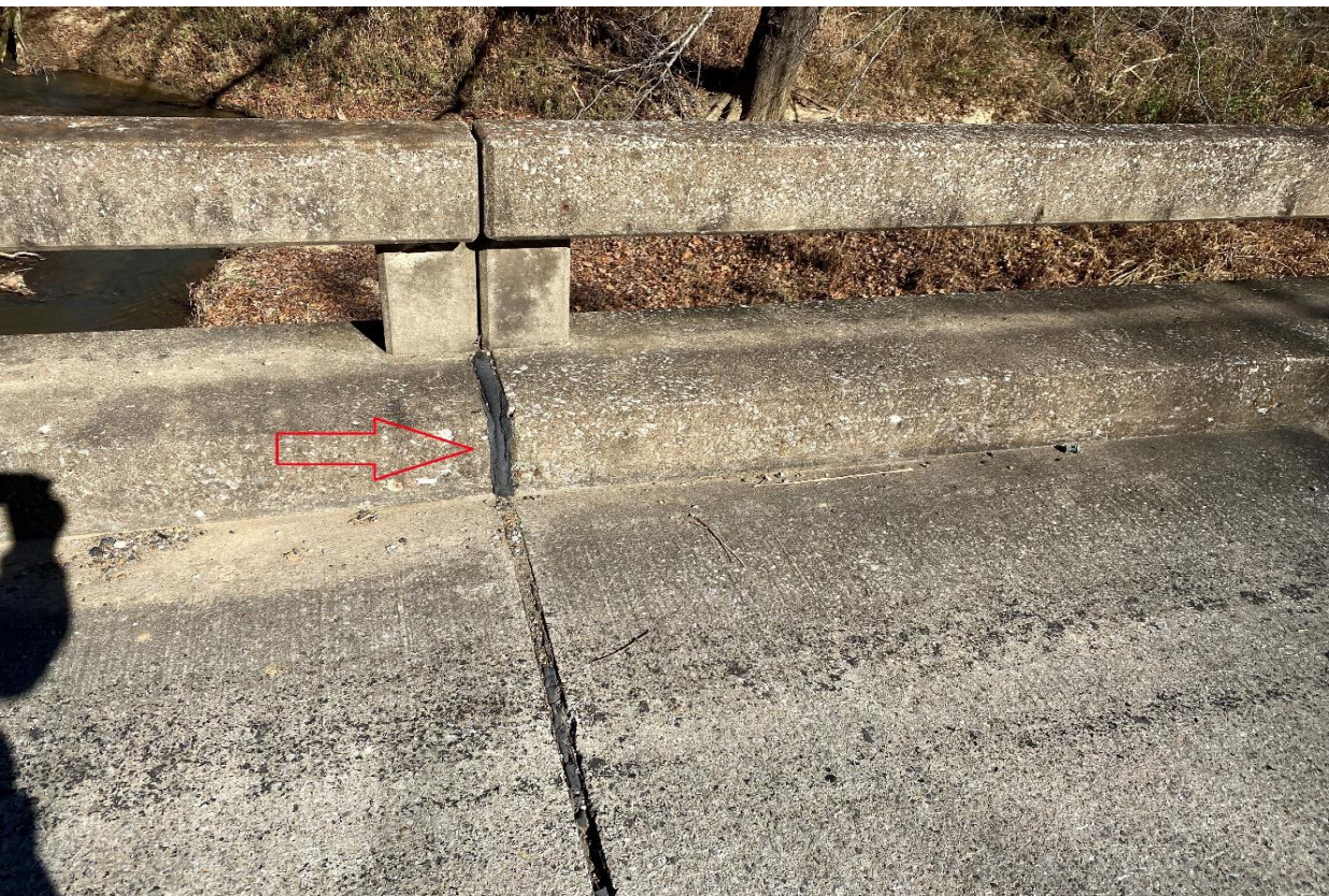
4 - IMG_2626 Joint in Bridge Surface - Facing N - Sample I-10102-1.jpg
