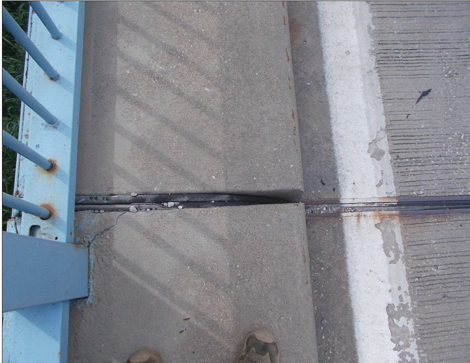
Photo 7: Example of potential bat roosting habitat if not filled with expansion joint, there were no exposed crevices like this; August 8, 2023
