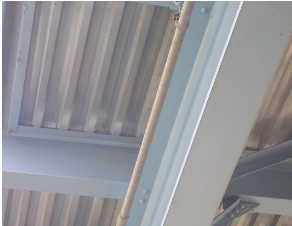
Photo 7: Example of the electrical conduit under the bridge; August 8, 2023
