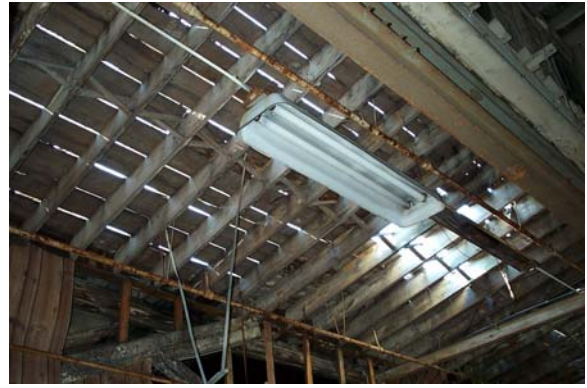
Photograph No. A-8: Daylight through the roof of Building 2.
