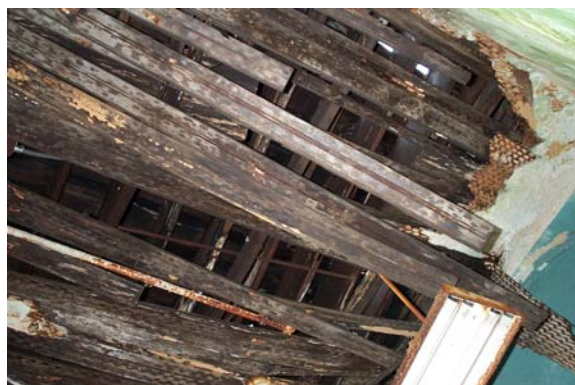
Photograph No. A-5: Ceiling collapse in Building 5.
