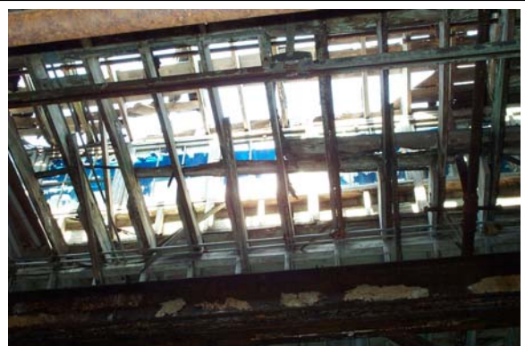
Photograph No. A-12: Deterioration of clerestory in Building 12.
