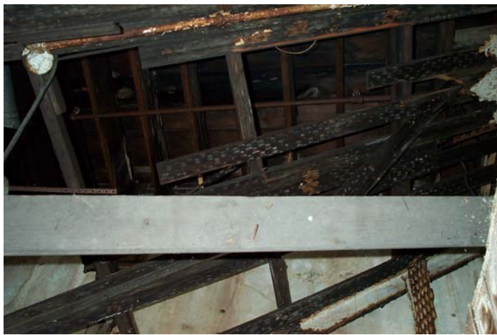
Photograph No. 6 - Failed metal lath and plaster ceiling in Building No. 5 exposing the deteriorated roof framing.
