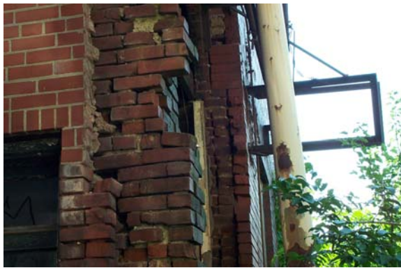
Photograph No. A-3: Severe erosion of mortar joints at corner of Building 5.
