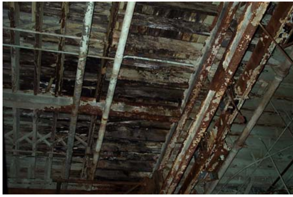
Photograph No. A-1: Decay of second floor wood framing supported by rusted steel in Building No. 2.
