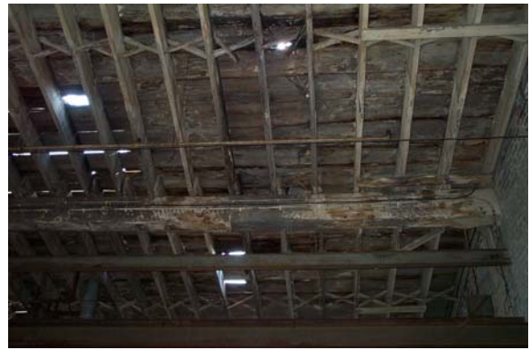
Photograph No. A-10: Deterioration of roof at Building 3.
