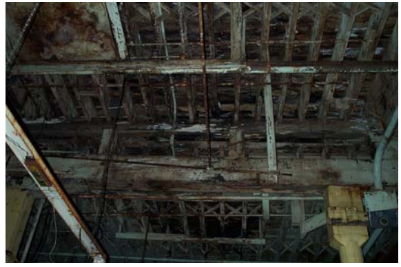
Photograph No. A-2: Decay of second floor wood framing on heavy timber supports in Building 3
