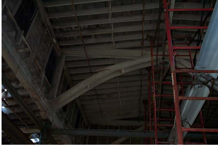
Photograph No. 5 - Failed roof truss in Building No. 2 clerestory.
