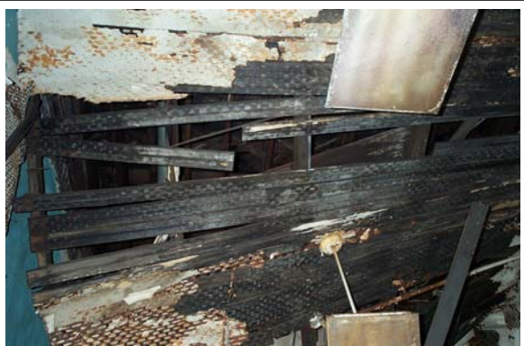
Photograph No. A-4: Ceiling collapse in Building 5
