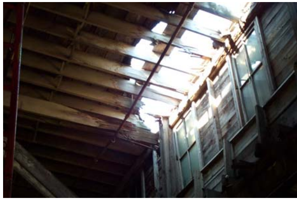
Photograph No. A-9: Daylight through roof of Building 2.
