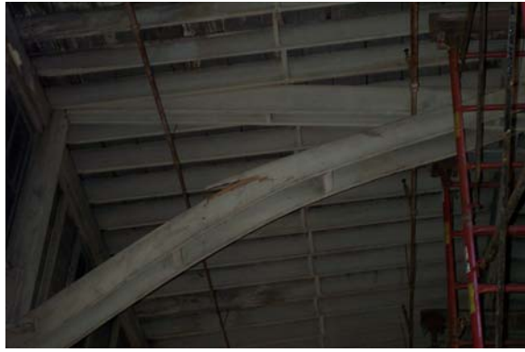
Photograph No. A-7: Failed truss in clerestory of Building No. 2
