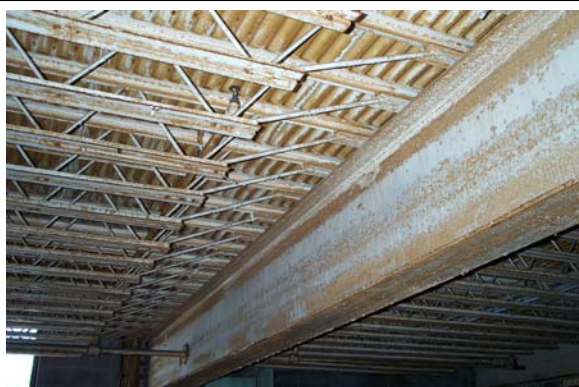
Photograph No. A-11: Mezzanine framing in Building 6 showing that it is relatively good condition.
