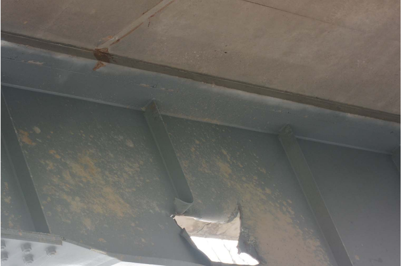
Photo 8- Girder 6 web tear
