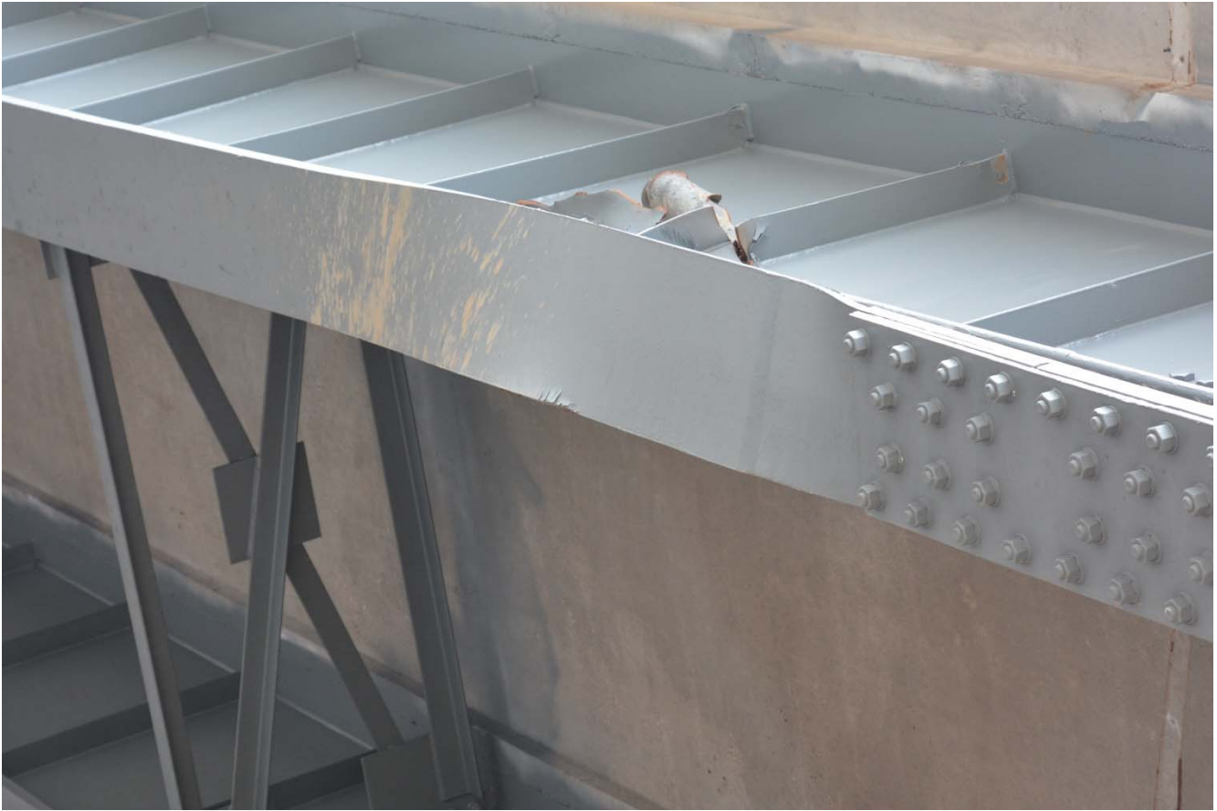
Photo 9 – Girder 6 impact area and web tear
