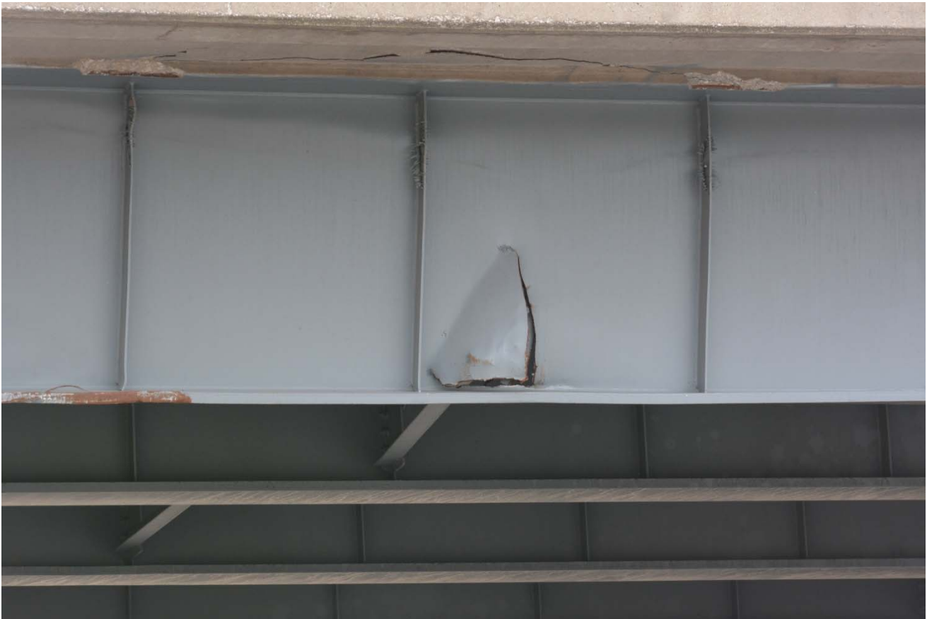
Photo 3- Girder 1 web tear
