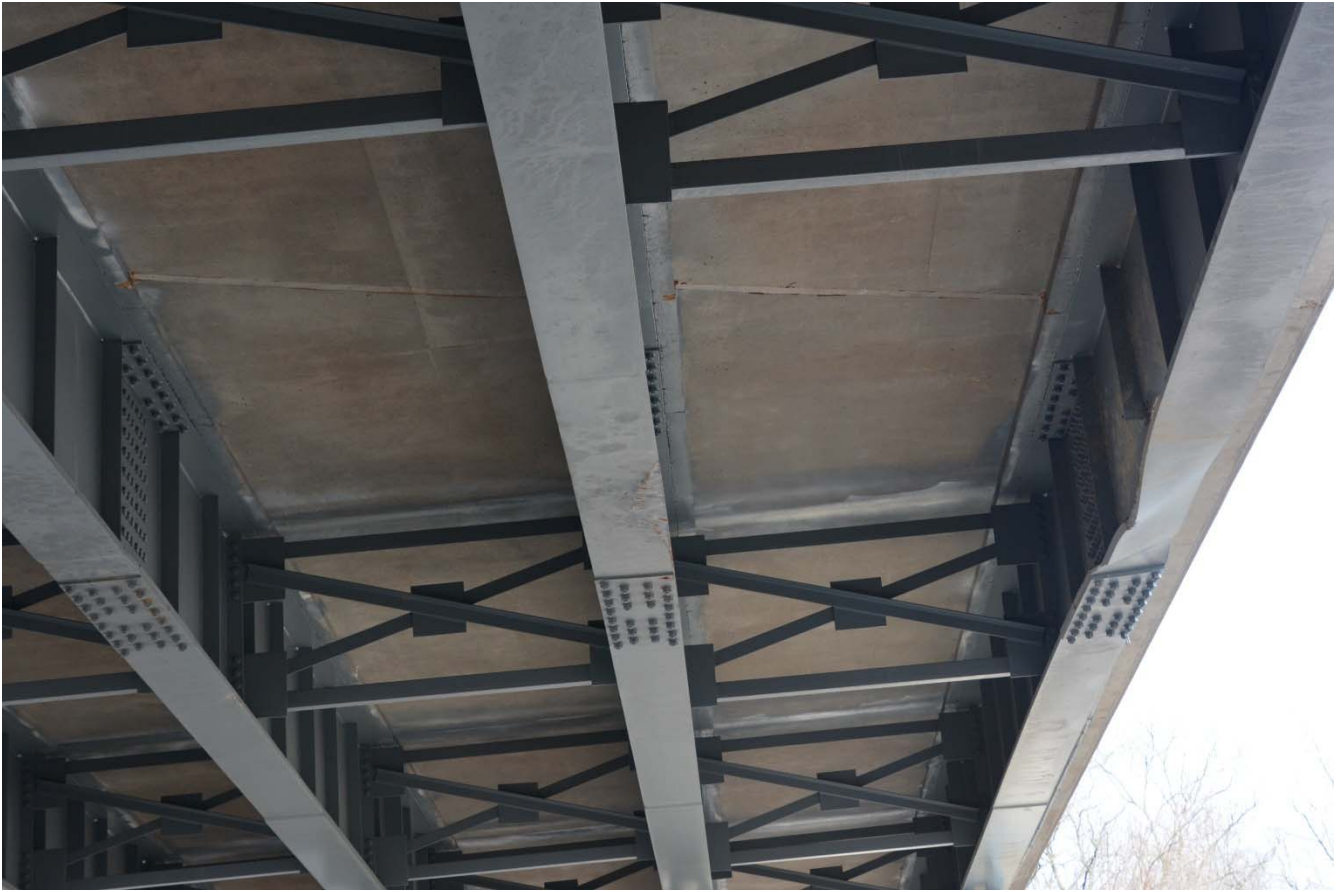
Photo 7- Girder 6 impact area
