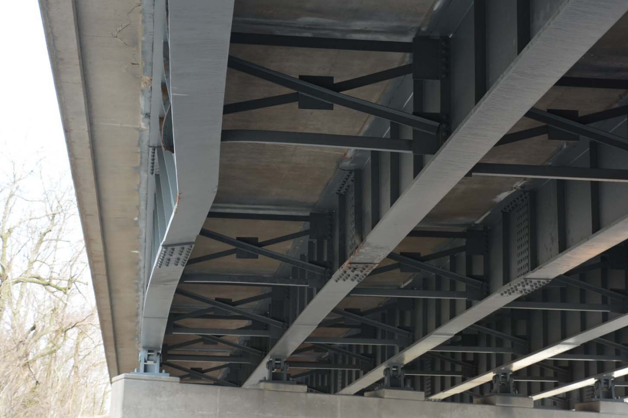
Photo 2 – Girder 1 impact area.
