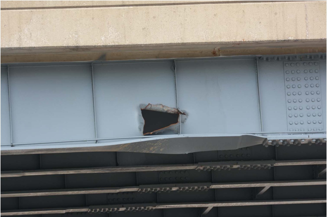
Photo 10 – Girder 6 impact area & web tear
