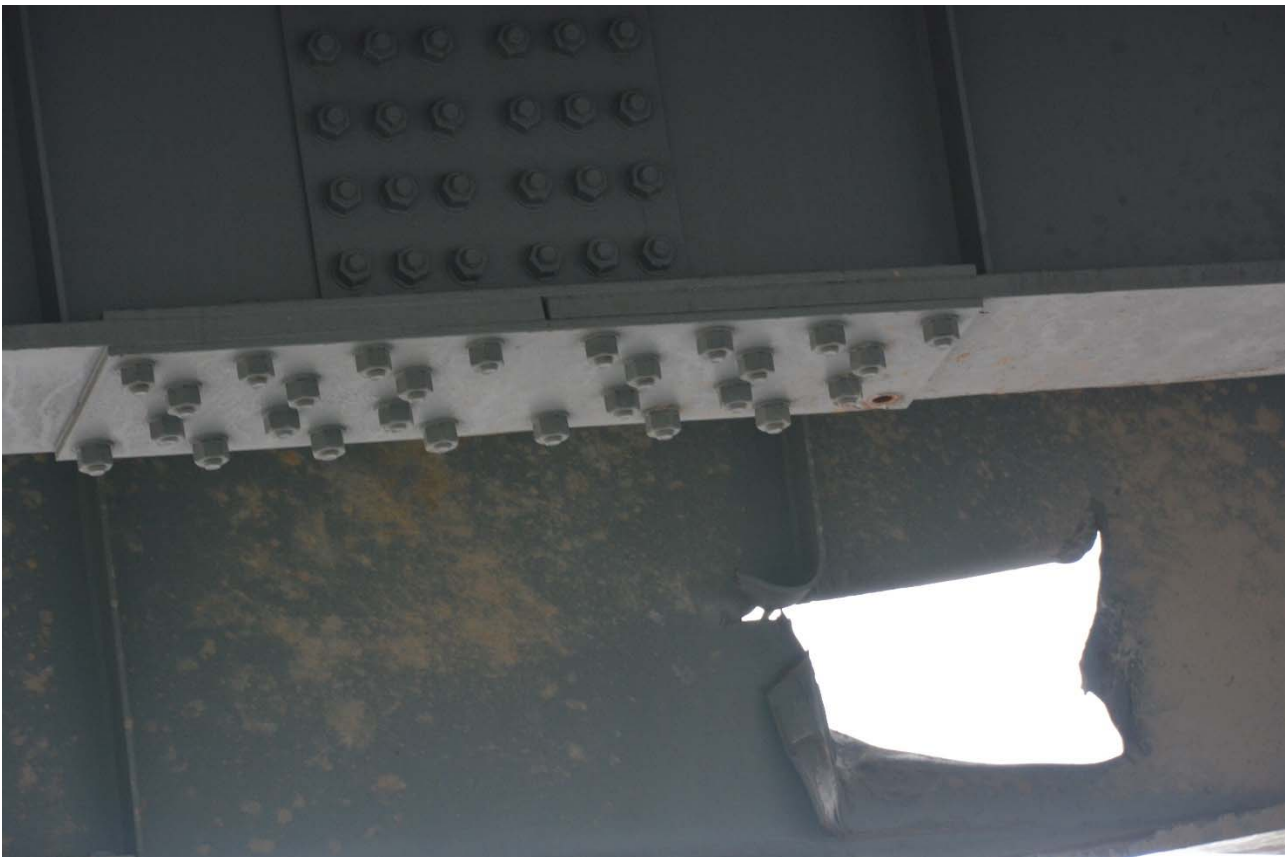
Photo 6 – Girder 5 splice plate bolt replacement. Girder 6 impact area & web tear
