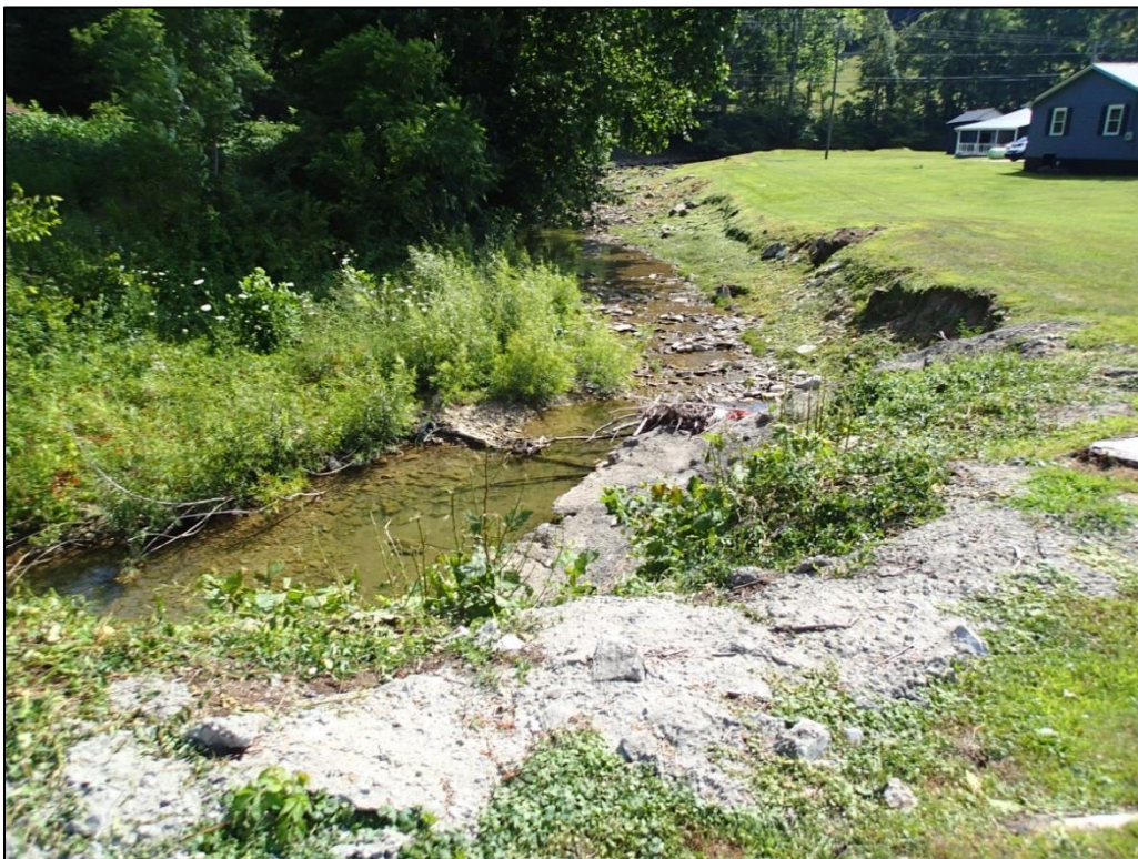
Figure 3-4. APE around Smith Creek, south of KY 474, disturbed by erosion and re-channeling efforts, looking southwest.
