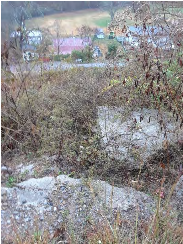
Figure 70. Post-1971 collapsing concrete slabs in southern part of survey Section 5.
