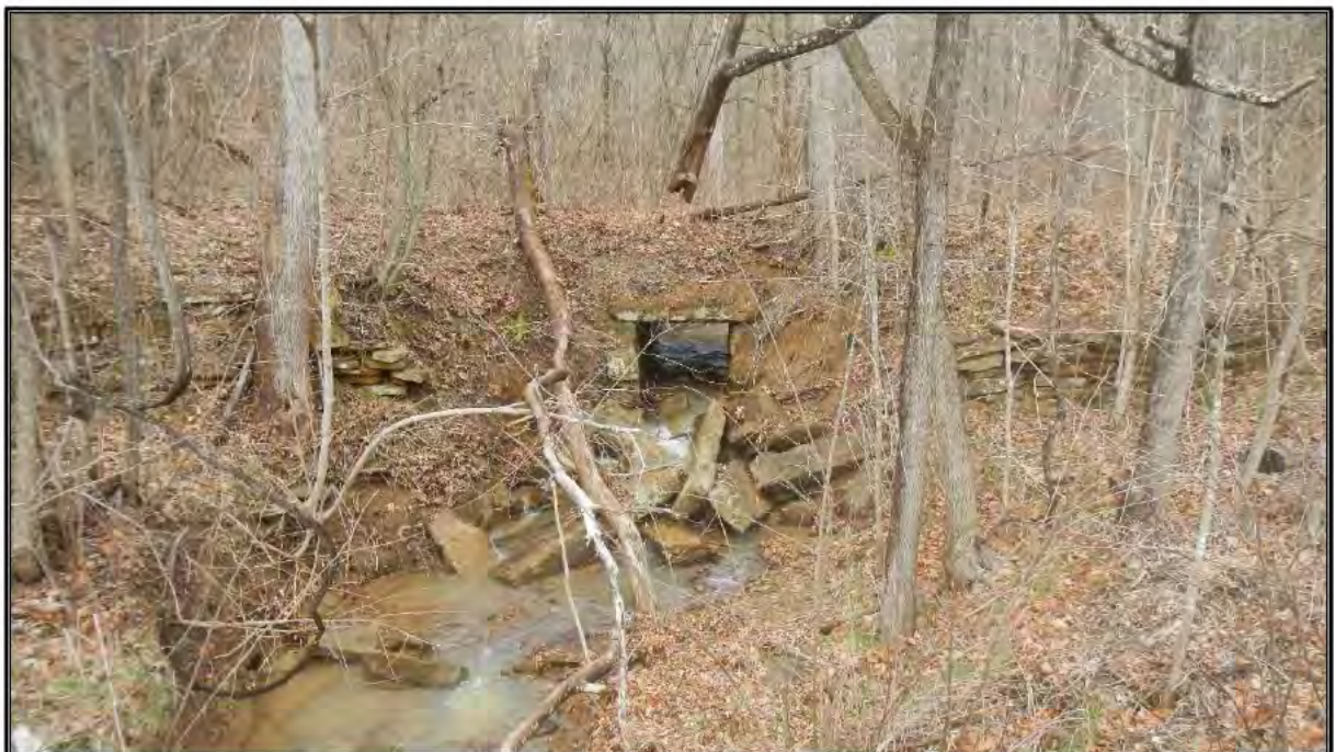
Figure 22. Overview of stone culvert and stone retaining walls along old roadway in the project area, facing north.
