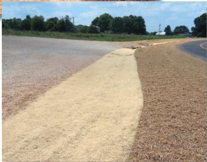
When using blankets and mats, make sure product has good soil contact throughout the ditch. Use plenty of staples to protect against surge flows during heavy rains. Blankets and mats are extremely vulnerable before seed germination, and can be dislodged by high-velocity flows if stapling is insufficient.
