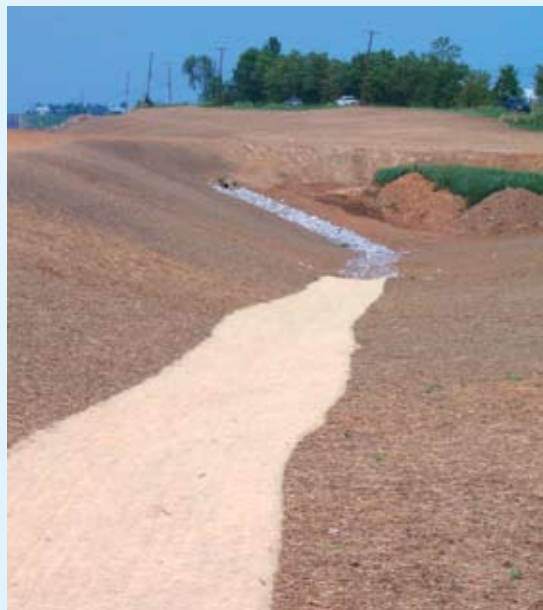
Good construction of drainage ditch, with riprap liner for steeply sloping section (background) and erosion control blanket over triple-seeding in flatter area. Ditches should be stabilized or seeded and mulched immediately after construction.
