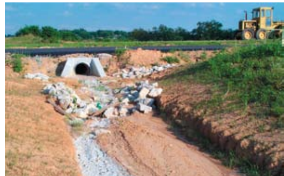
Poor placement of outlet dissipator rock; poor ditch lining (no grass, mulch, or blanket); poor slope protection.
