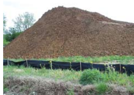
This is a good location of topsoil pile on flat, grassy area and good use of a silt fence to protect nearby creek (foreground).
