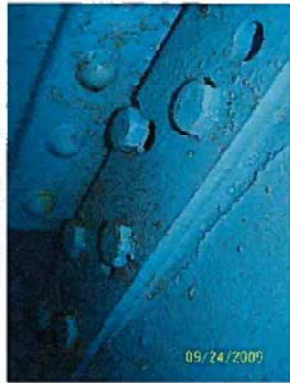
Typical view of previously rehabed diagonals. Having problems were the bolt holes had to be redrilled during the rehab.
