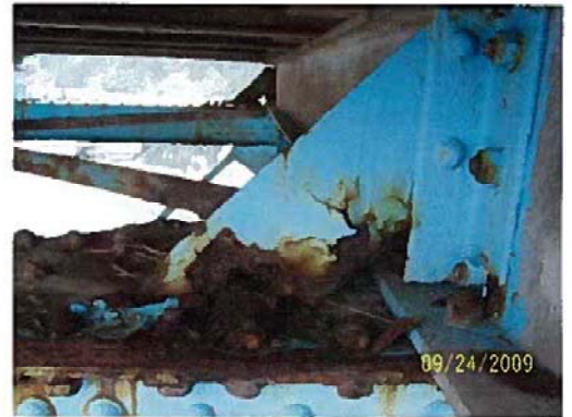
Typical view of floor beam bracing. Most have heavy section loss and some braces are completely gone or broken.
