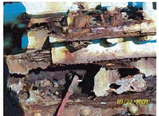
Exterior view of bearing device #2 at Pier #2. Bearing device needs to be replaced.
