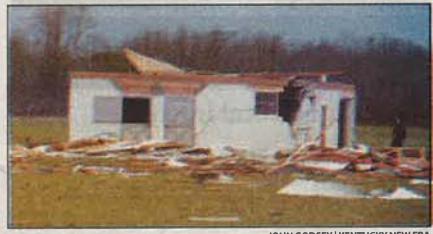
A building off Herndon Oak Grove Road was badly damaged after a storm early Wednesday.
