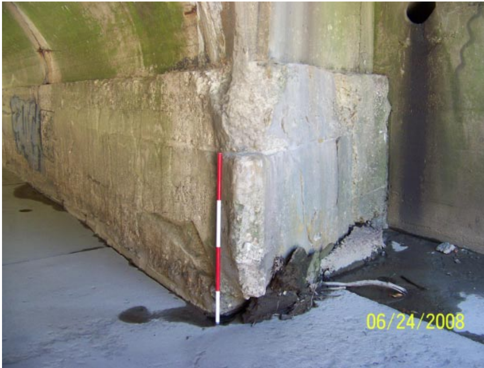
Footing of the arch at the southeast corner (US right) is deteriorated.
