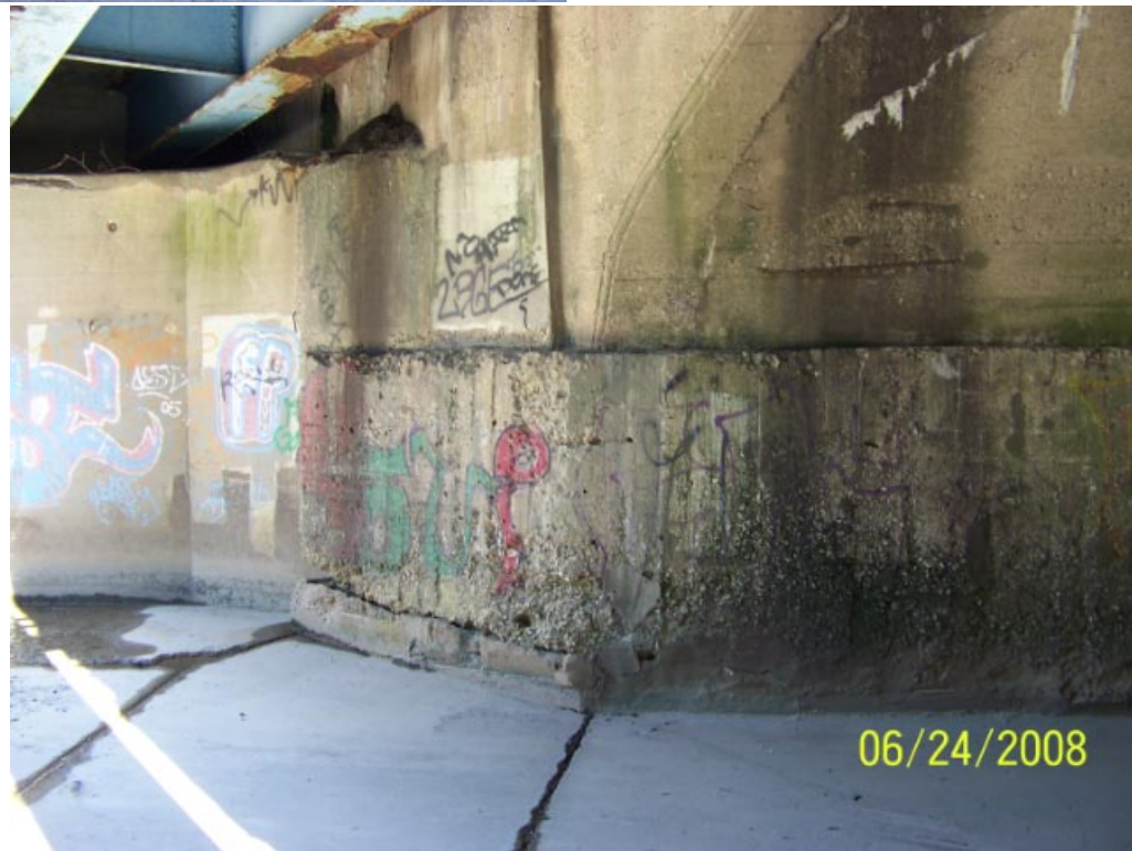
Footing of the arch at the southwest corner (US left) is deteriorated.
