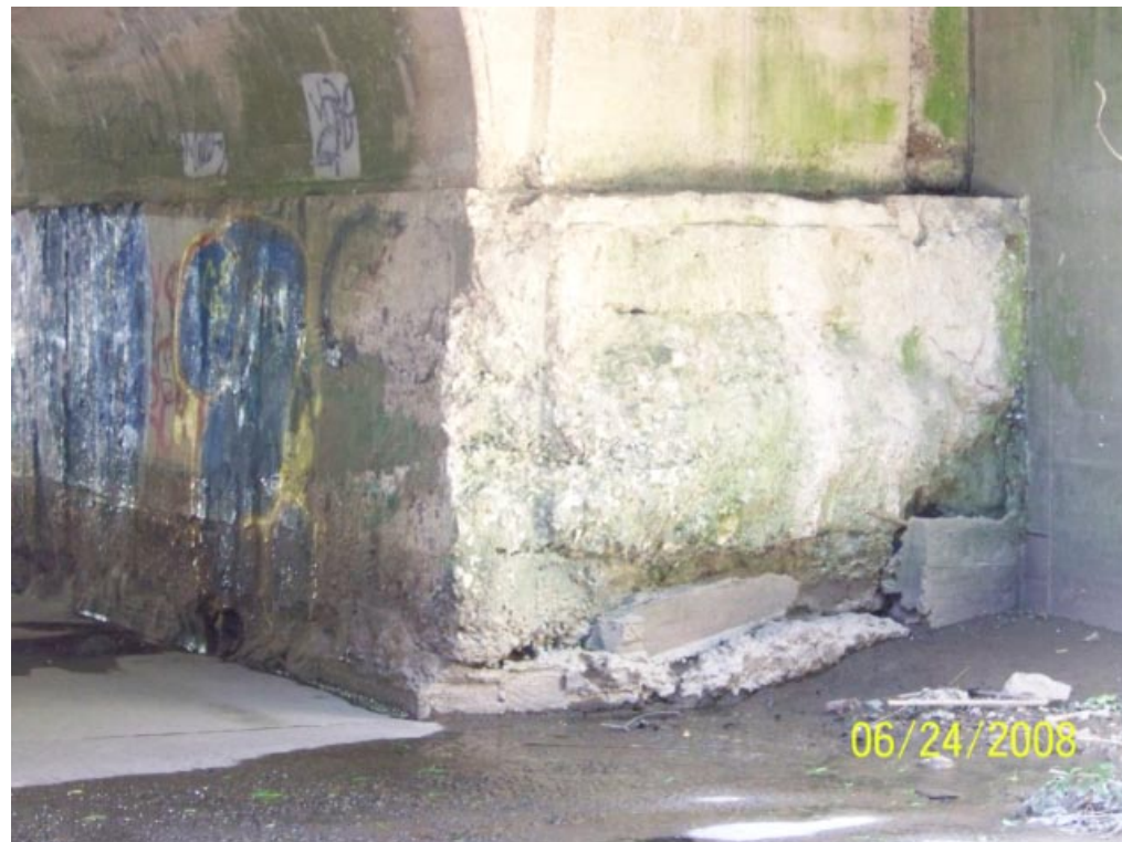
Footing of the arch at the northwest corner (DS left) is deteriorated.
