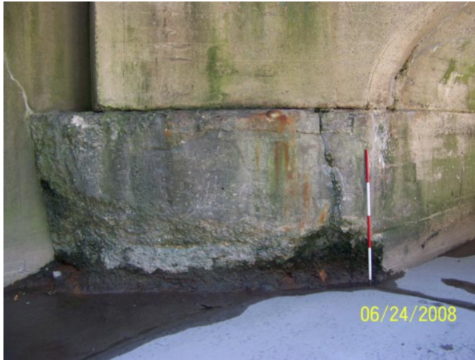
Footing of the arch at the northeast corner (DS right) is deteriorated.
