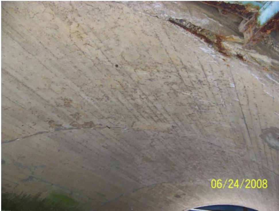
Top of the arch looking downstream. Note spall with exposed rebar near the south end.
