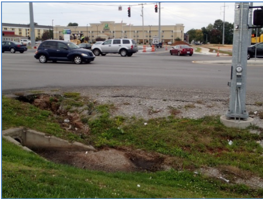
Scottsville Road at Three Springs Road. The majority of the corridor does not adequately accommodate pedestrians; for example, the push button location pictured above without sidewalks or crosswalks.
