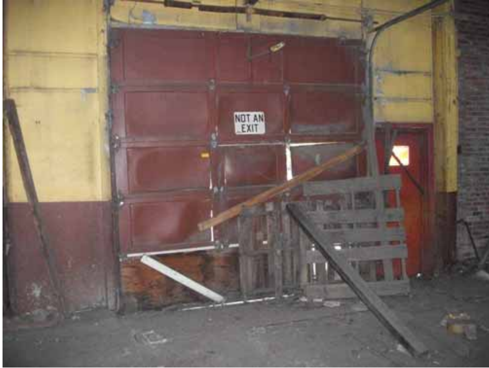
PHOTO 13: Door leading from Main Street Building out to East Main Street. Door is broken and cannot be opened in its current condition.
