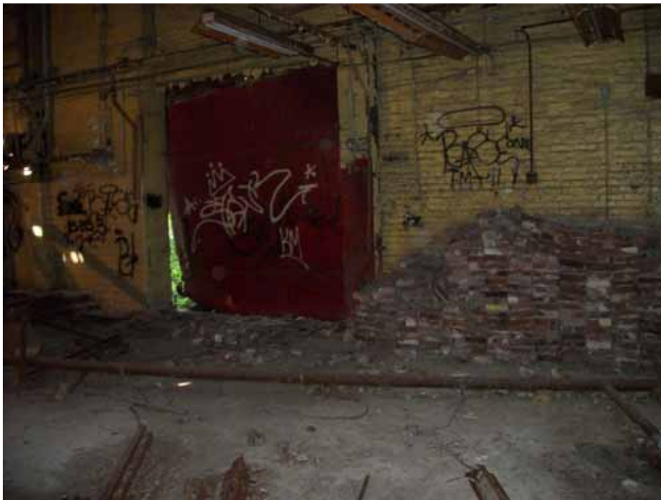
PHOTO 6: View of the same door from the inside of the East Shop, loose brick is piled against wall to right of door, floor trench in front of bricks, typical dust and debris on floor.
