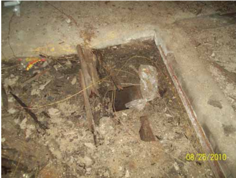
PHOTO 9: Steel plate with hole covering trench at north end of East Shop.
