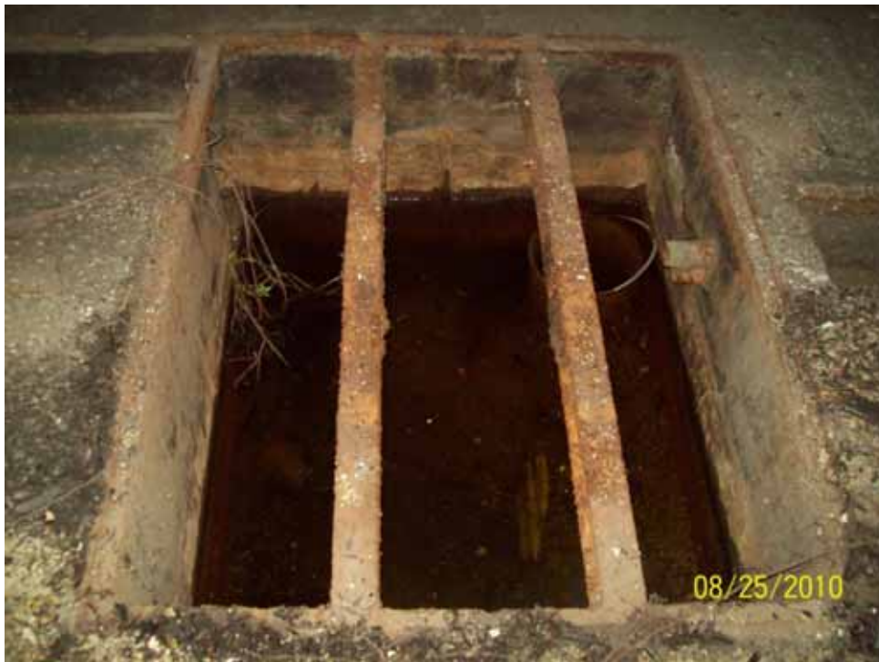
PHOTO 10: Large pit located in the center of the East Shop floor. Water is present in the pit.
