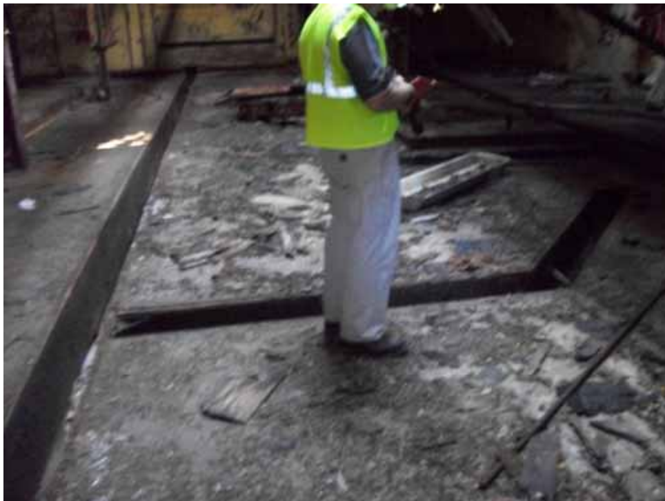
PHOTO 8: View of East Shop showing debris across floor, typical floor trenches.
