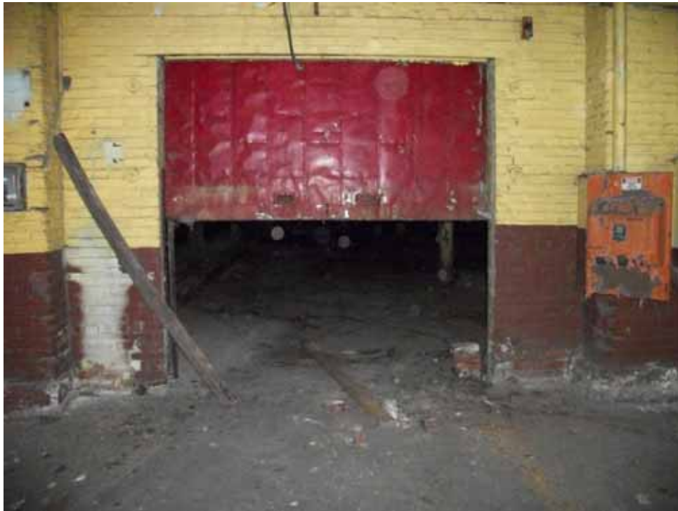
PHOTO 14: Interior door leading from Main Street Building into East Shop. Door could only be opened halfway.
