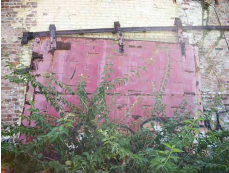
PHOTO 5: View of sliding steel door leading from court yard into East Shop. Door is broken (falling off hangers).
