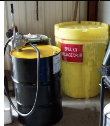
The spill kit contains protective equipment and absorbent materials for emergency use. Locate spill kits near where materials are stored and used.
