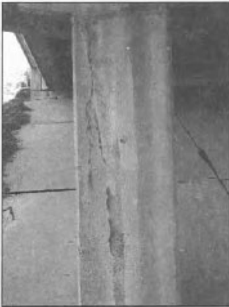
Figure B-12— 3 / 16 -in. Width Vertical Crack in Left Column of Pier 4
