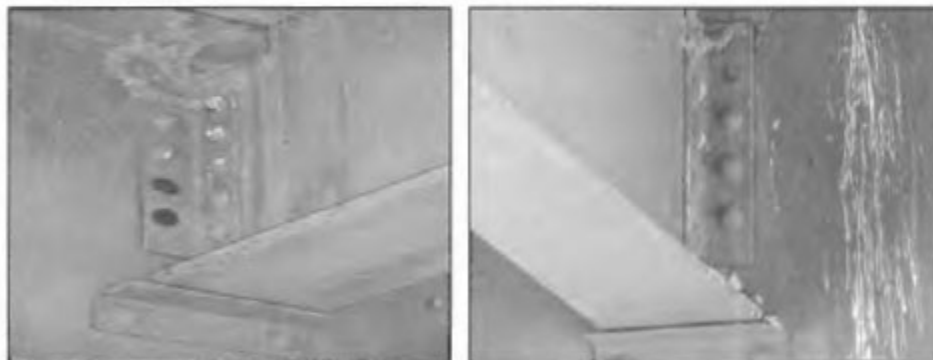
Figure B-18--Missing and Broken Fasteners at Stringer-to-Floor Beam Connections
