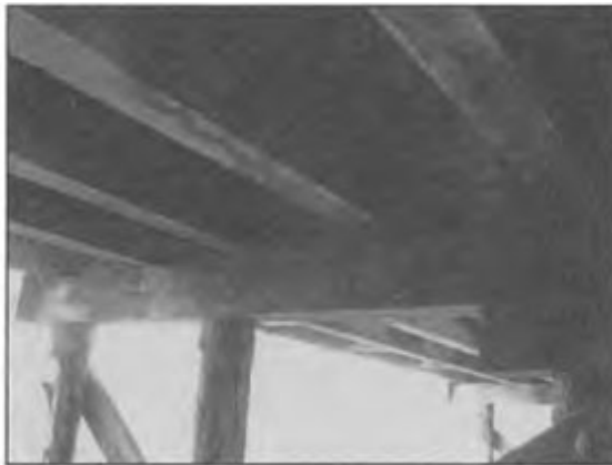
Figure B-3-1-in. Deep Check in Bent Cap at Bent 2
