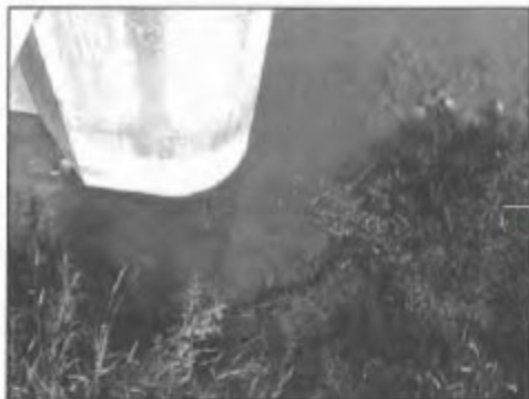
Figure B-19--Scour Hole at the Upstream End of the Pier Wall
