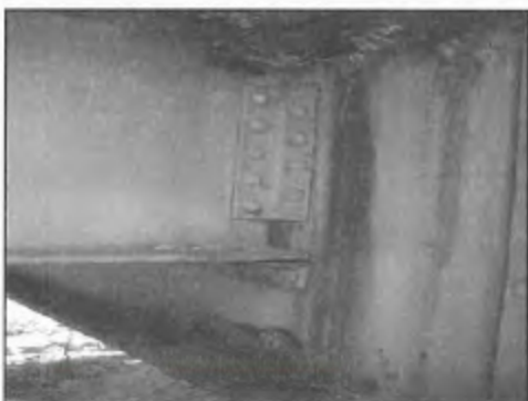
Figure B-17—Corrosion at Floor Beam Ends
