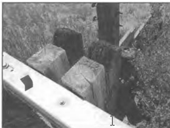
Figure B-5-Decay in Timber Rail Posts
